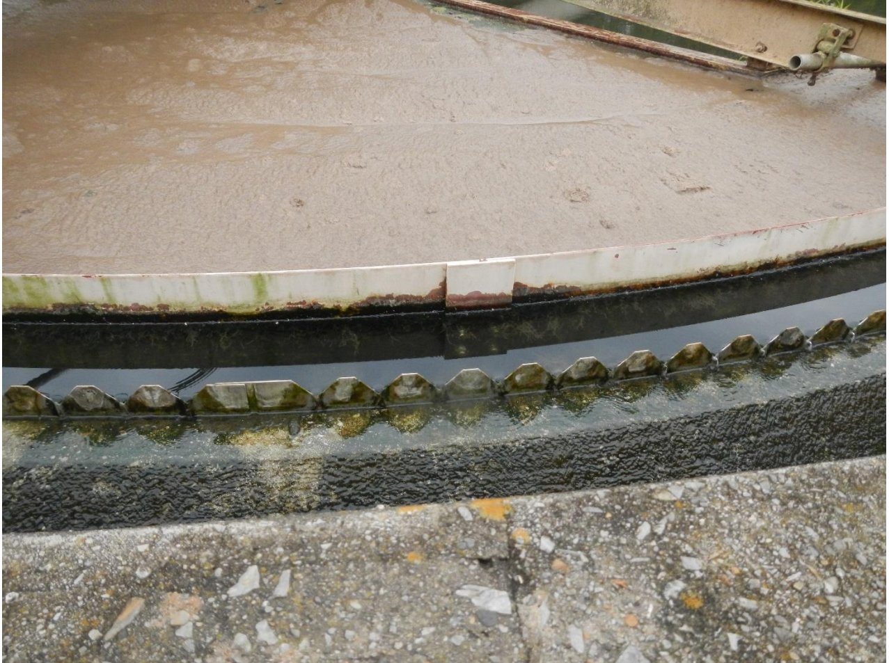
Figure 5. Excessive foaming in Clarifier.
