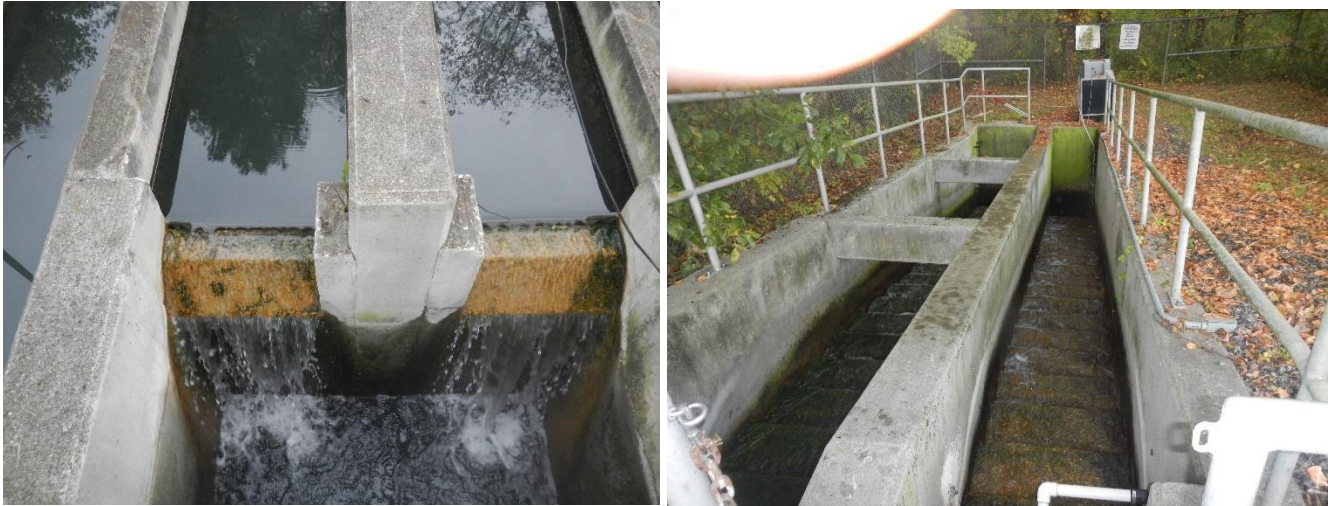
Figure 6. Left, effluent discharged from CCC. Right, step aeration.
