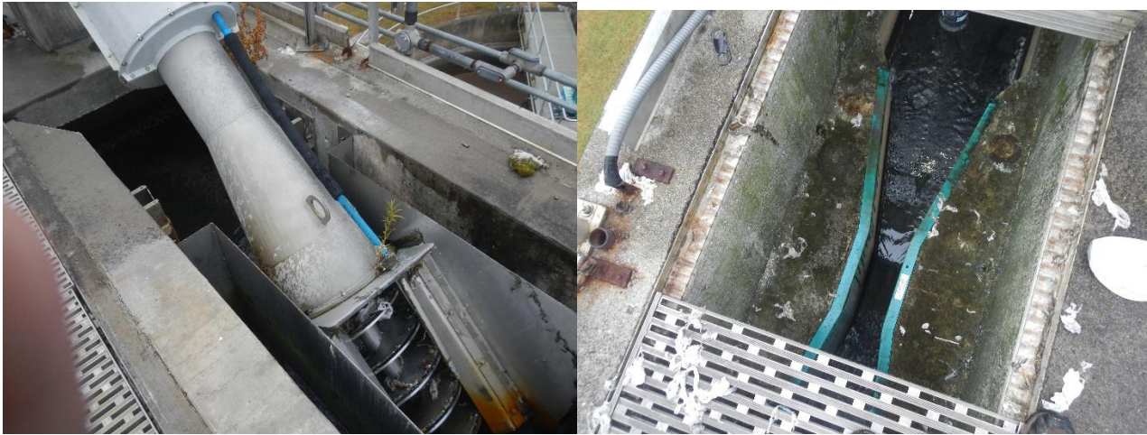
Figure3. Headworks grit removal unit and influent Parshall flume.
