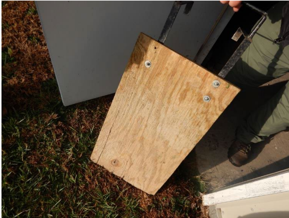
Photograph 11. (DSCN0052) View of a wooden board that is placed over raceway outlets during quiescent zone cleaning.
