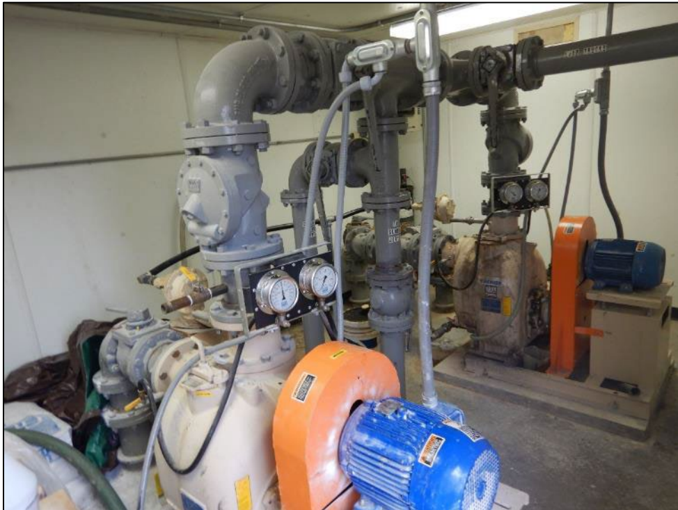
Photograph 20. (DSCN0067) View of the two pumps and associated piping and valves inside the pump house. The pumps, piping, and valves were configured such that sludge from the clarifier can be discharged to the sludge holding tank or to Spring Run via Outlet 011.
