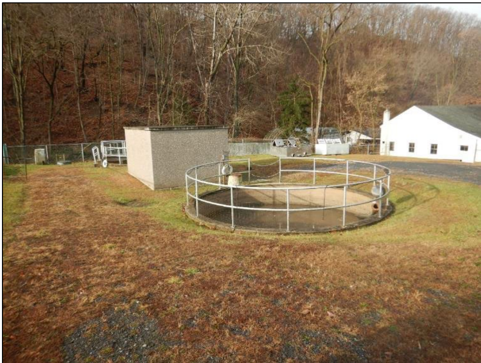
Photograph 18. (DSCN0056) View of the sludge holding tank and pump house. The clarifier is behind the pump house obscured from view.
