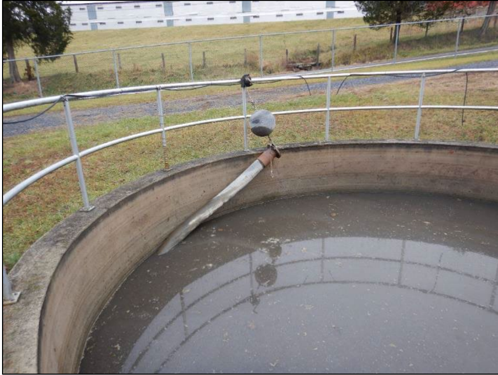
Photograph 19. (DSCN0088) View inside the sludge holding tank. Facility representatives stated the decanter flows to the clarifier.
