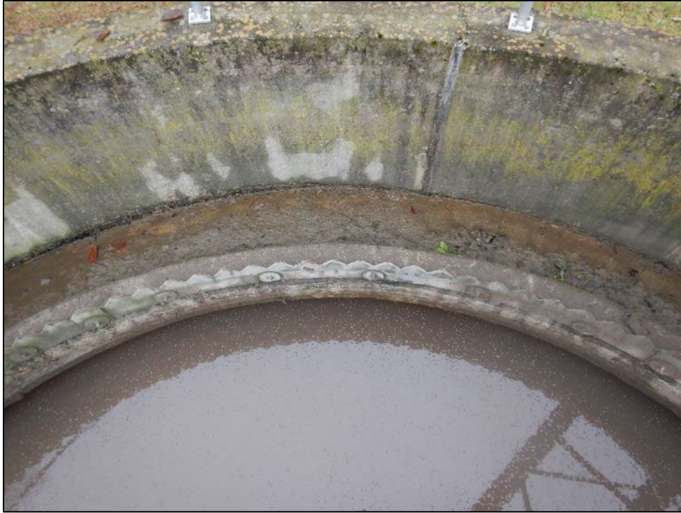
Photograph 17. (DSCN0064) Additional view inside clarifier. The clarifier contained sludge and dead fish at the time of the inspection; Facility representatives stated that the clarifier is not cleaned frequently.
