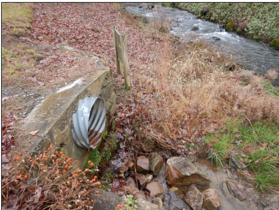
Photograph 32. (DSCN0111) Additional view of Outlet 010.
