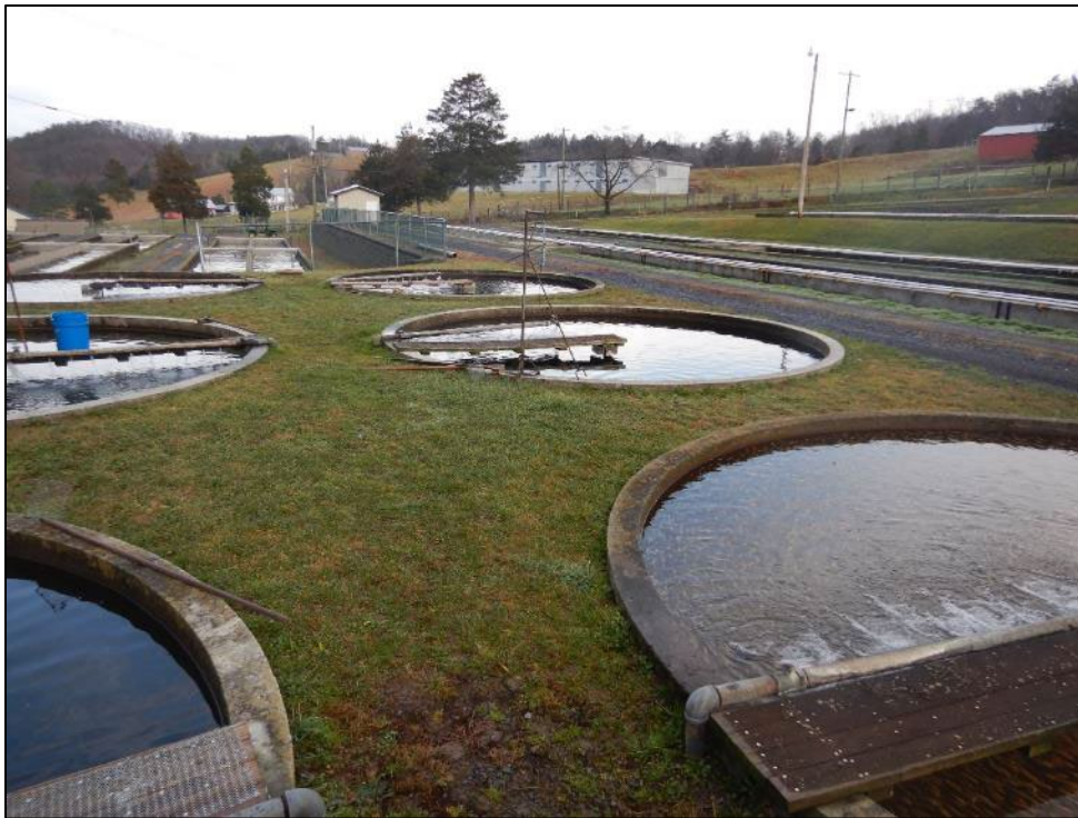
Photograph 2. (DSCN0033) View of the holding pools. Water that passes through these pools is discharged untreated to Spring Run via Outlet 008.
