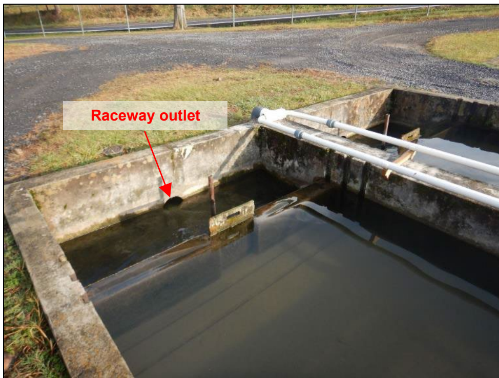
Photograph 10. (DSCN0051) View of the northern end of one of the middle raceways. During cleaning of the quiescent zones, the raceway outlets are covered so that only wastewater from the quiescent zones is conveyed to the clarifier.
