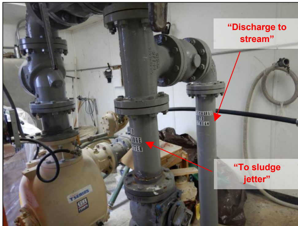
Photograph 23. (DSCN0074) View of piping associated with the sludge pumps. The pumps, piping, and valves were configured such that sludge from the clarifier can be discharged to the sludge holding tank or to Spring Run via Outlet 011.
