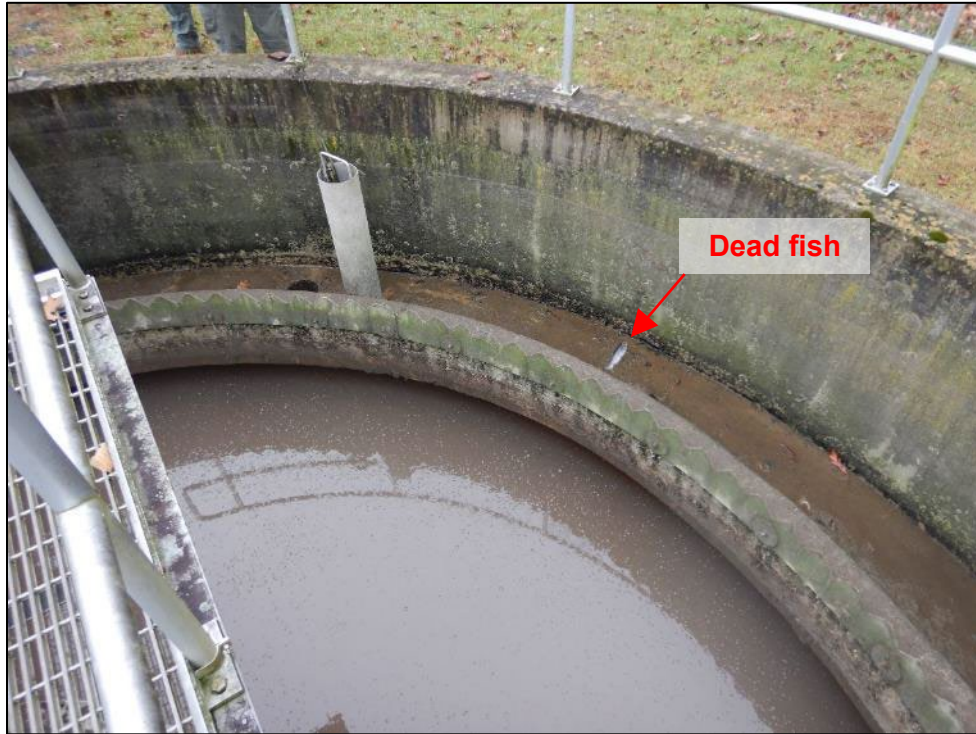
Photograph 15. (DSCN0065) Additional view inside clarifier. The clarifier contained sludge and dead fish at the time of the inspection; Facility representatives stated that the clarifier is not cleaned frequently.
