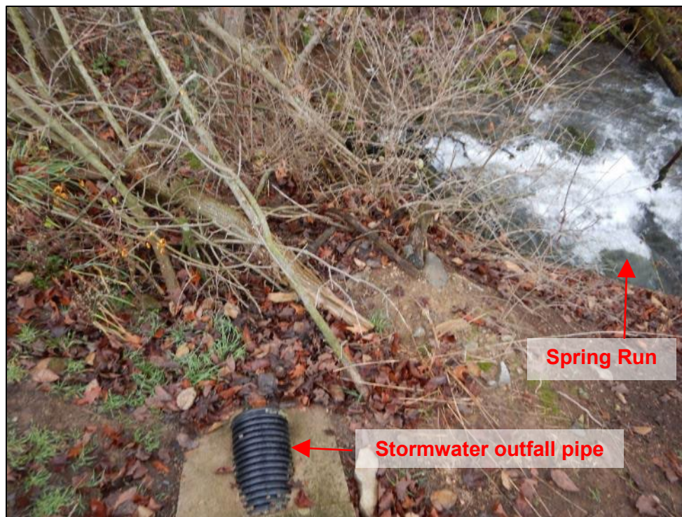
Photograph 34. (DSCN0095) View of the unpermitted outfall pipe near Outlet 011.
