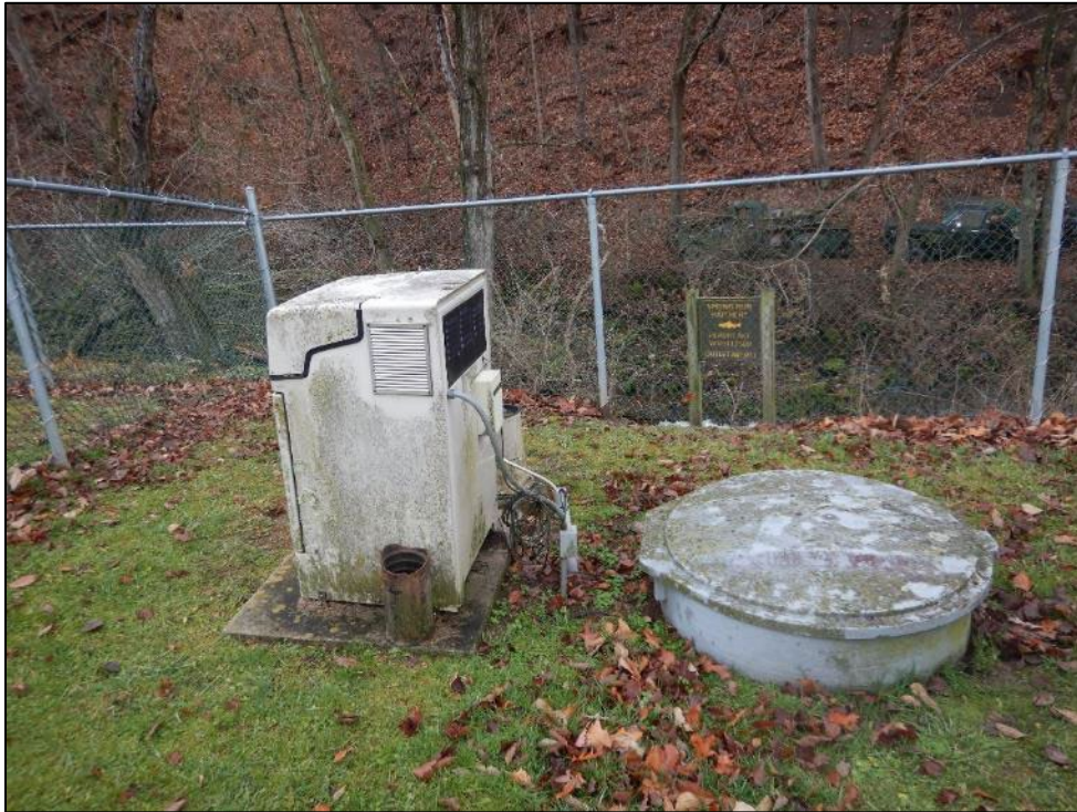
Photograph 25. (DSCN0089). View of the automatic composite sampler and flume vault for Outlet 011.
