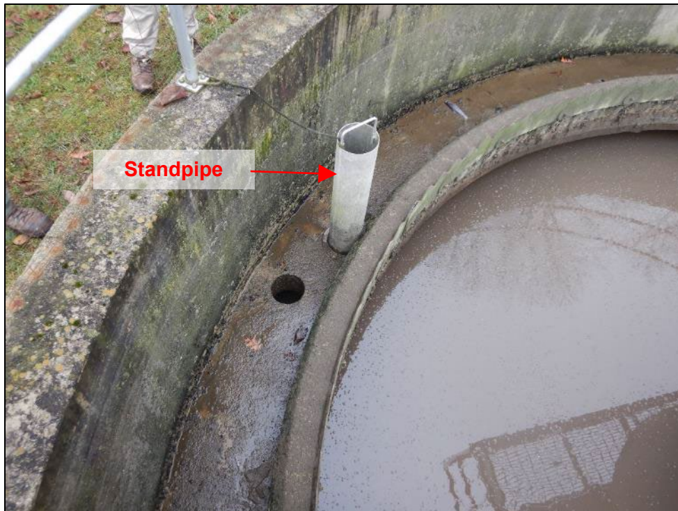
Photograph 14. (DSCN0061) View inside the clarifier. A standpipe had been installed to provide additional hydraulic capacity. Facility representative stated a standpipe had been installed in the clarifier to increase the hydraulic capacity of the clarifier but that only the decanter is used to discharge from the clarifier to Outlet 011. Facility representatives stated the opening near the standpipe flows back into the clarifier.
