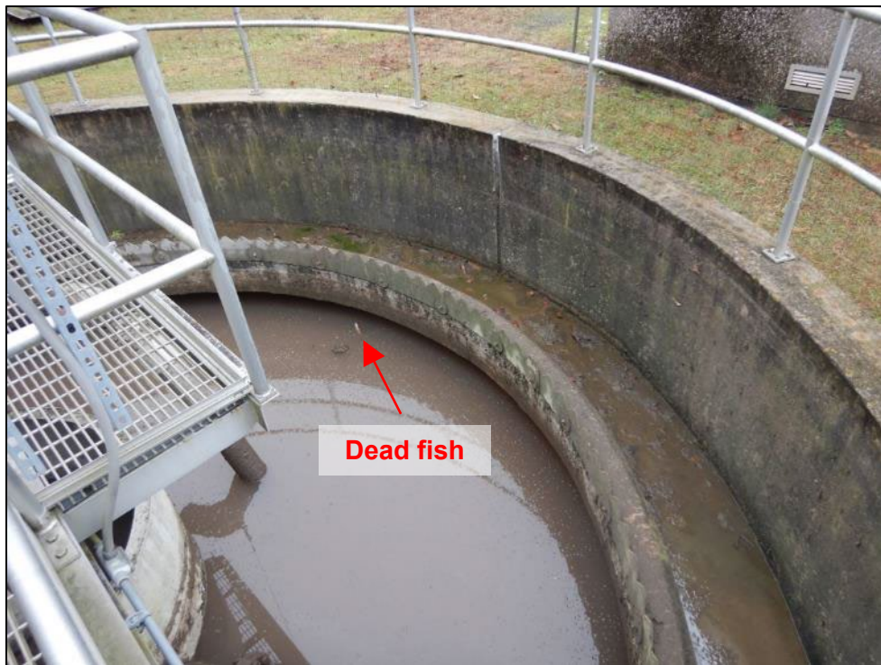
Photograph 16. (DSCN0063) Additional view inside clarifier. The clarifier contained sludge and dead fish at the time of the inspection; Facility representatives stated that the clarifier is not cleaned frequently.
