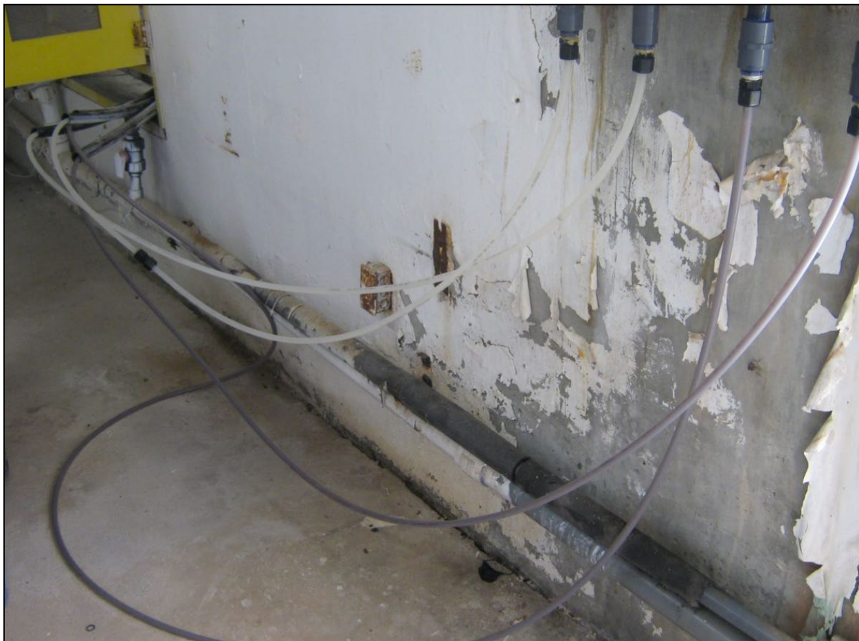
Photograph 37. Chlorine Lines, WTP #1 Alternate view of the chlorine pump lines on the floor in the chemical injection room at WTP #1. The lines presented a tripping hazard.
