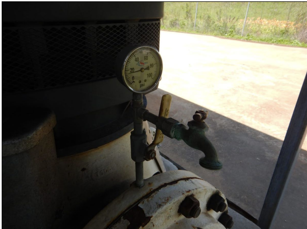
Photograph 5. Well No. 20 View of a threaded hose tap and pressure gauge extending off of the Well No. 20 pump line. The hose tap did not have backflow prevention.
