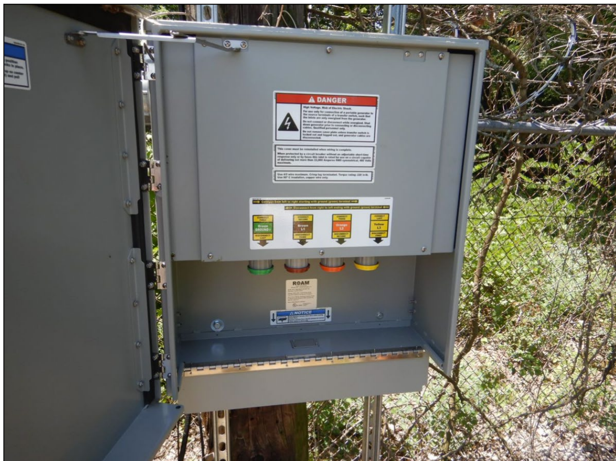
Photograph 19. Generator Connection, Well No. 17 View of the generator connection box at Well No. 17. The Operations Manager stated that this box enabled easy connection to the portable generators.
