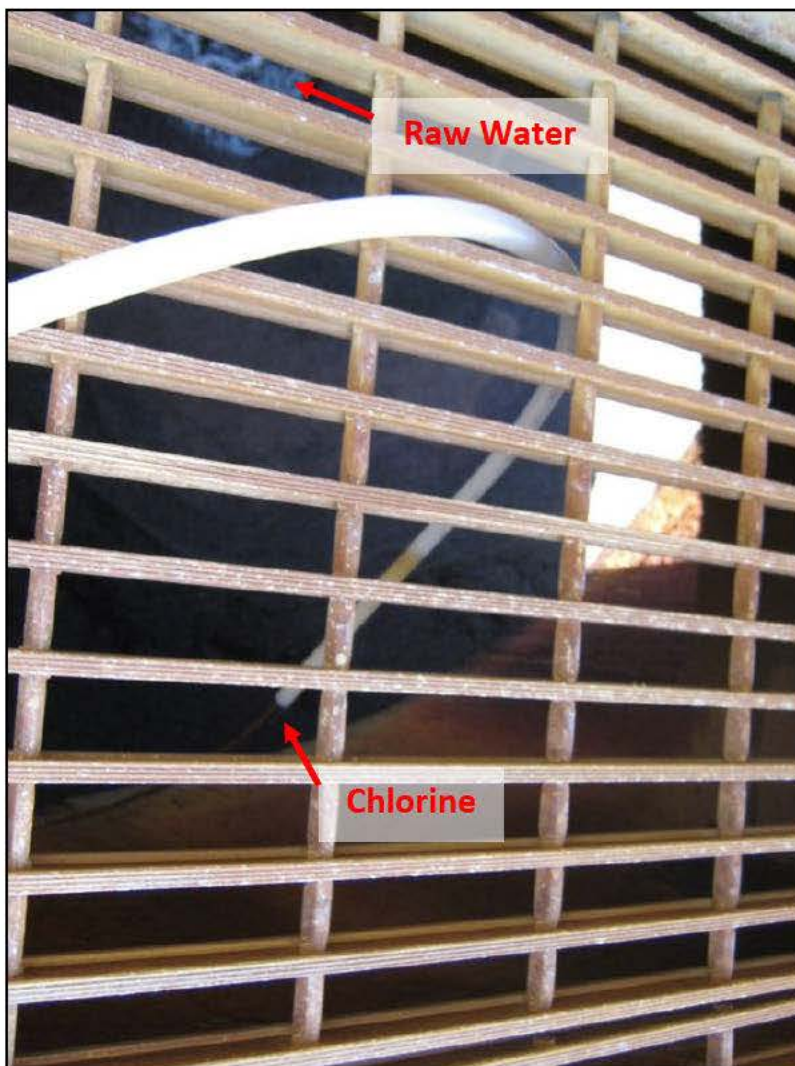
Photograph 23. Filter No. 2 Chlorine Injection Tube, WTP #1 View of the chlorine injection tube that was sending chlorine against the wall of the Filter No. 2 basin. Since the water was below the filter media in the basin, the chlorine was not mixing with the raw water prior to filtration.
