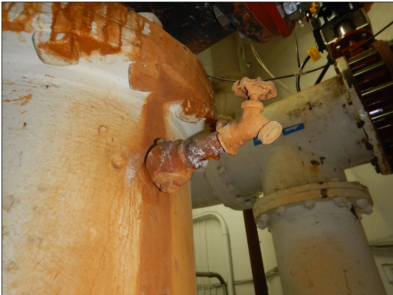
Photograph 30. Raw Water Line, WTP #1 View of a threaded hose tap that extended off of the raw water line at WTP #1. The hose tap did not have backflow prevention.
