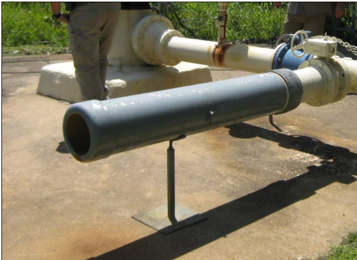
Photograph 16. Well No. 17 View of the pump to waste line at Well No. 17. The line was valved off from the line into the treatment system, but the end of the line was uncovered.
