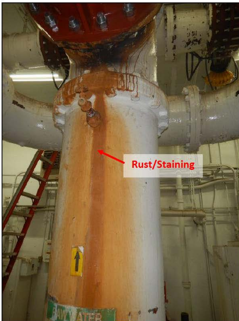
Photograph 29. Raw Water Line, WTP #1 View the influent raw water line in the pipe gallery at WTP #1. There was rust/staining on the line, and it appeared that the rust had come from a valve leak. The leaking valve was the only valve separating raw influent water from being sent into the distribution system.
