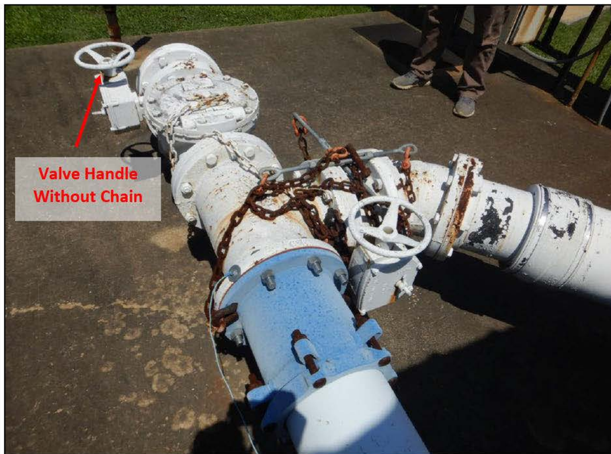
Photograph 11. Well No. 18 View of the pump line and valves at Well No. 18. There was a chain sitting next to the valve handle that closed off flow to the treatment system. An operator stated that the chain was supposed to be threaded through the valve handle to prevent it from accidentally being opened.
