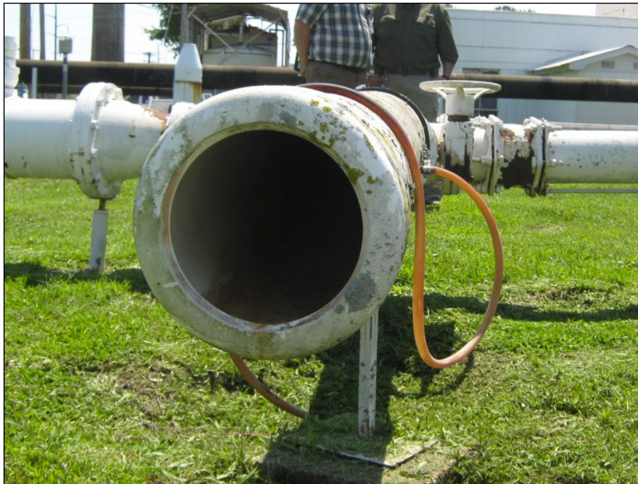
Photograph 4. Well No. 20 View of the pump to waste line at Well No. 20. The line was valved off from the line into the treatment system, but the end of the line was uncovered.
