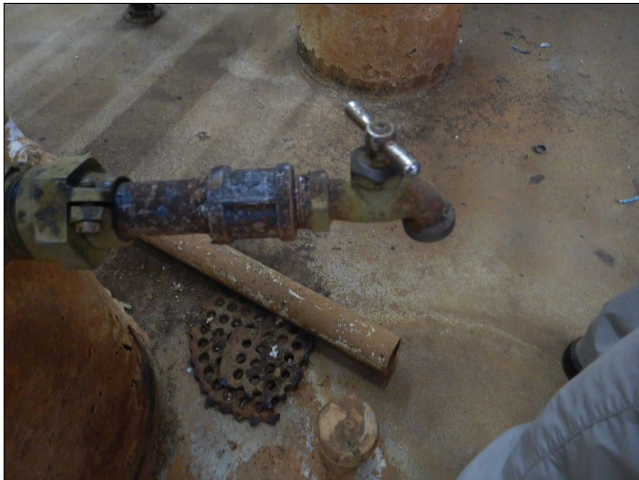
Photograph 31. Raw Water Line, WTP #1 View of a second threaded hose tap that extended off of the raw water line at WTP #1. The hose tap did not have backflow prevention.
