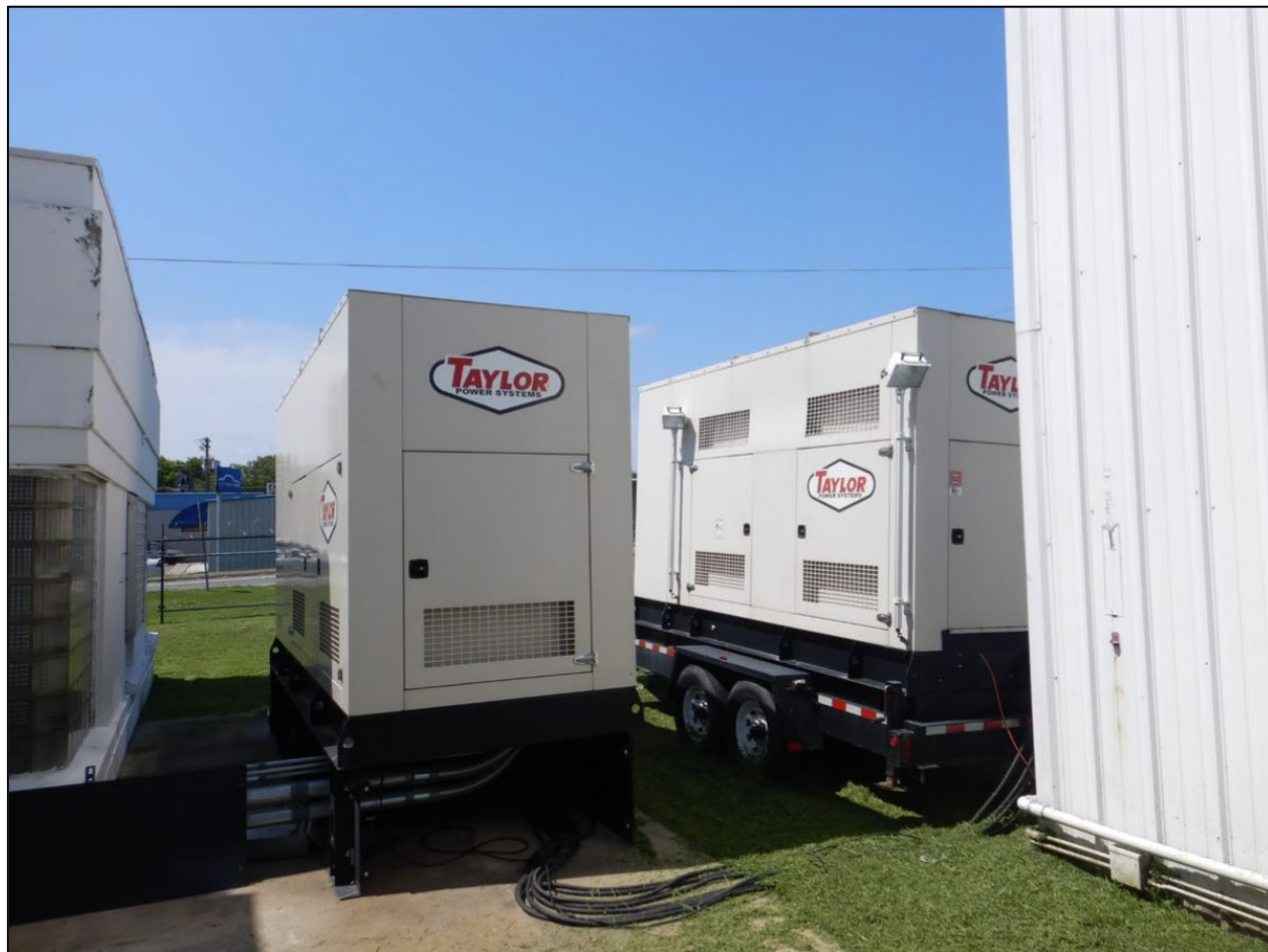
Photograph 20. Generators, WTP #1 View of the mounted backup generator and portable backup generator that were positioned at WTP #1. The mounted generator was out of service, so the portable generator had been brought in and wired through the mounted generator's switch gear. The trailer generator had turned on automatically and ran the treatment plant on the night prior to the inspection.
