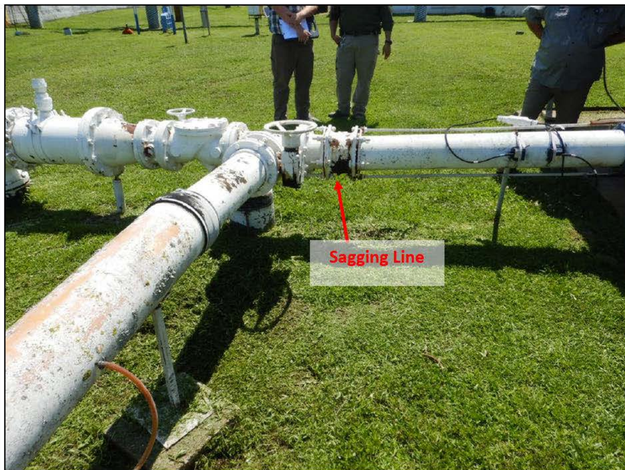
Photograph 2. Well No. 20 View of the pump line of Well No. 20. The line was sagging, and it appeared that a support stand was missing under the line.
