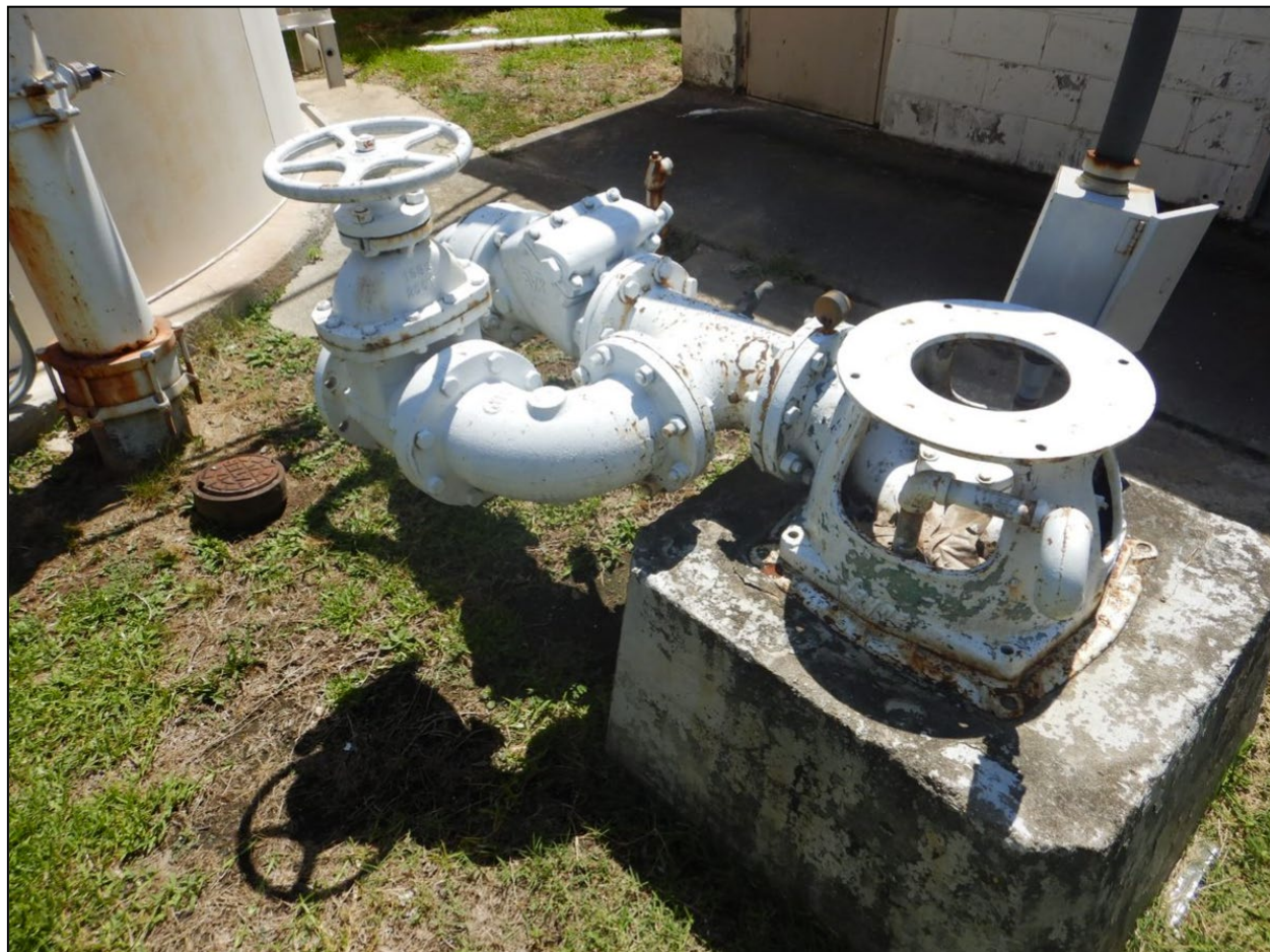
Photograph 39. Well No. 28 View of Well No. 28 at the White Hall property. System representatives stated that the well had been out of service for several years due to its proximity to a bathroom. If the well was in service, it would pump raw water to White Hall WTP #4.
