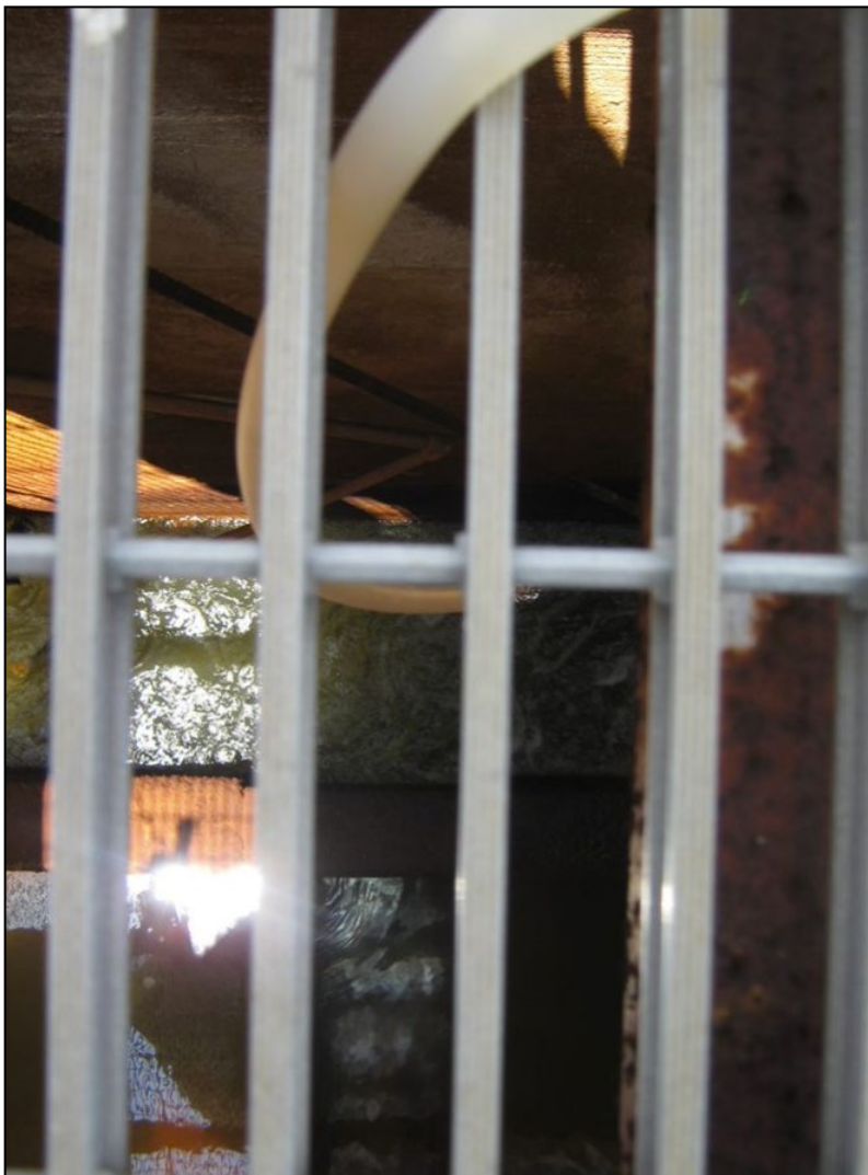
Photograph 24. Filter No. 4 Chlorine Injection Tube, WTP #1 View of the chlorine injection tube that was sending chlorine into the raw water at Filter No. 4 to mix prior to being filtered.
