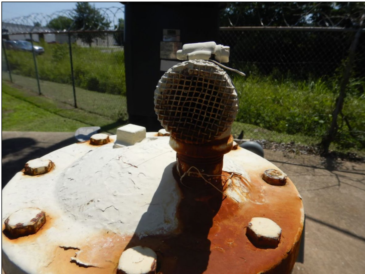
Photograph 18. Well No. 17 View of an air relief valve that extended off of the Well No. 17 pump line. The valve opening was screened but not downturned.
