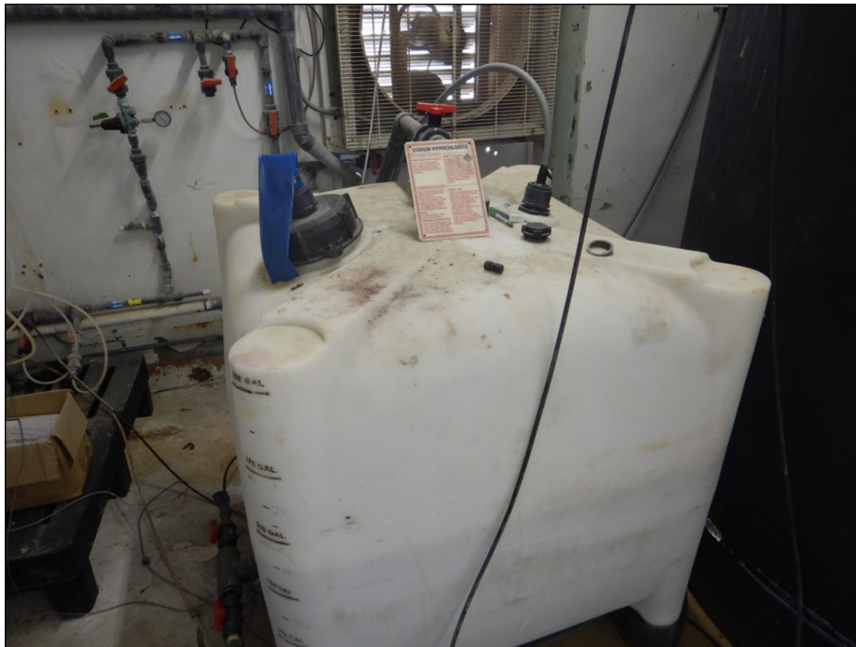
Photograph 33. Chemical Storage/Injection Room, WTP #1 View of the sodium hypochlorite day tank inside the chlorine storage room at WTP #1. The tank had a label sitting on top of it.
