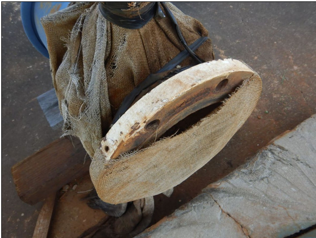
Photograph 10. Well No. 18 View of the end of the pump line that was attached to the pump at Well No. 18 prior to its removal. The end of the line was covered with a burlap sack. The sack was ripped in multiple places creating openings to the pump line.
