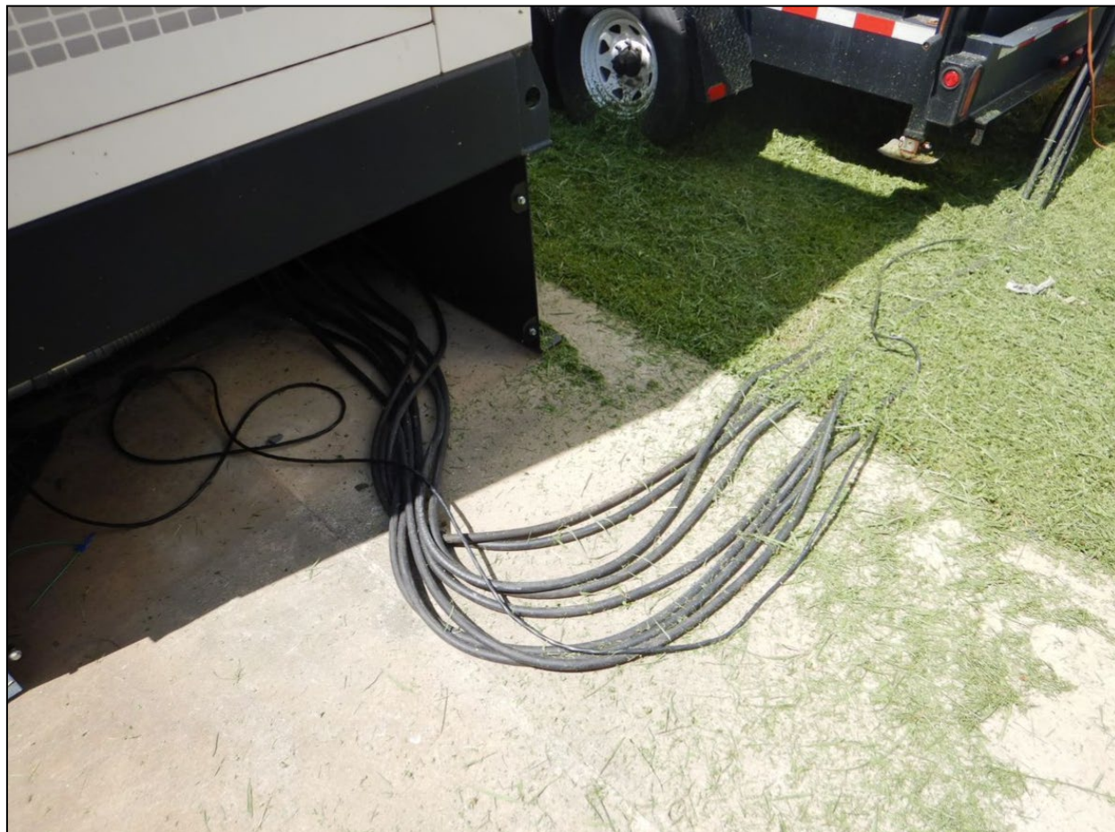
Photograph 21. Generators, WTP #1 View of the wiring between the trailer backup generator and the mounted generator at WTP #1. The trailer generator was wired through the mounted generator's switch gear so that it would turn on automatically in the event of a power outage.
