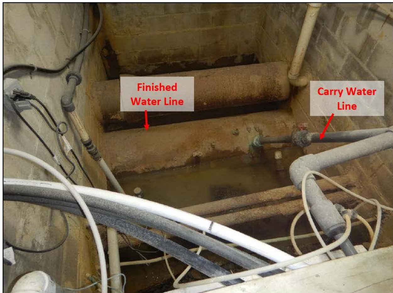
Photograph 35. Carry Water Line, WTP #1 View of the carry water line that extended off of the finished water line. There was no backflow prevention on the line.
