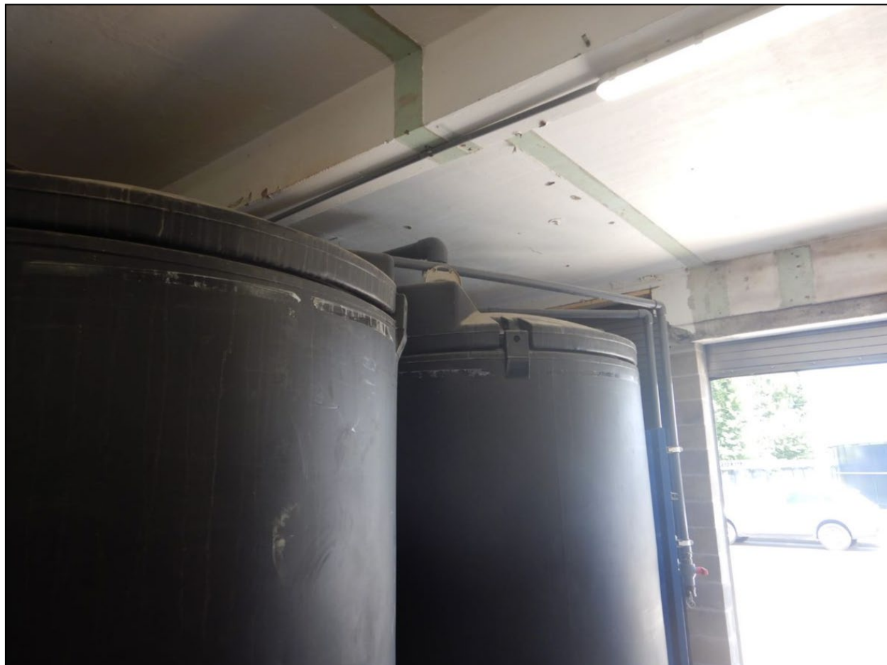
Photograph 32. Chemical Storage/Injection Room, WTP #1 View of the two sodium hypochlorite bulk storage tanks inside of the chemical storage room at WTP #1. The tanks were not labeled.
