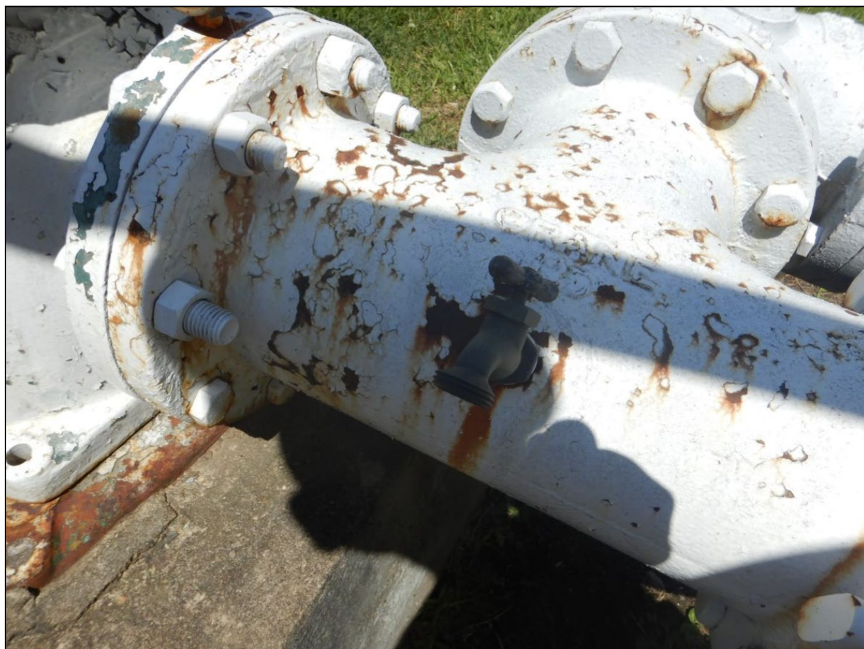
Photograph 41. Well No. 28 View of a threaded hose tap without backflow prevention that extended off of the pump line at Well No. 28.
