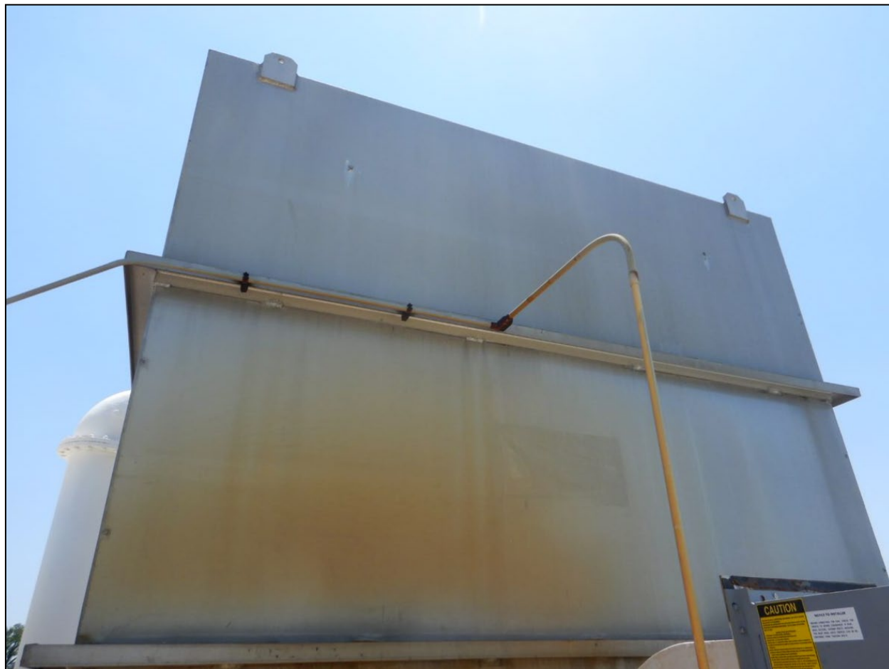
Photograph 22. Aerator No. 2, WTP #1 View of the aerator that was associated with Filter No. 2 at WTP #1. Raw water is pumped into the plant, and it cascades through the aerators prior to being filtered.
