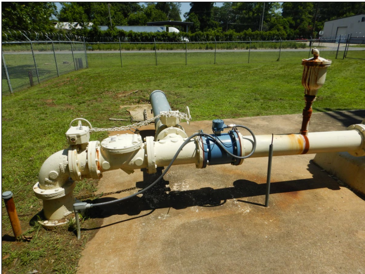
Photograph 12. Well No. 17 View of Well No. 17. The well was fully functional. The well is used to pump raw water to WTP #1.
