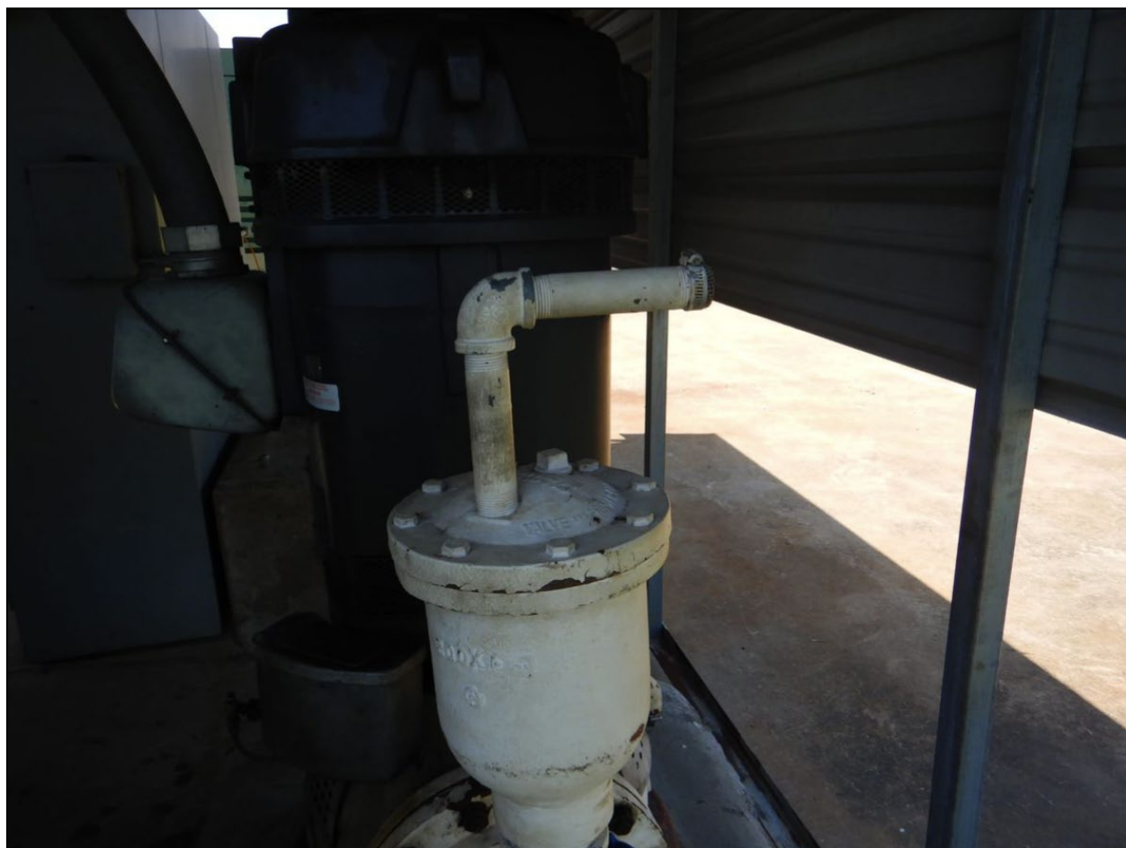
Photograph 6. Well No. 20 View of an air relief valve extending off of the pump line at Well No. 20. The opening was screened but the valve was not downturned.
