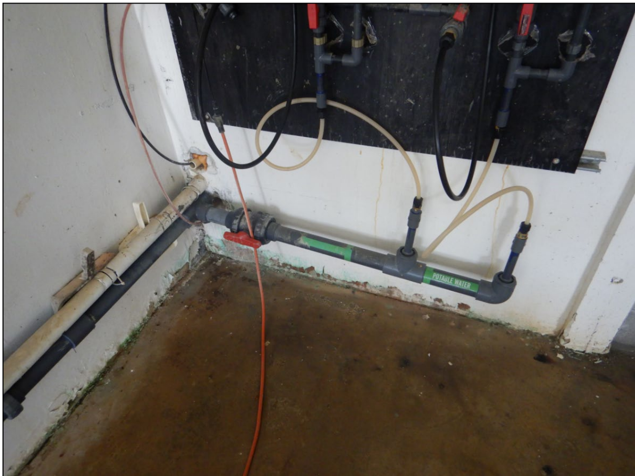
Photograph 34. Carry Water Injection Point, WTP #1 View of the point where carry water is injected to facilitate sodium hypochlorite injection. There was no backflow prevention on the carry water line.
