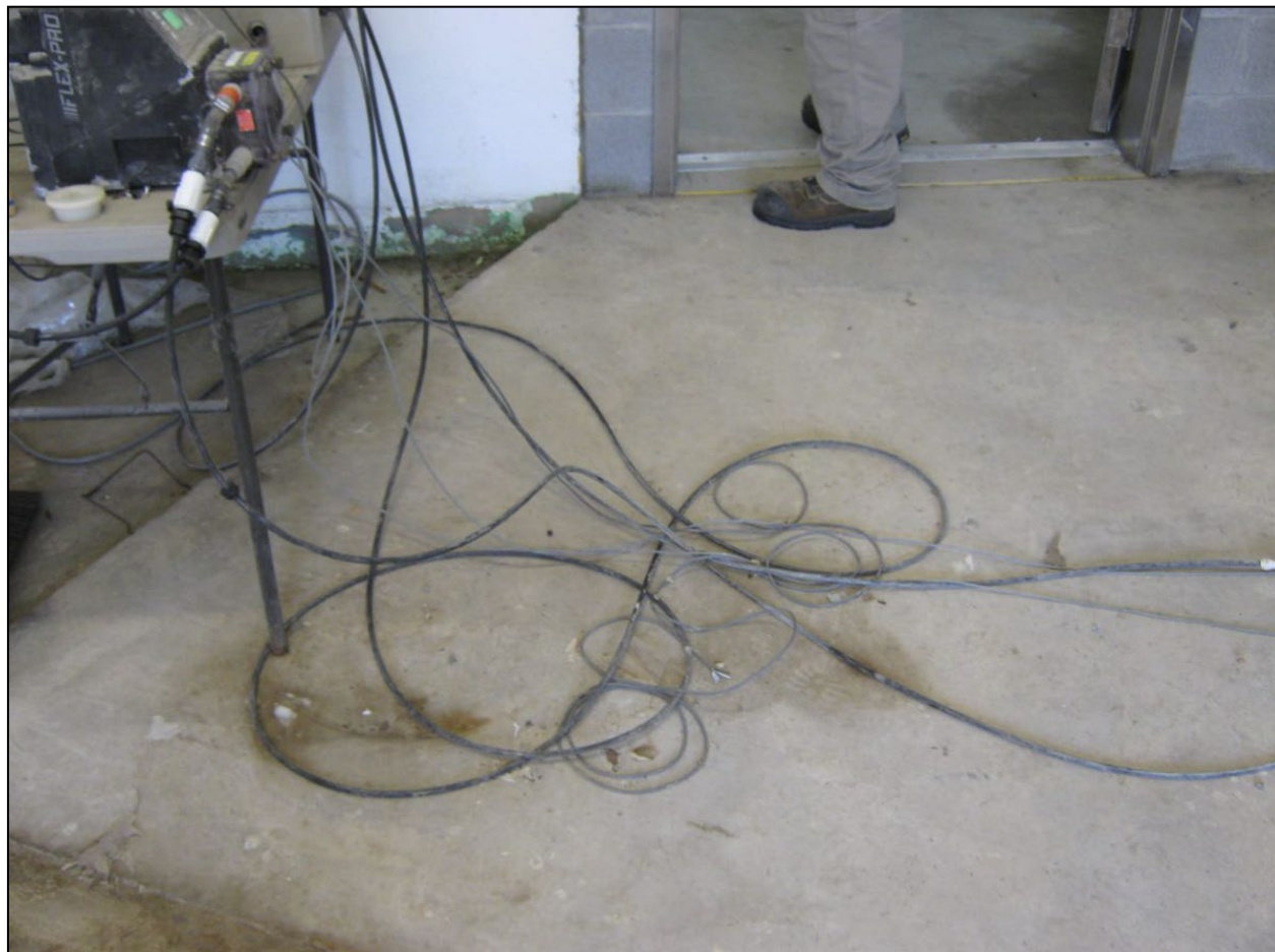
Photograph 36. Chlorine Lines, WTP #1 View of the chlorine pump lines on the floor in the chemical injection room at WTP #1. The lines presented a tripping hazard.
