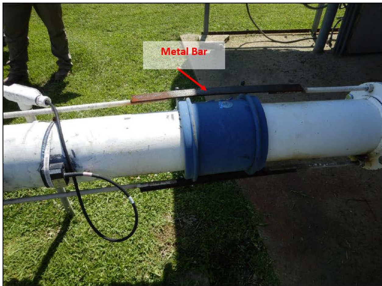
Photograph 3. Well No. 20 View of the pump line at Well No. 20. Metal bars had been welded to the support rebar. System representatives stated that the metal bars had been used because the rebar was not long enough.
