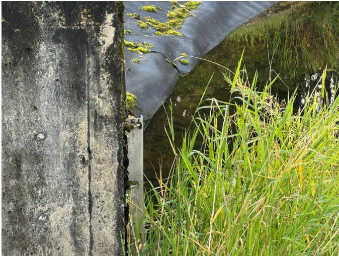
Photo #:19 (8473) Description: Effluent pipe to wetlands.
