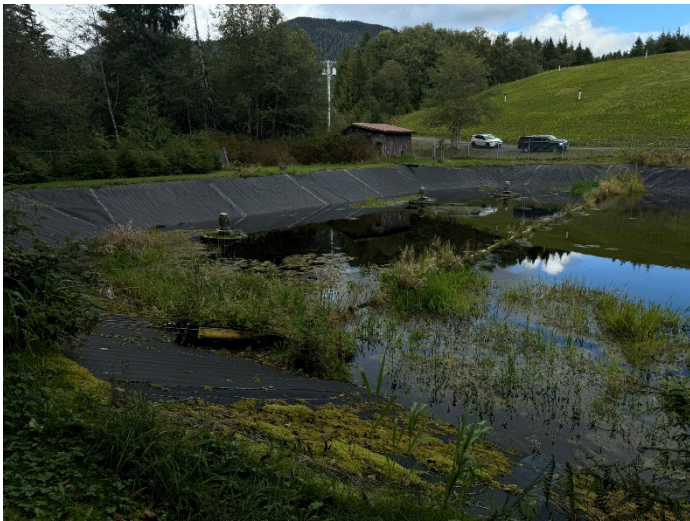
Photo #:39 (8515) Description: Wastewater lagoon with vegetative growth.
