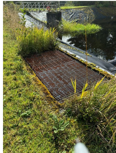
Photo #:16 (8467) Description: Influent sump.
