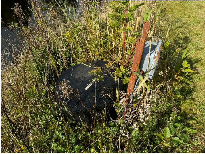
Photo #:21 (8477) Description: Groundwater dewatering pump #2.
