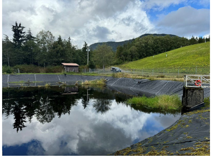
Photo #:38 (8514) Description: Wastewater lagoon with vegetative growth.
