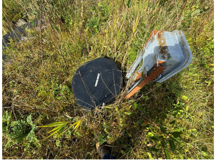
Photo #:14 (08464) Description: Groundwater dewatering pump #1
