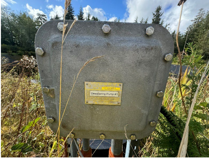
Photo #:13 (08463) Description: Groundwater dewatering pump #1.
