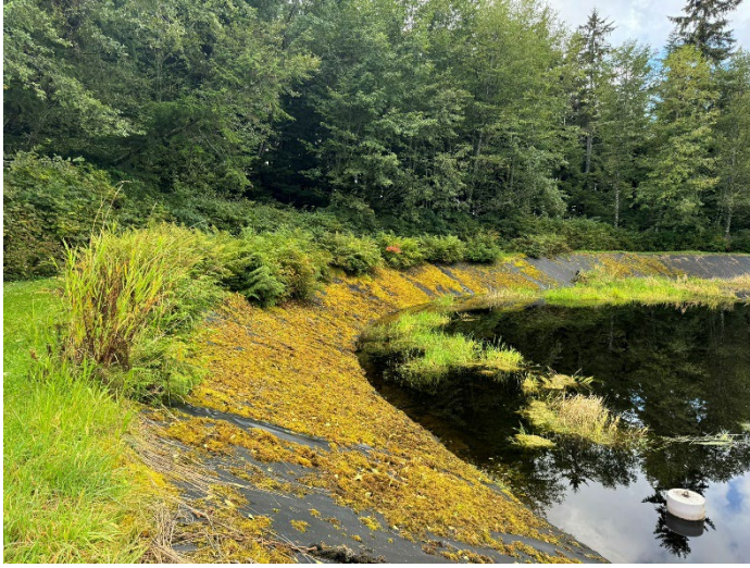
Photo #:37 (8513) Description: Wastewater lagoon with vegetative growth.
