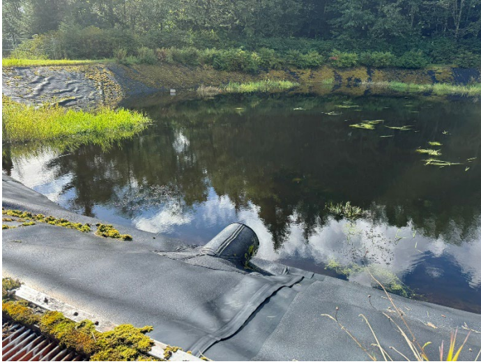
Photo #:17 (8469) Description: Overflow pipe.
