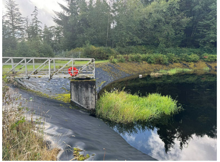
Photo #:18 (8472) Description: Effluent pipe to wetlands.
