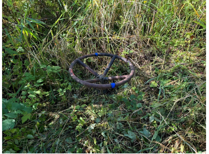
Photo #:22 (8479) Description: Pinch valve to shutoff flow to wetlands.
