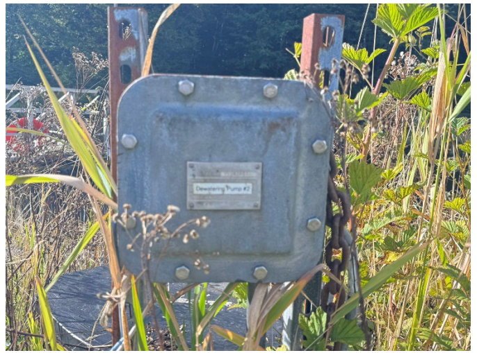
Photo #:20 (8476) Description: Groundwater dewatering pump #2.
