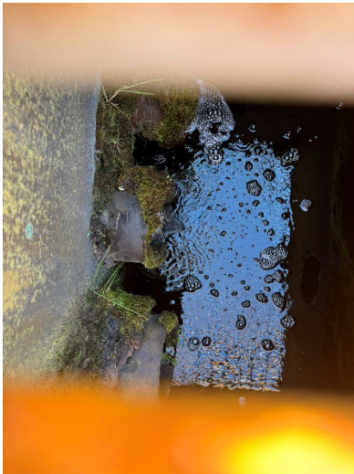
Photo #:15 (08466) Description: Influent sump.
