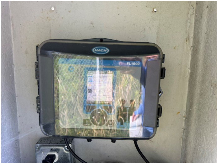
Photo #:23 (8481) Description: Flow meter.
