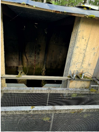
Photo #:25 (8484) Description: Weir for effluent flow to discharge pipe and sample location.
