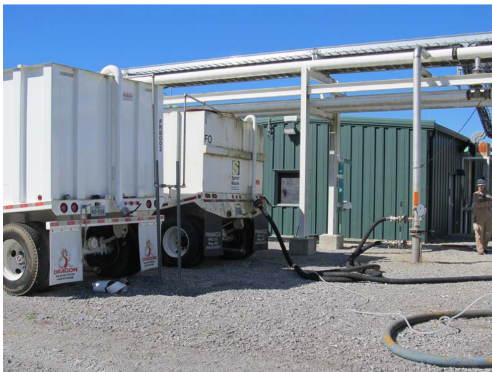
Photo 5 – two frac tanks connected to internal outfall 302
