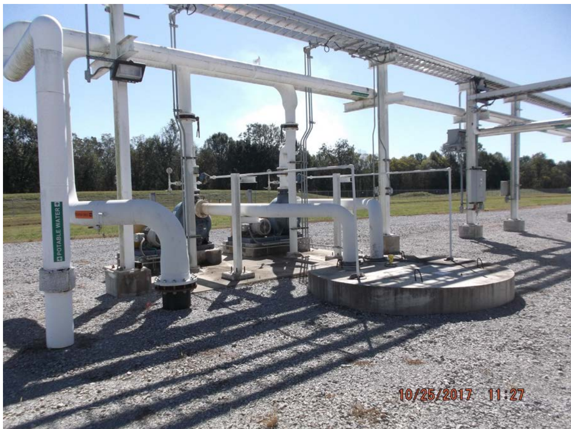
Photo 6 – Lift station with all internal outfalls combining before discharging to 002
