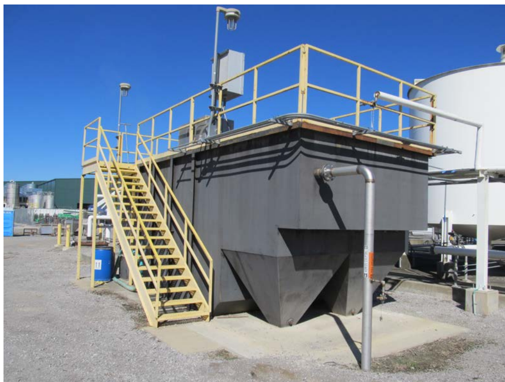
Photo 3 – Sanitary Wastewater Treatment (package) Plant
