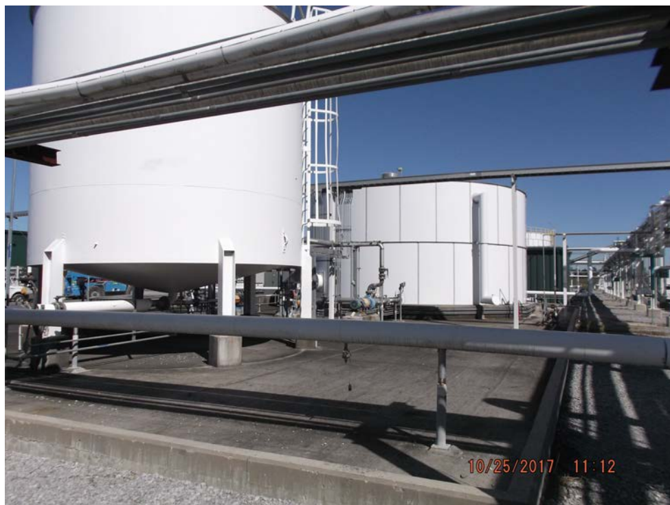
Photo 4 – Equalization tanks and internal outfall 402
