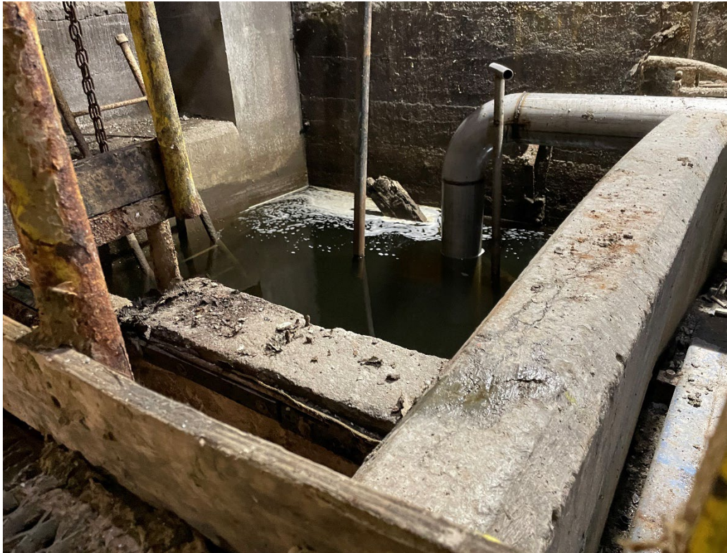
Photo #3. River water is pumped into the water receiving chest before it is treated.
