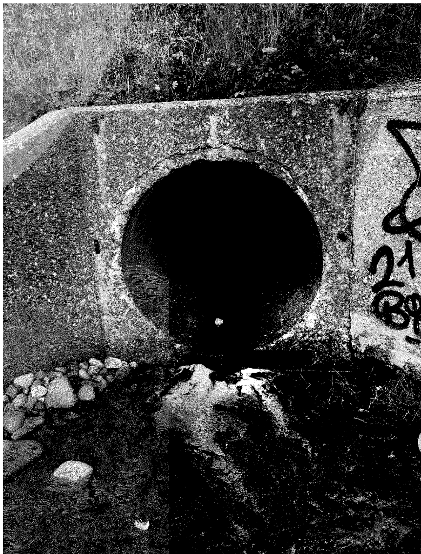
SB02 : Close-up of SB02. Note the green algae growth and orange suds in the pool downstream of the pipe. Sample collection point indicated by a red arrow.
