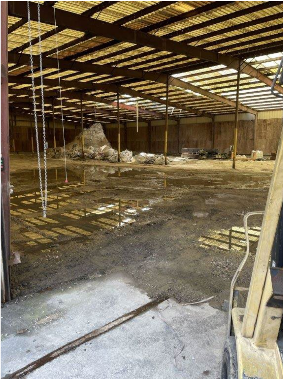
Photograph 11: Building 139, Pile of Bath Salts Material and Supersacks of Crushed Bath Material Containing Cryolite. Maintenance issues are visible with the roof and clear liquid is covering a significant portion, approximately half, of the visible floor.
