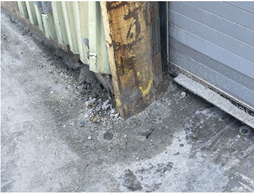
Photograph 37: Building 138, loose siding with a small release of K088 hazardous waste.
