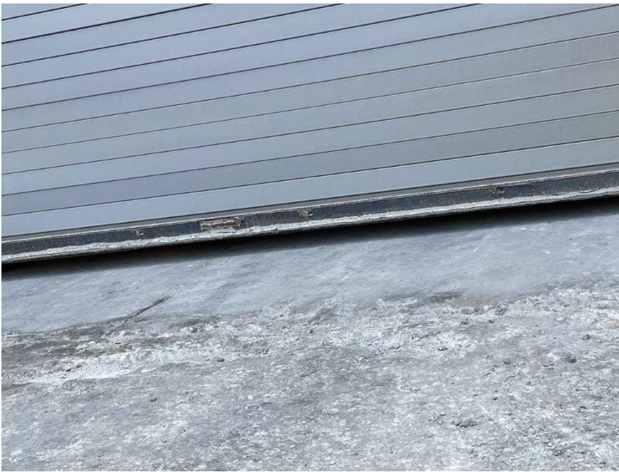
Photograph 38: Roll-up vehicle door on Building 138 will not close due to a build-up of K088 hazardous waste at the sides of the door.
