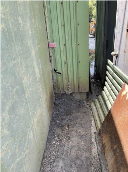
Photograph 36: Small hole in the wall of Building 138 and loose siding near the building's foundation. A small release of K088 hazardous waste is shown.
