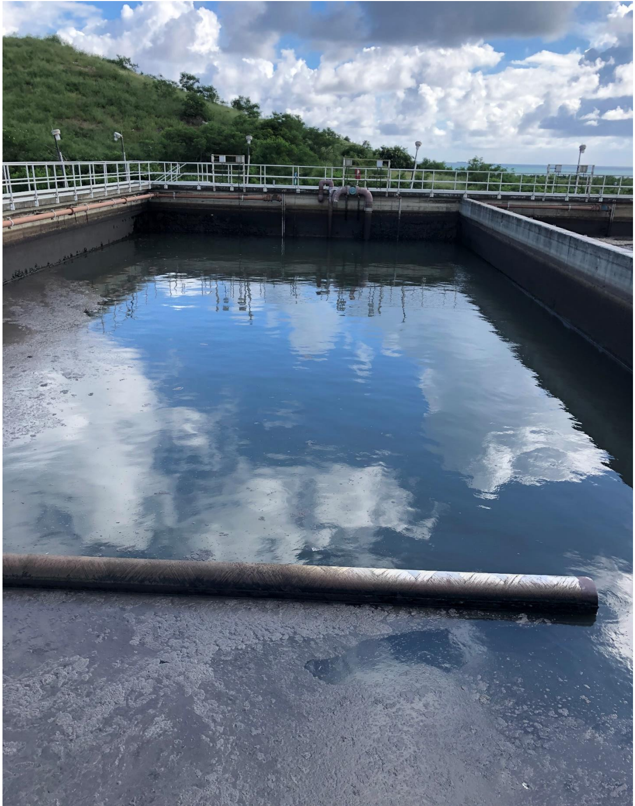
Photo #5: View of SBR 3.
