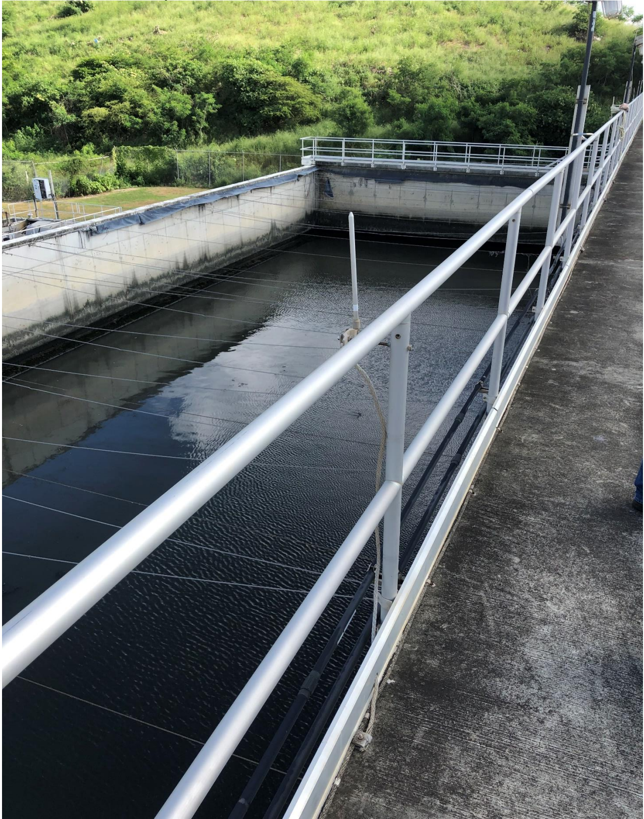
Photo #6: View of the equalization tank.
