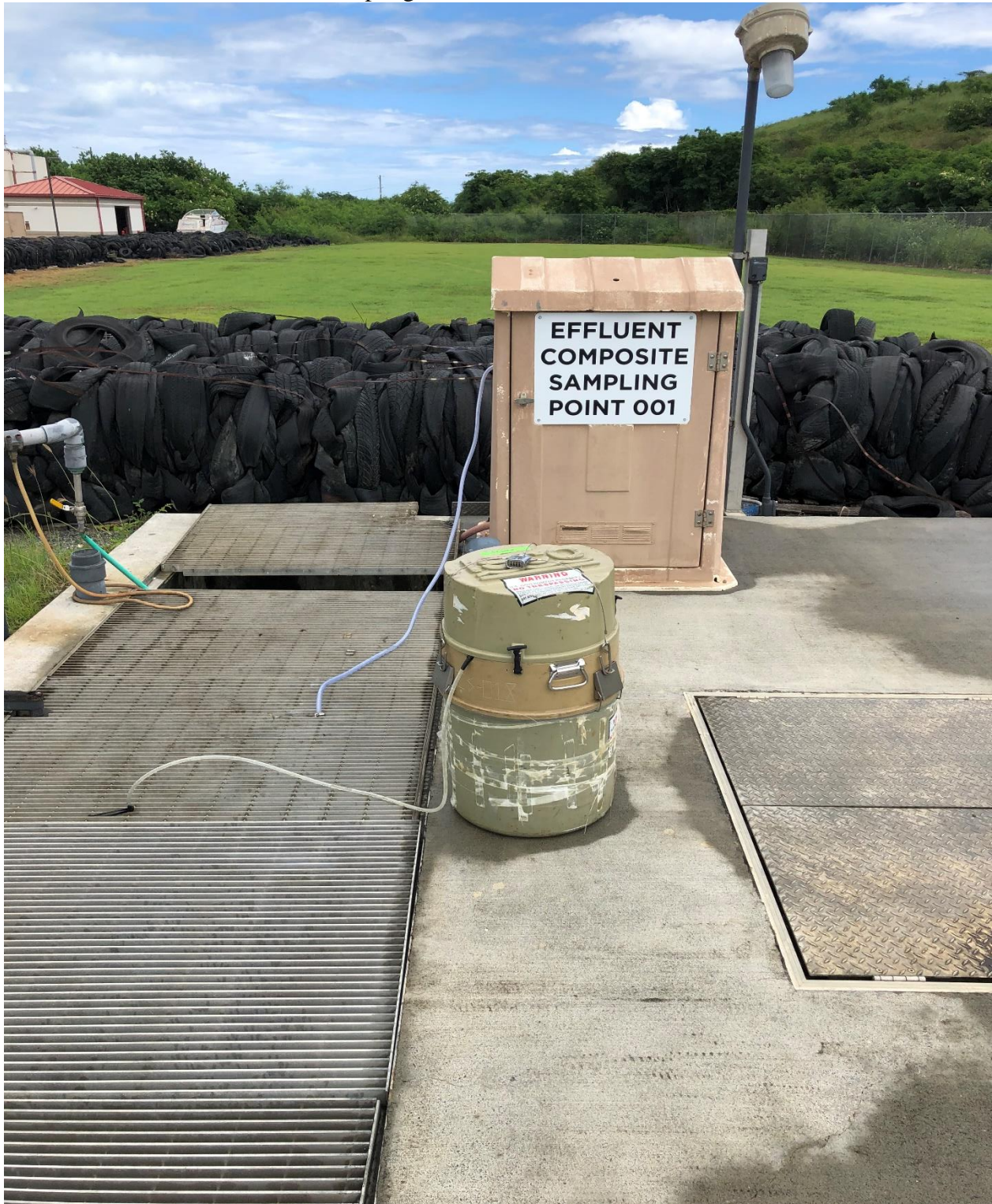
Photo #1: View of the effluent sampling location for Outfall 001.
