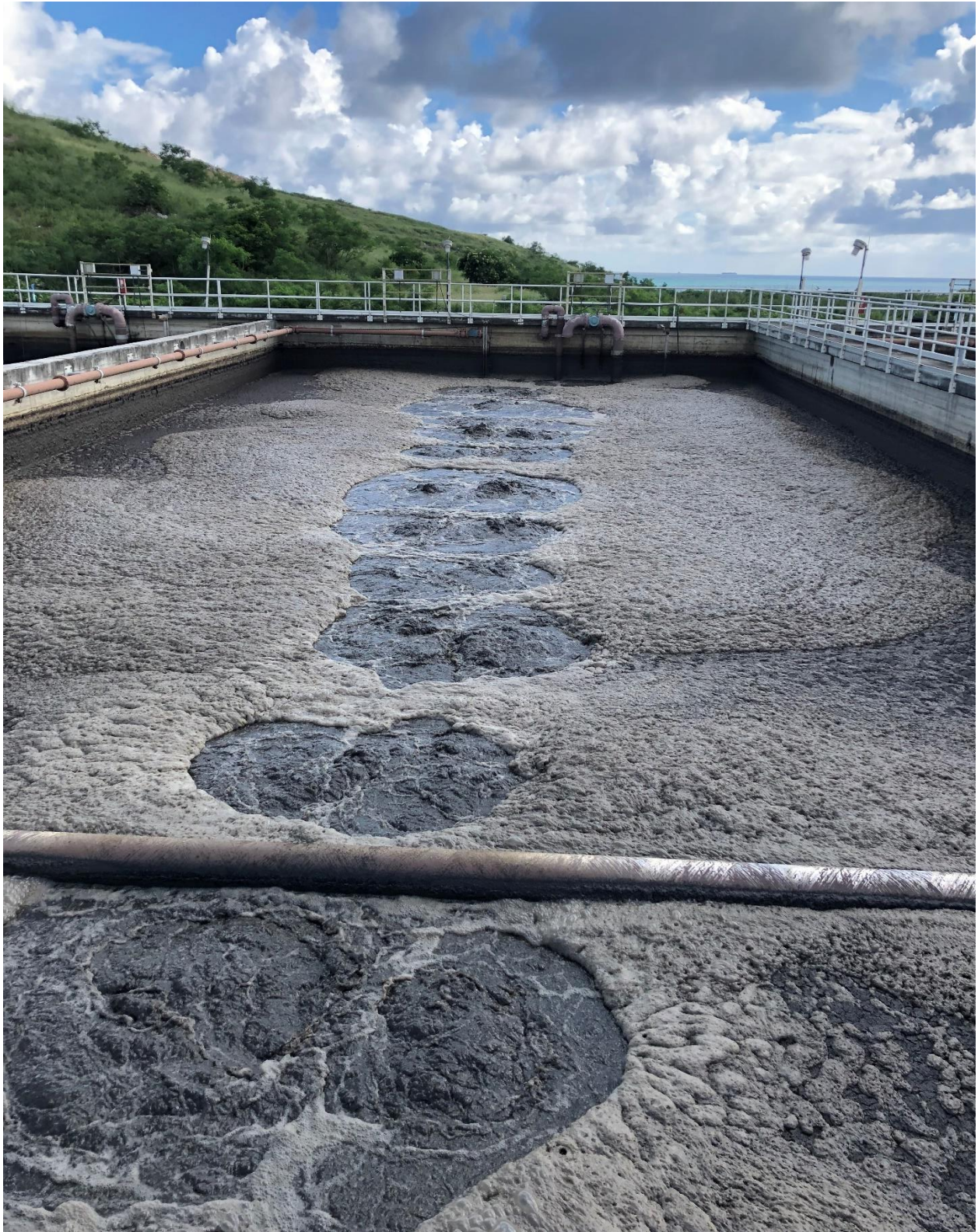
Photo #4: View of SBR 2.
