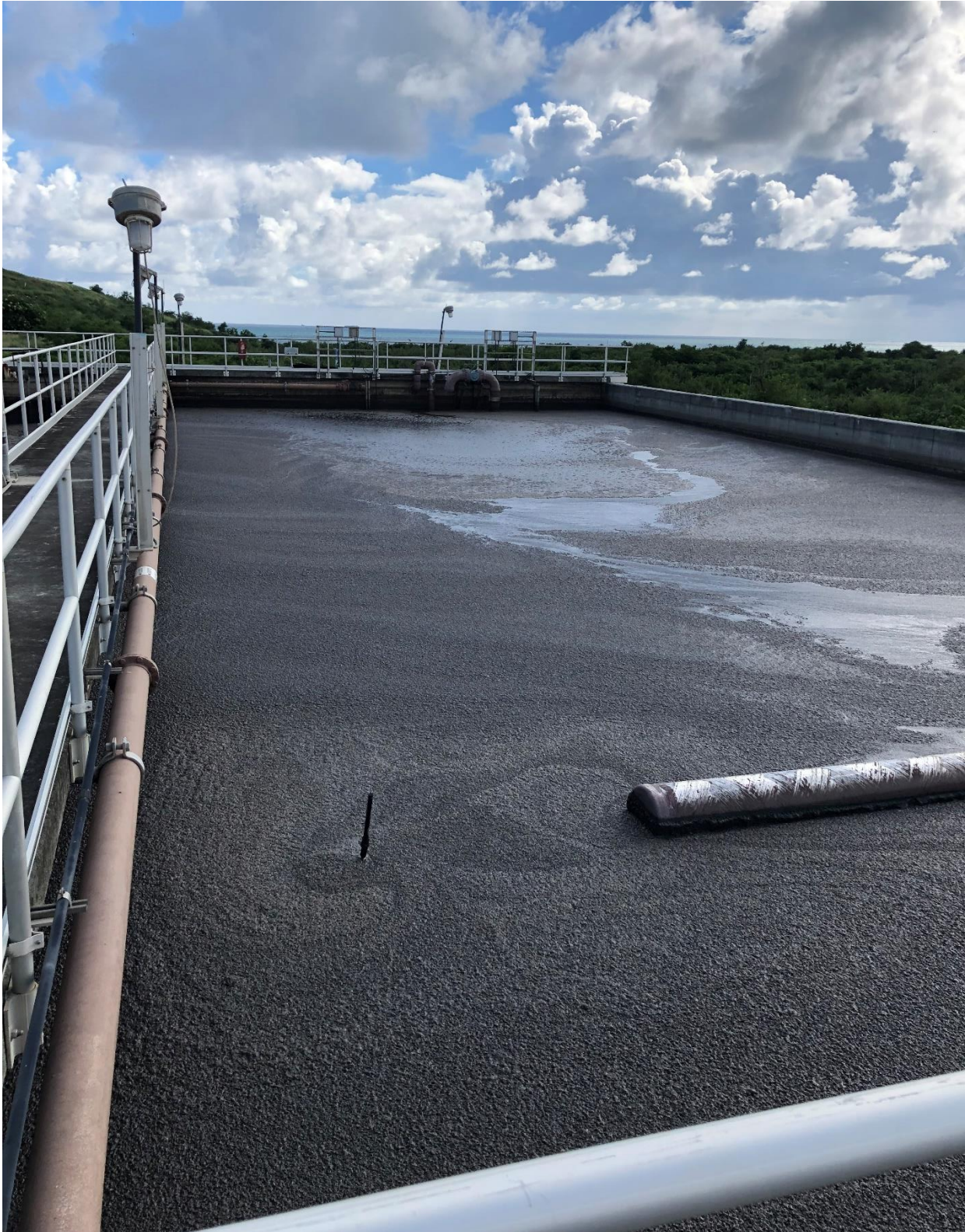
Photo #3: View of SBR 1.
