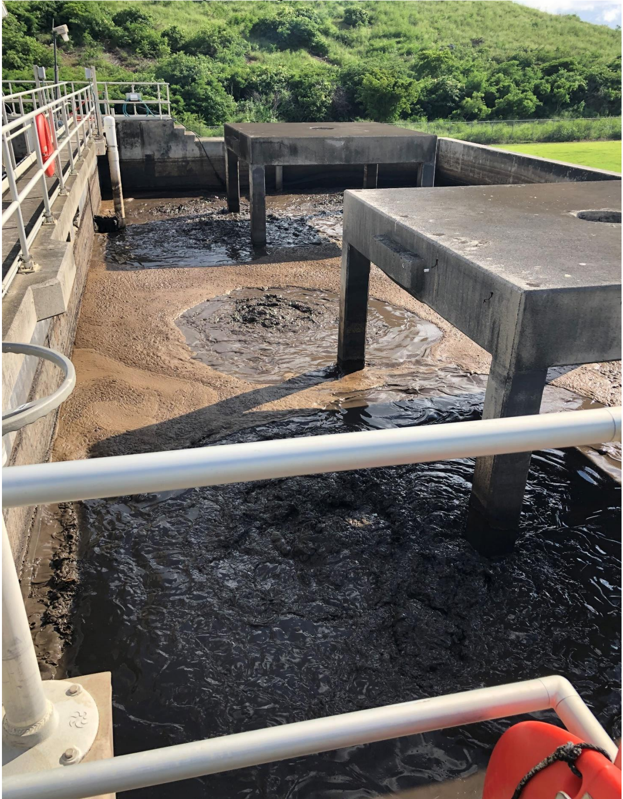
Photo #7: View of the secondary aerobic digester.
