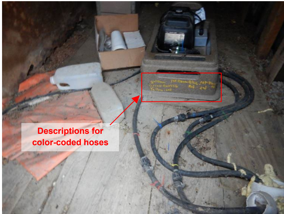
Photograph 25. (DSCN9132) View inside shed of an aeration compressor and four air-delivery hoses. The hoses were color-coded; the yellow writing described where the hoses delivered air in the ponds. The compressor was not operating at the time of the inspection, and it was unclear if the equipment was operable or used in the treatment process.
