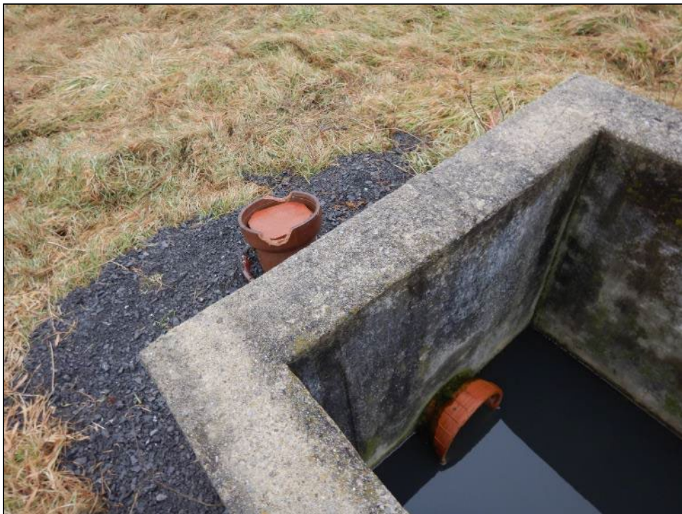
Photograph 20. (DSCN9122) View of end of effluent pipe in chlorine contact tank. Effluent that enters this pipe flows to Outlet 001.
