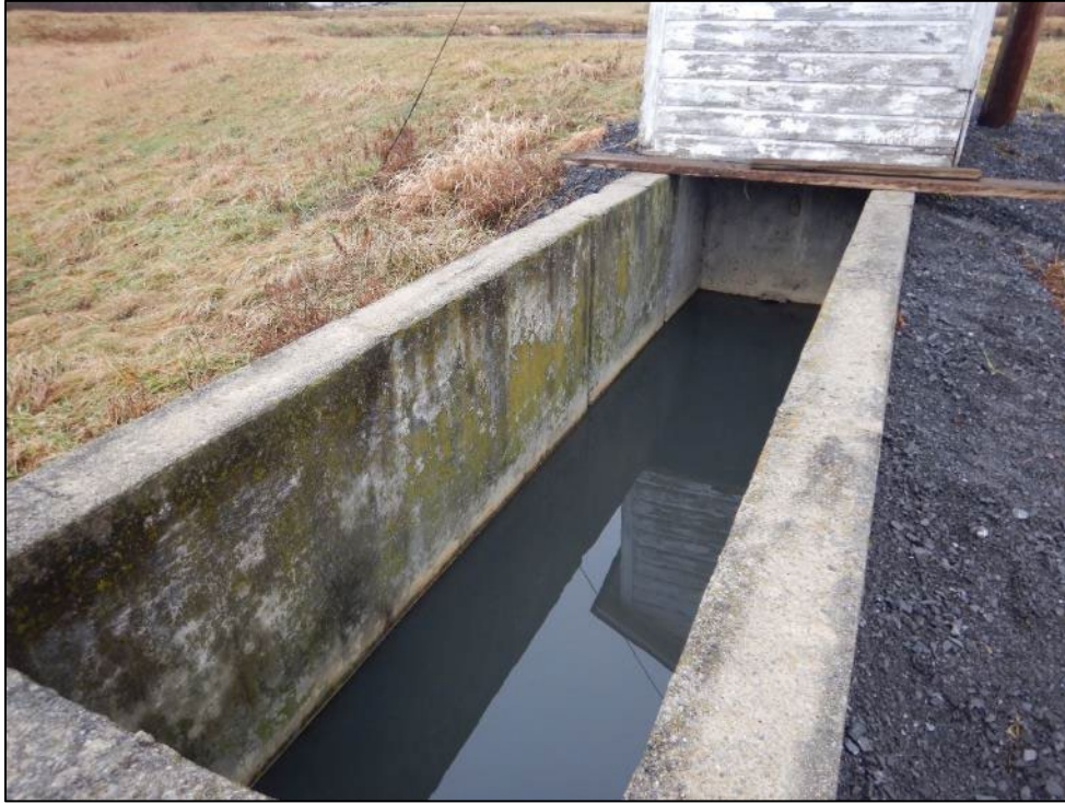
Photograph 19. (DSCN9121) View of chlorine contact tank, per description provided in Permit. The Permittee was not disinfecting the effluent at the time of the inspection. Permittee representatives stated effluent compliance samples are obtained from this tank.
