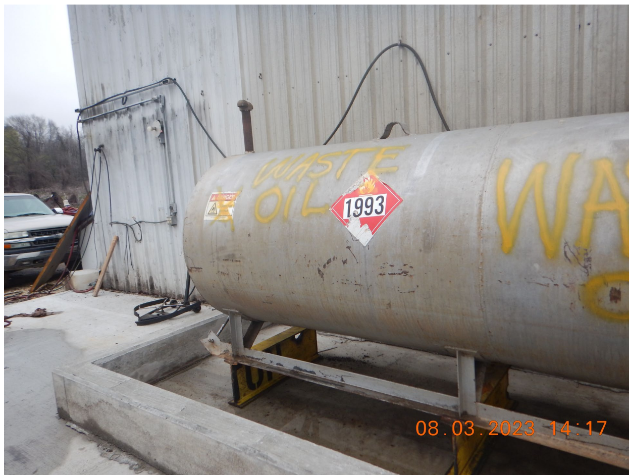
Another view of one (1) of the Facility on-sites ASTs and a recently completed concrete containment berm Note: the lack of proper labeling or signage. (DSCN2347) Photographed by C. Sherwood.
