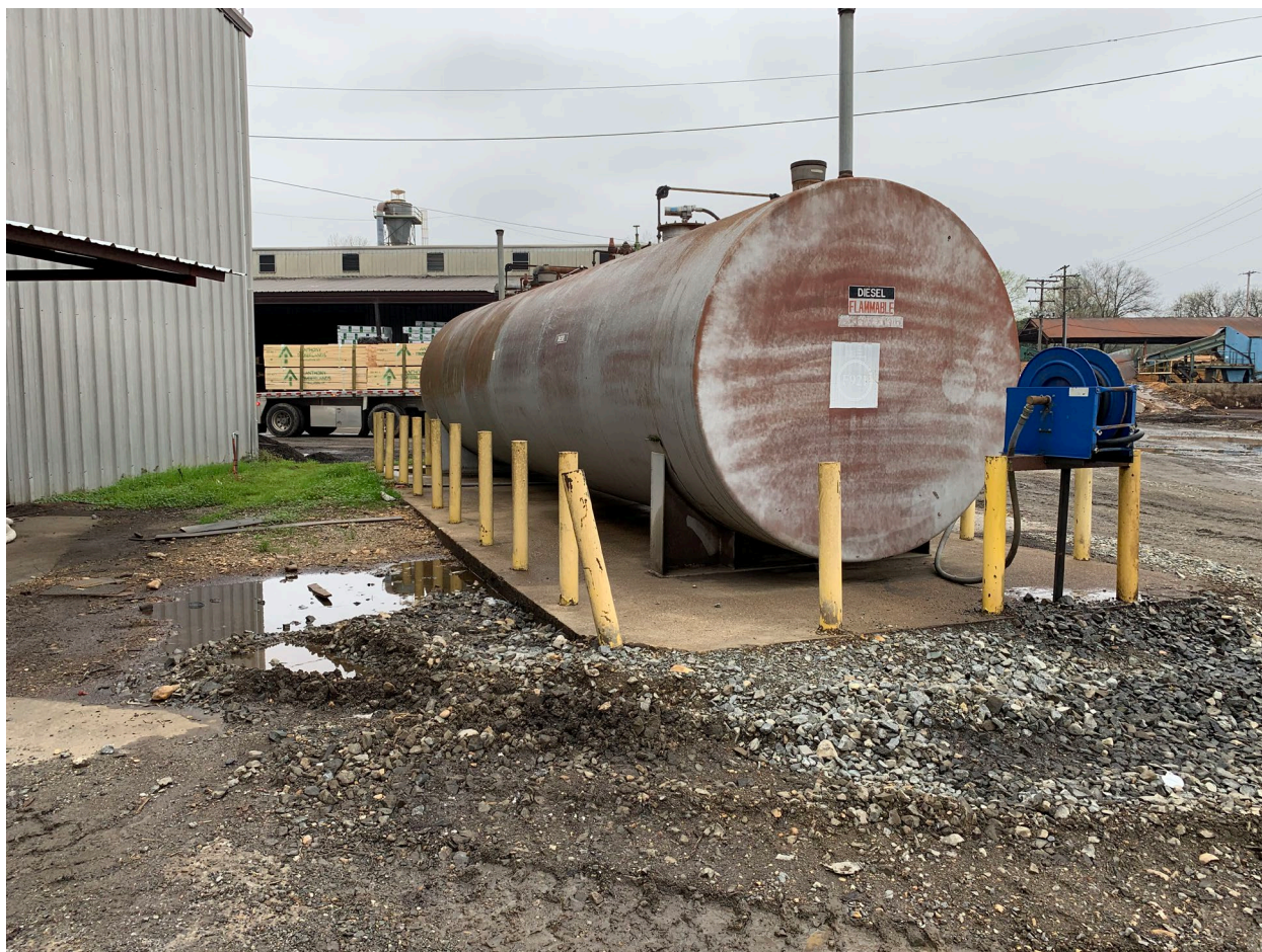
View of one (1) of the Facility on-sites ASTs. Note: the lack of proper labeling, signage, containment, and damaged bollard. (IMG_0179) Photographed by D. Esparza.
