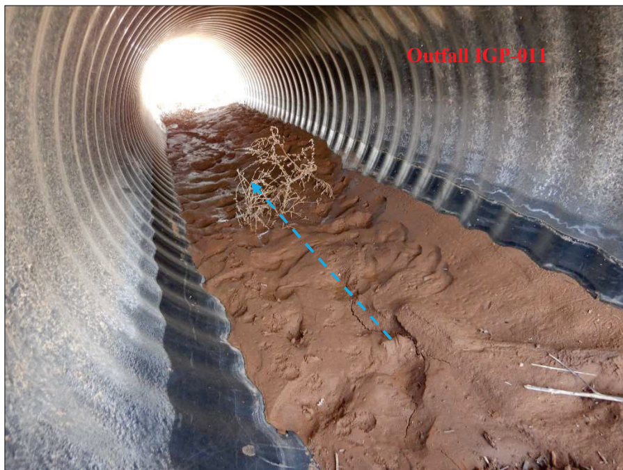
Photograph 104. Additional view, facing Southwest, of the inside of Outfall IGP-011, as referenced in Photographs 101 and 102. Note sediment accumulation.
