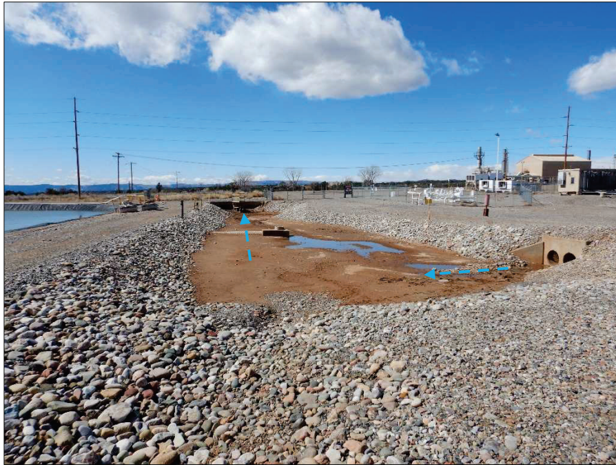
Photograph 55. Additional view, facing West, of North Evaporation Stormwater Holding Pond, as referenced in Photographs 53 and 54. Note sediment accumulation in the pond.
