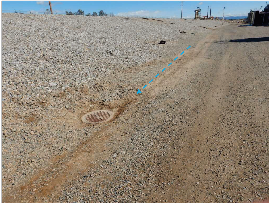
Photograph 81. View, facing East, of catch basin in Drainage Area 1. Note loose gravel and sediment near entrance of catch basin.
