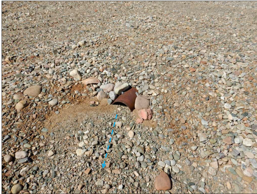
Photograph 93. Close-up view, facing Southeast, of the outlet of a culvert that discharges into the ditch leading to Outfall IGP-006, as referenced in Photographs 91 and 92. Note accumulated sediment and gravel obstructing the culvert outlet pipe.
