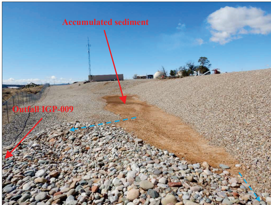
Photograph 99. Additional view, facing Southwest, of sediment accumulation near Outfall IGP-009, as referenced in Photographs 97 and 98.
