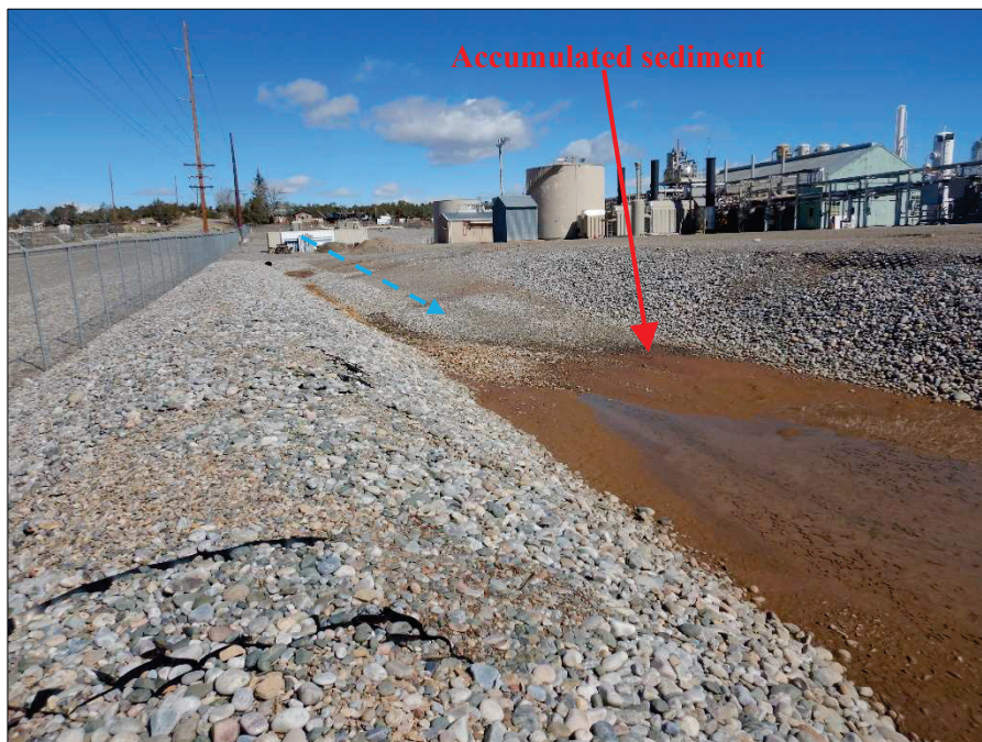
Photograph 66. Additional view, facing North, of inlet to Gosney Pond, as referenced in Photographs 64 and 65. Note accumulated sediment in the pond.
