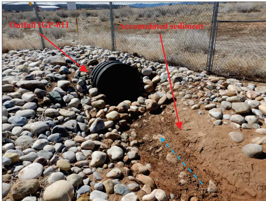
Photograph 103. Close-up view, facing Southwest, of Outfall IGP-011, as referenced in Photograph 102. Note sediment accumulation.
