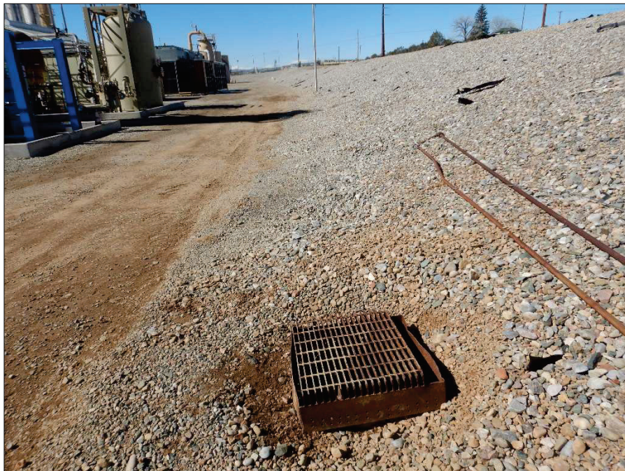
Photograph 82. View, facing West, of catch basin in Drainage Area 1. Note structure is not seated in ground and loose gravel and sediment near entrance of catch basin.
