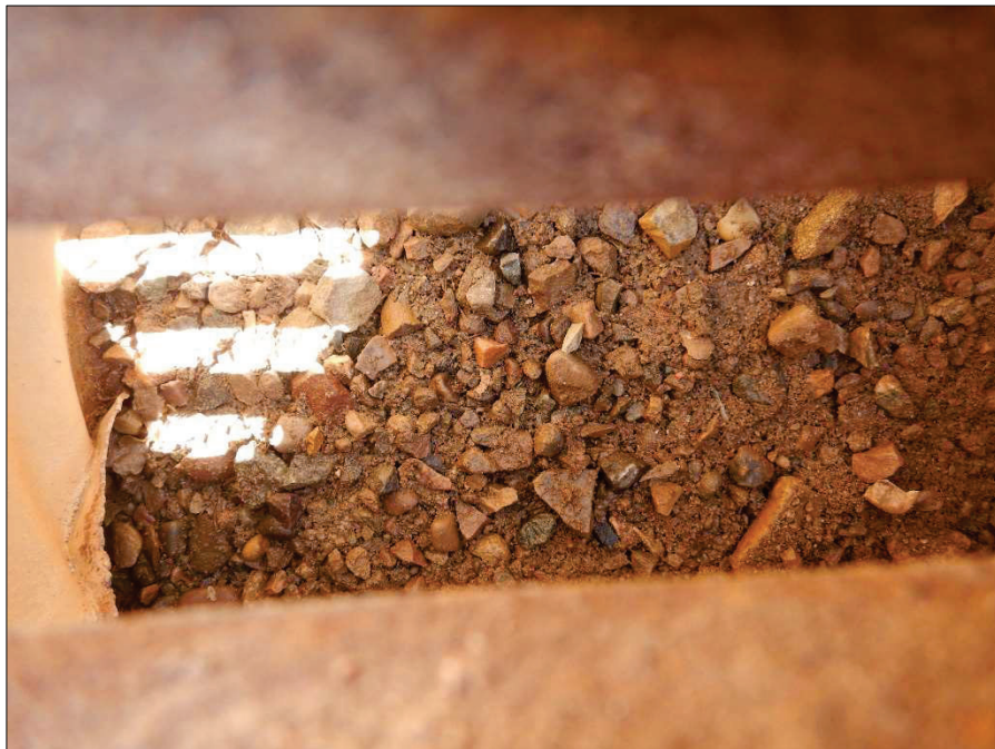
Photograph 80. Close-up view into catch basin in Drainage Area 1, as shown in Photograph 79. Note accumulated sediment and gravel.
