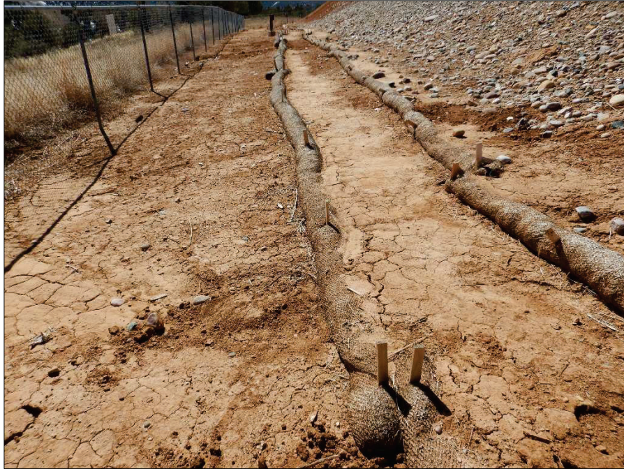
Photograph 111. Close-up view, facing Southwest, of straw wattles along southeastern side of South Evaporation Pond, as referenced in Photograph 110. Note deterioration of straw wattles and sediment accumulation against the wattles.
