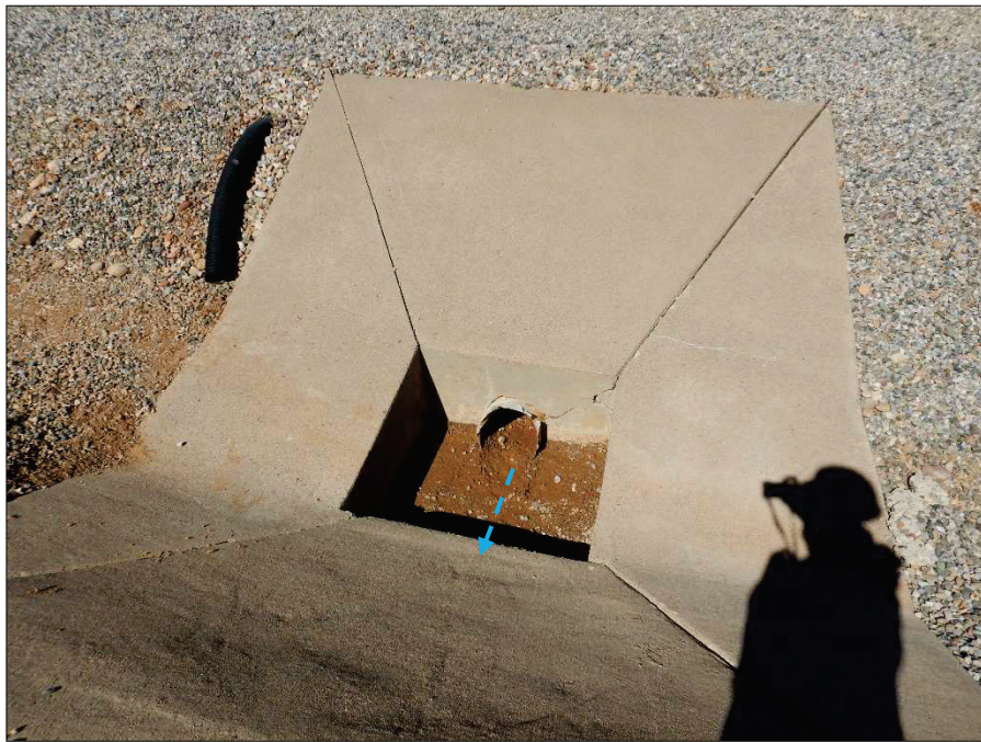
Photograph 48. View, facing North, of a drainage inlet flowing from Drainage Area 3 to the North Evaporation Stormwater Holding Pond. Note sediment accumulation.
