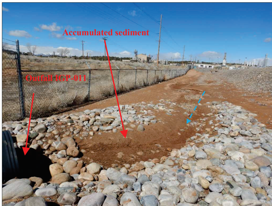
Photograph 102. View, facing North, of Outfall IGP-011. Note sediment accumulation.
