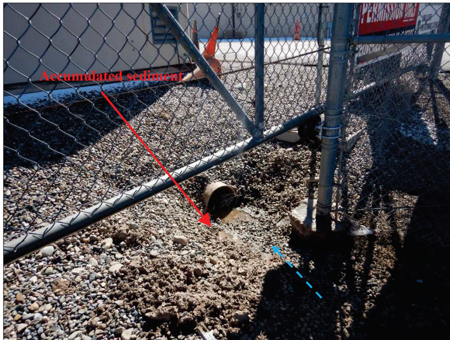
Photograph 69. Close-up view, facing Southeast, of culvert beneath main entrance road, connecting Gosney Pond to Drainage Area 8, as referenced in Photograph 68. Note sediment accumulation at the mouth of the pipe.
