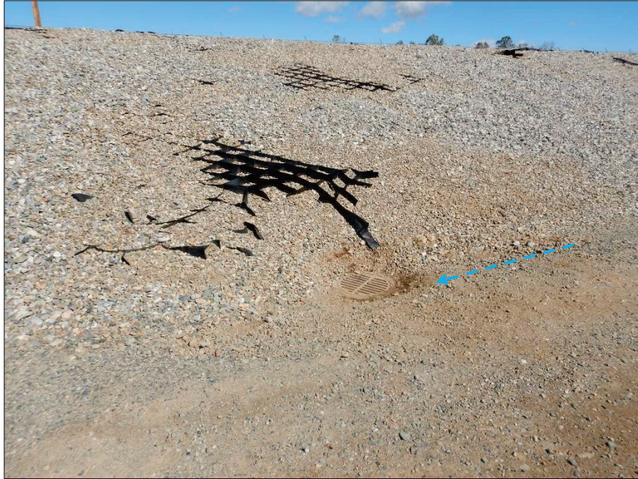
Photograph 79. View, facing Northeast, of an unprotected catch basin in Drainage Area 1. Note loose gravel and sediment near entrance of catch basin.
