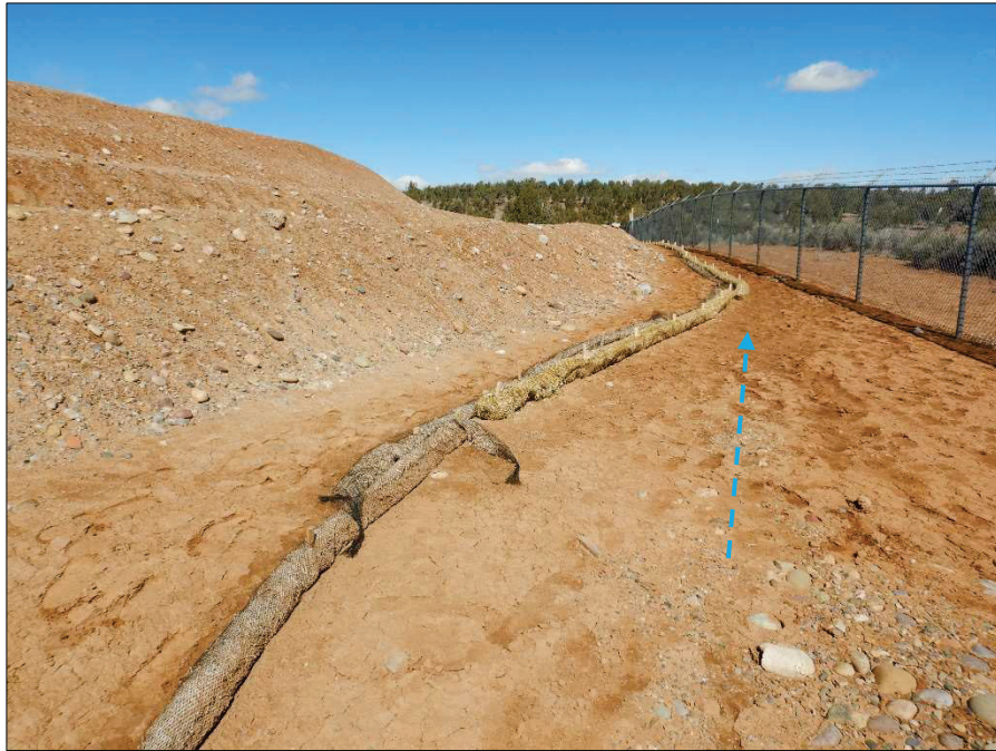
Photograph 105. View, facing North, of straw wattle along fence line in Drainage Area 15, downgradient from an unstabilized bank around the Soil Drying Containment Area. Note deterioration of the straw wattle and sediment accumulation against wattle barriers.
