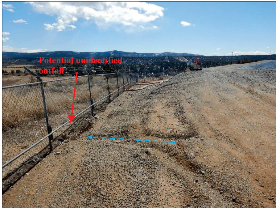
Photograph 22. View, facing South, of another potential unidentified outfall point in Drainage Area 14.
