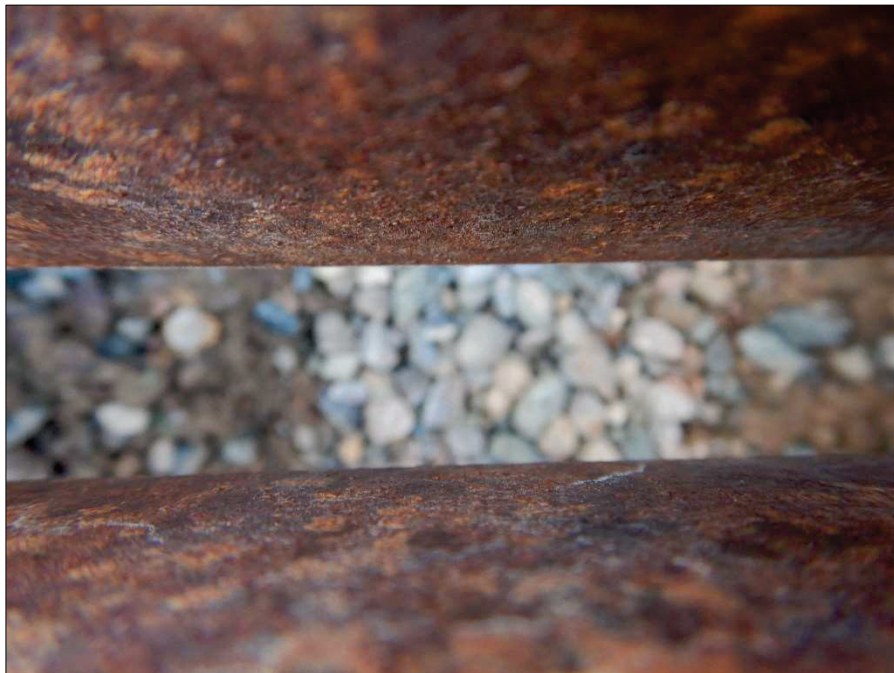
Photograph 78. Close-up view into catch basin in Drainage Area 2, as shown in Photograph 77. Note accumulated sediment and gravel.
