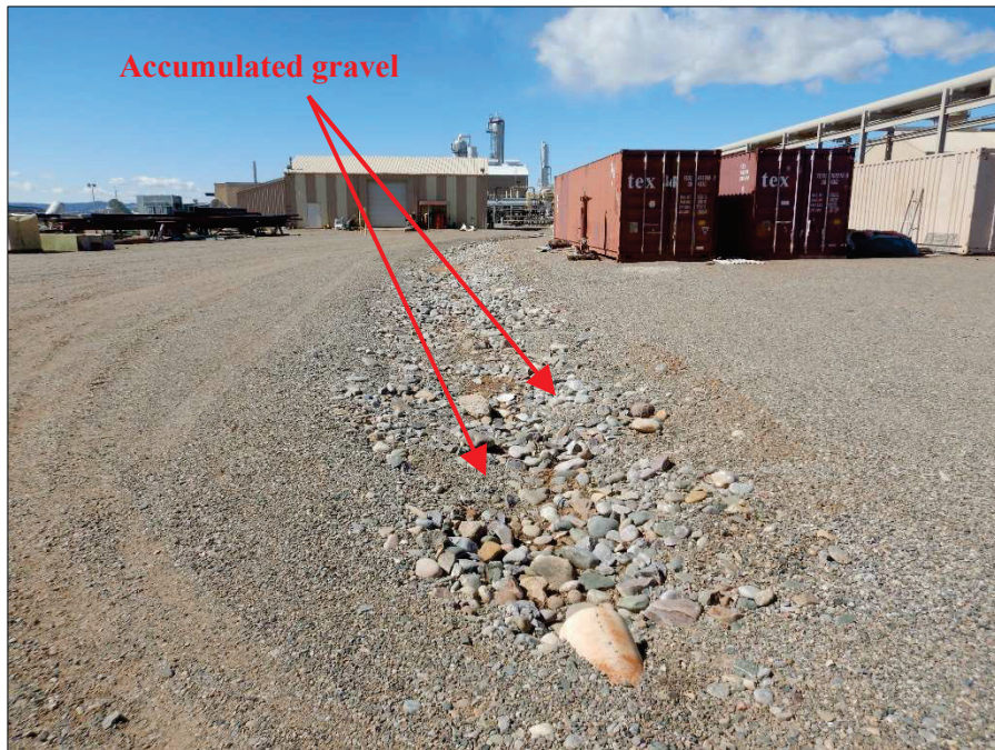
Photograph 101. View, facing West, of inlet of culvert into the Facility boneyard. Note accumulated gravel in the ditch upgradient from the culvert.
