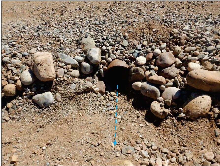
Photograph 83. View, facing south, of culvert in Drainage Area 15 that ultimately drains to Outfall IGP-003. Note accumulated sediment and gravel at the mouth of the pipe.
