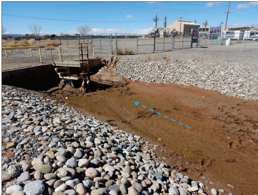
Photograph 54. Additional view, facing Northwest, of North Evaporation Stormwater Holding Pond, as referenced in Photograph 54. Note sediment accumulation in the pond.
