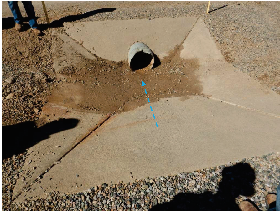
Photograph 61. Close-up view, facing West, of inlet of culvert connecting Drainage Area 1 to Gosney Pond, as referenced in Photograph 60. Note sediment accumulation.
