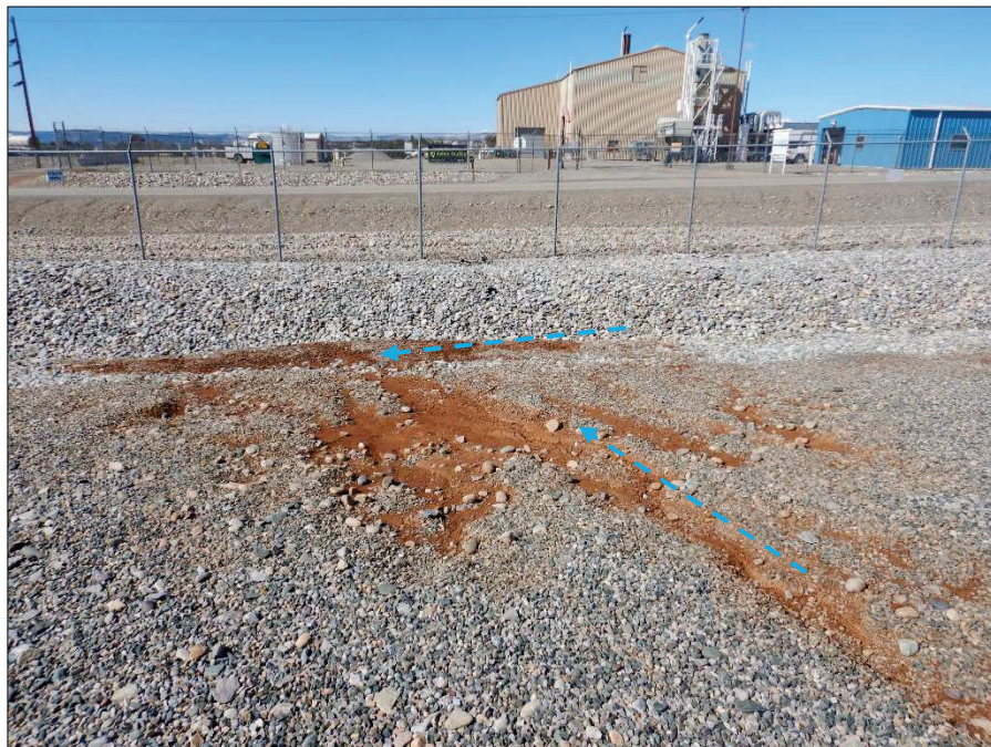
Photograph 38. View, facing West, of the bank of the ditch that drains into Gosney Pond. Note the rilling on the bank.
