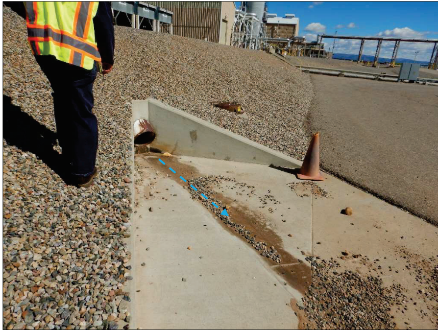
Photograph 49. View, facing Northeast, of the outlet pipe from the inlet shown in Photograph 48. From here, flow continues across the facility parking lot toward the North Evaporation Stormwater Holding Pond. Note sediment and gravel accumulation.
