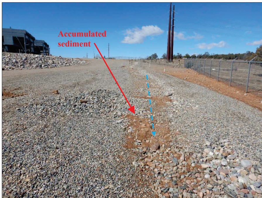
Photograph 74. Additional view, facing Northwest, of the ditch along Northeastern fence line in Drainage Area 15, as referenced in Photograph 73. Note accumulated sediment in the ditch.
