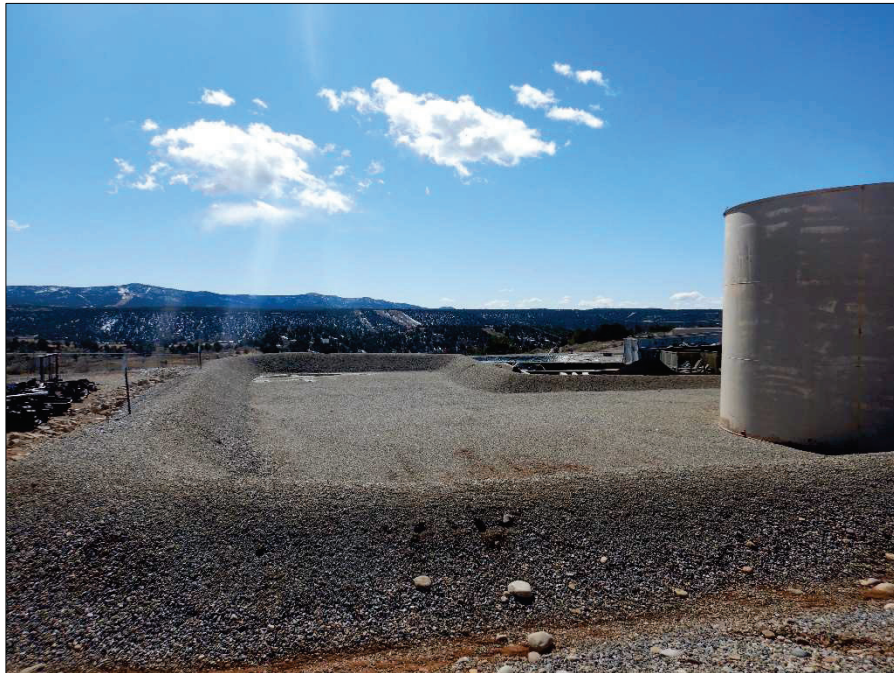
Photograph 6. View, facing South, of the secondary containment area for the above ground storage tanks, as referenced in Photograph 5.
