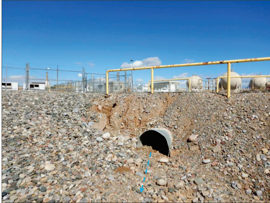
Photograph 57. View, facing Northeast, of the North Evaporation Stormwater Holding Pond discharge pipe. Note sediment and gravel accumulation in the pipe.
