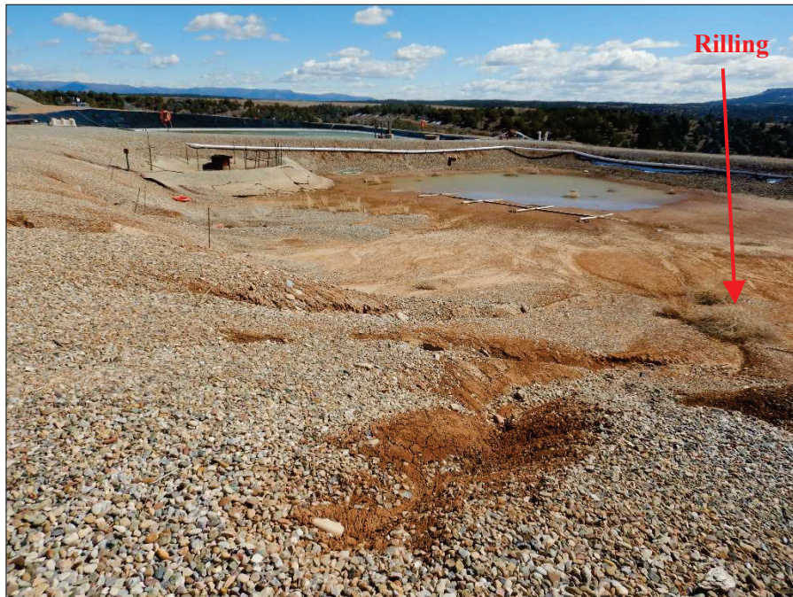
Photograph 42. Additional view, facing Southeast, of West Excess Pond, as referenced in Photographs 40 and 41. Note rilling on the pond bank.
