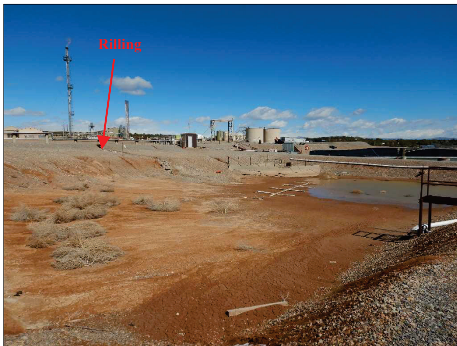
Photograph 40. View, facing North, of West Excess Pond. Note rilling on the pond bank.
