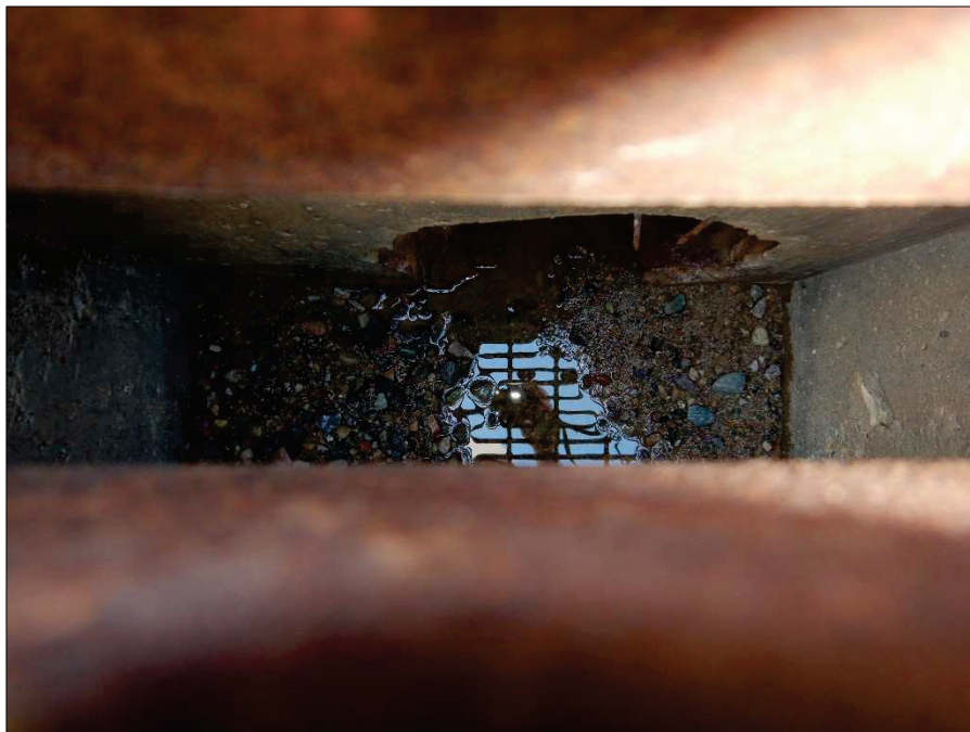
Photograph 76. Close-up view inside of catch basin in Drainage Area 1, as referenced in Photograph 75. Note accumulation of gravel and sediment.
