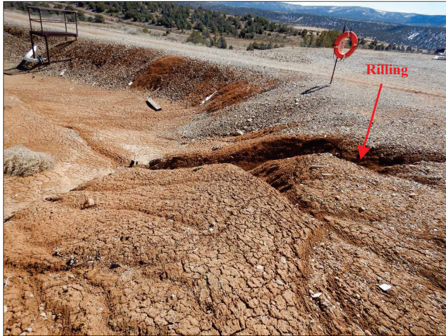
Photograph 41. Additional view, facing Southeast, of West Excess Pond, as referenced in Photograph 40. Note rilling on the pond bank.
