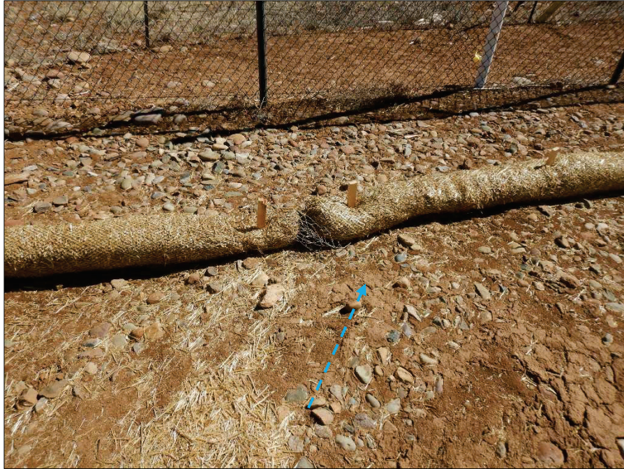
Photograph 109. Additional view, facing East, of new straw wattles near Outfall IGP-004, as referenced in Photograph 108. Note straw wattle segments are not overlapping, creating gaps.
