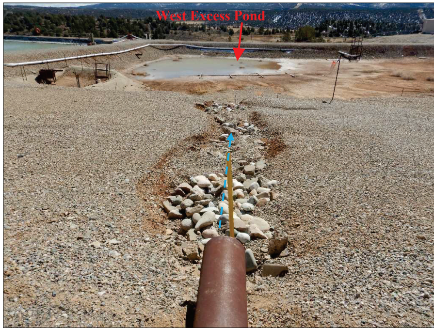
Photograph 45. View, facing South, of outlet of culvert leading to West Excess Pond. Note evidence of erosion.
