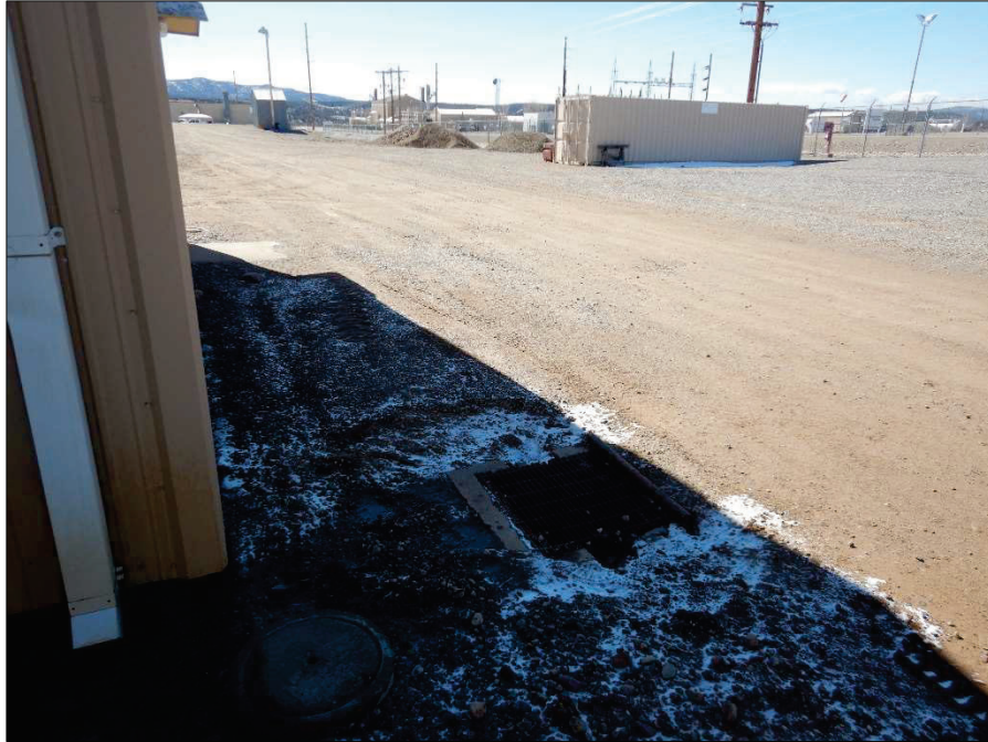
Photograph 75. View, facing Southwest, of an unprotected catch basin in Drainage Area 1. Note loose gravel and sediment near catch basin grate.
