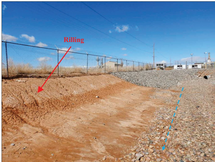
Photograph 43. View, facing North, of bank of the ditch leading to Outfall IGP-011. Note rilling on the unstabilized bank.
