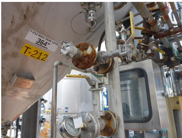
Photo 26: Severe corrosion on tags and ancillary equipment associated with Tank 212. Corrosion caused the tags to be illegible.
