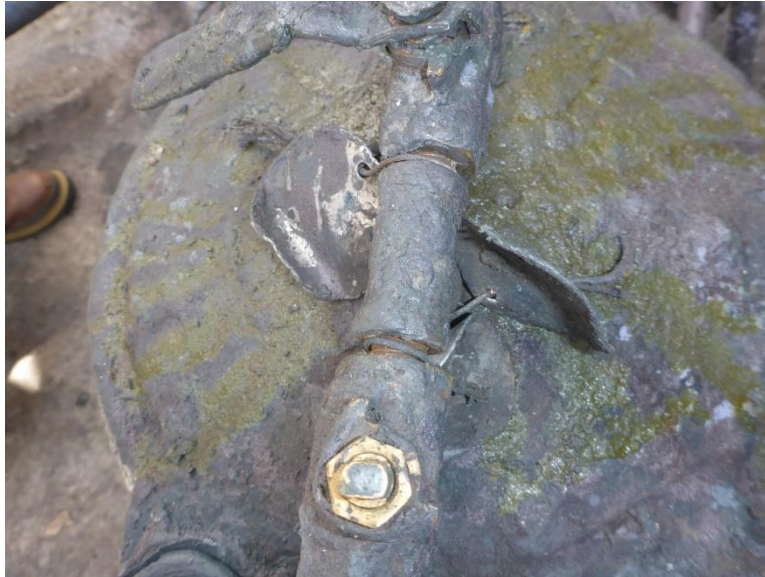
Photo 15: Three illegible tags on top of a filter house associated with the BP tank farm in SA-7.
