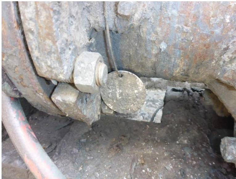
Photo 16: Illegible tag located between a filter and pump associated with the BP tank farm in SA-7.
