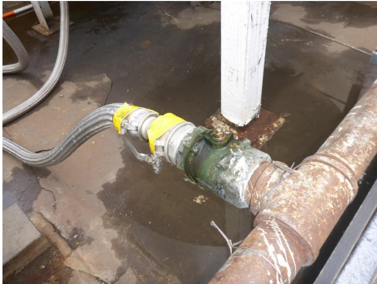
Photo 22: Liquid at the connection identified with tag number 583.
