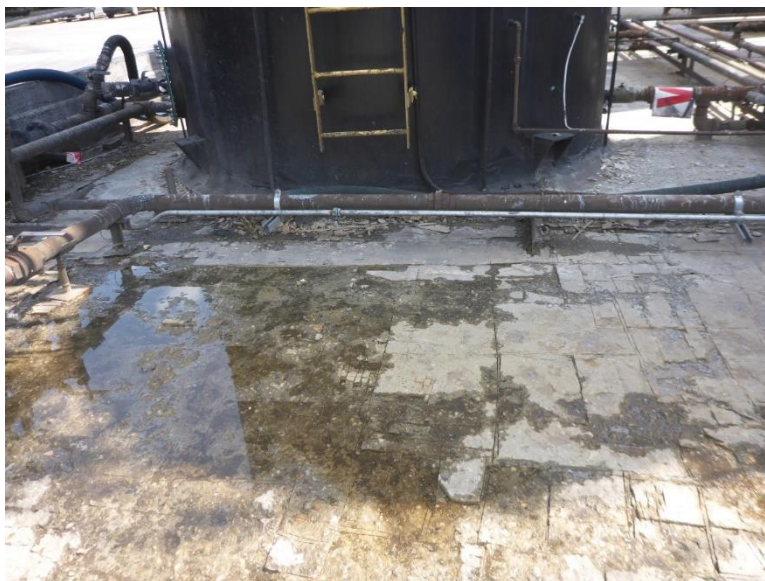
Photo 17: Significant cracks, peeled and missing coating in the secondary containment of SA-2.
