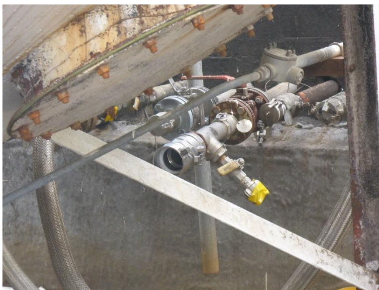
Photo 20: Open ended line at the cam-lock fitting that was identified with tag number 572.
