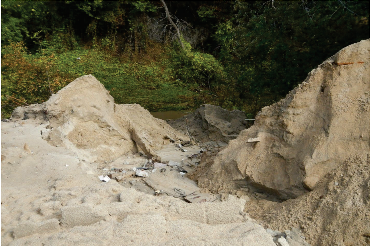
Photo 17, significant erosion caused process material to enter the South Papillion Creek
