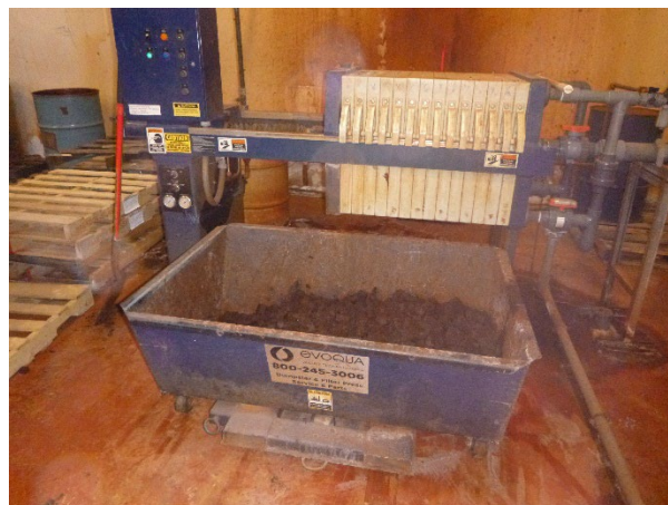
Photograph 16: WWT Filter Press
