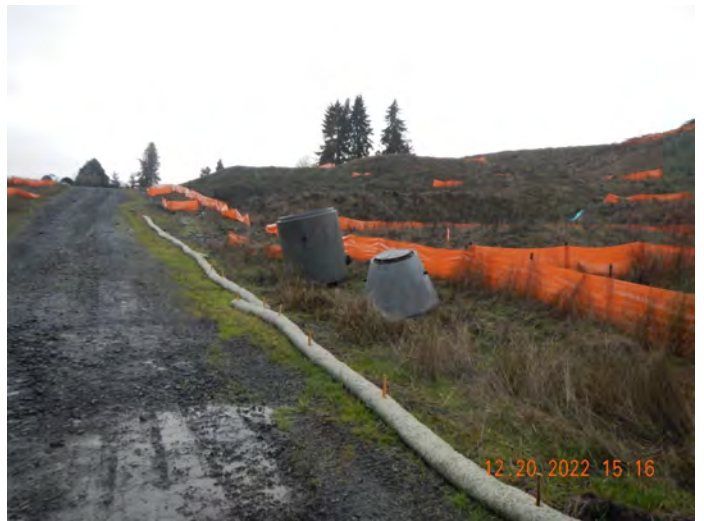
Photo #:20 (DSC3147) Description: Facing south/southwest, photo of BMPs along the North Pond access road.
