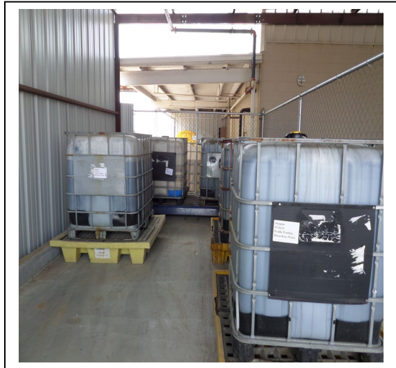
Hager. Acid and Alkaline Hazardous Waste Storage Area – 90-Day. Inspector observed five 275-gallon totes, closed, labeled with the words hazardous waste, pending analysis. Photograph 10 taken at 10:52 a.m.
