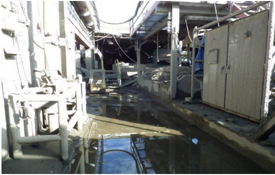
Figure 79: HTL. OKP. WWT. Observed wastewater, waste solids and sludge on floor. 4:03 pm.
