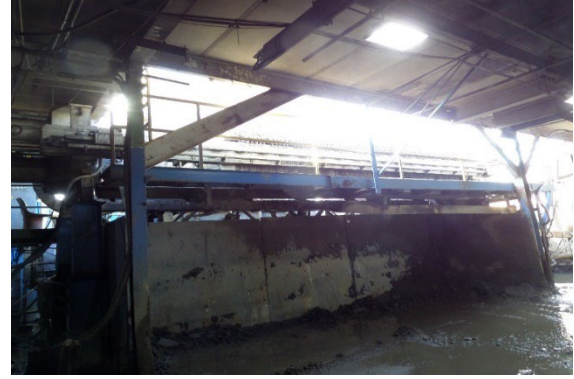
Figure 80: HTL. OKP. WWT. View of the Filter Press. Observed waste solids and wastewater on floor under the filter press. 4:04 pm.
