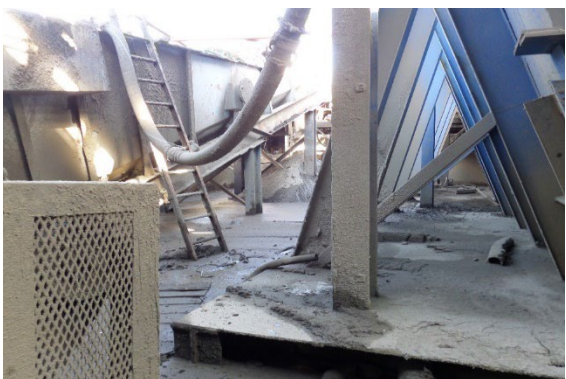
Figure 77: HTL. OKP. WWT. WWT. Observed wastewater, waste solids and sludge on floor. 3:58 pm.
