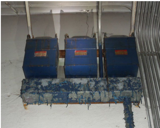
Figure 59: HTL. Old Keebler Plant Basement. Possible capacitors or transformers. 12:17 pm.
