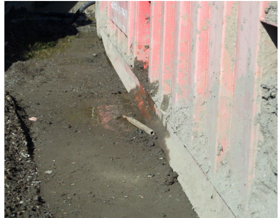
Figure 60: HTL. Culvert Next to Bunkers. Observed water released from roll-off container to concrete culvert next to right Bunker 3:04 pm. View North.
