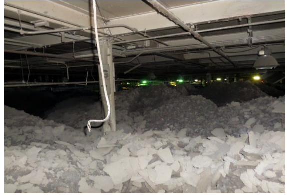
Figure 62: HTL. OKP. Old Keebler Plant. Observed Pile extends from Column C to I & Rows 5 to 9. 3:18 pm.
