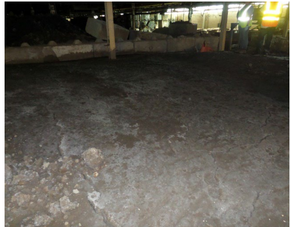
Figure 72: HTL. OKP. Observed a washed-out & dried area of the Pile between Columns B14 to B15 3:39 pm.
