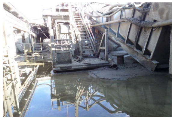
Figure 76: HTL. OKP. Wastewater treatment (WWT). Observed wastewater, waste solids and sludge on floor of screw area. 3:58 pm.
