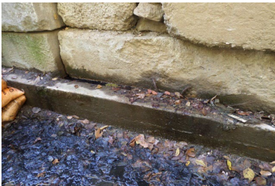
Figure 35: HTL. Bunkers. Observed liquid between Bunker Mafia Blocks along concrete culvert. Behind Bunkers 11:26 am.
