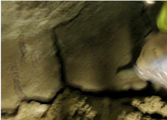
Figure 85: HTL. OKP. Observed washed-out and dried area of Pile. 5:15 pm.
