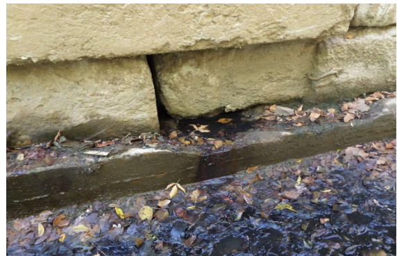
Figure 36: HTL. Bunkers. Observed water between Bunker Mafia Blocks along concrete culvert. Behind Bunkers 11:26 am.
