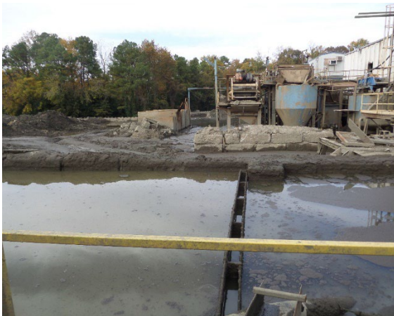
Figure 83: HTL. OKP. WWT. View of Jig Pad. Observed Jig Pad full of water adjacent to possible filter cake/waste solids. 4:28 pm.
