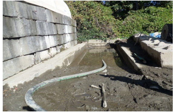
Figure 32: HTL. Bunkers. Observed wastewater accumulated in concrete culvert next to right Bunker 11:20 am. View North.
