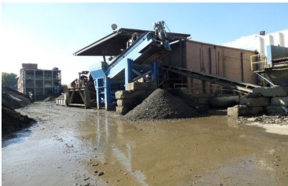
Figure 39: HTL. Adjacent Old Keebler Plant. Stopped sampling of New FVS lights. Generation of New FVS heavies stopped about 11:31 am. View South.
