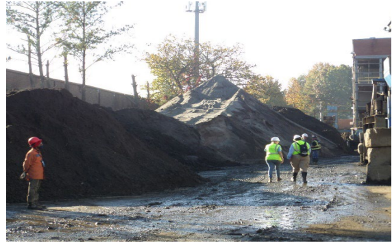
Figure 8: HTL. Adjacent Old Keebler Plant. Observed an assortment of comingled waste piles with sand on ground adjacent to TAV processing area 9:52 am. View South.
