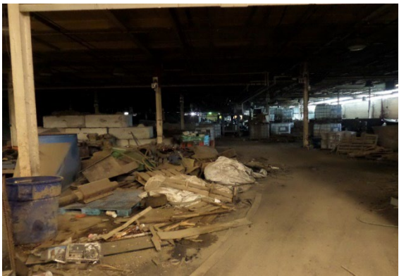
Figure 75: HTL. OKP. Observed unknown materials, process equipment and trash on backside of the Pile adjacent to columns A15 to H15. 3:50 pm.
