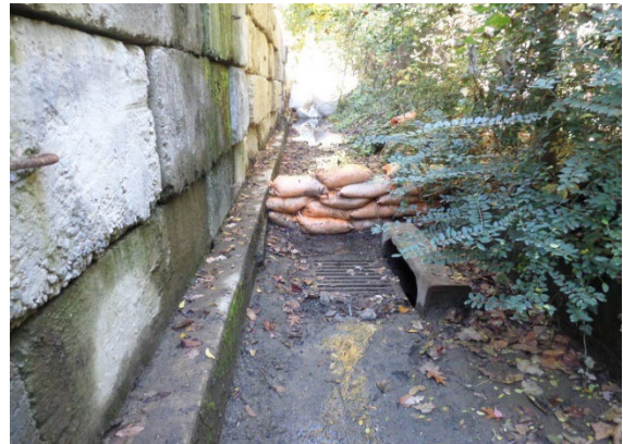
Figure 34: HTL. Bunkers. Observed concrete culvert was wet behind Bunkers. Observed drain. appeared wet 11:24 am. View Northwest.
