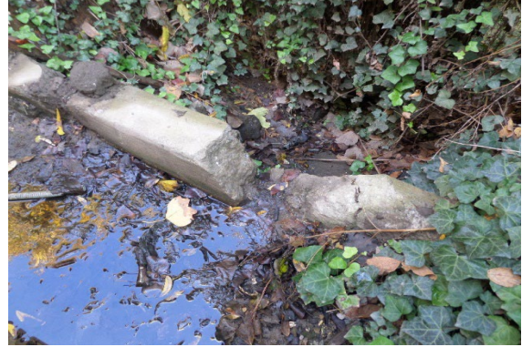
Figure 38: HTL. Bunkers. Observed concrete culvert and drain had water behind Bunkers. Observed concrete berm was breached and drains to outfall downhill to woods near Access Road Area. 11:27 am.
