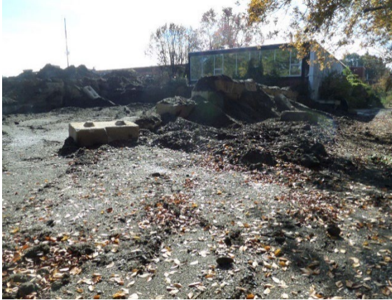
Figure 43: HTL. Northwest Corner Old Keebler Plant (NWOKP). Remaining ASR in storage area, 11:41 am. View West.
