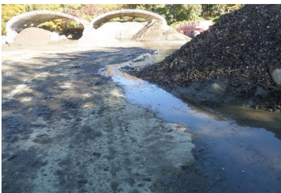
Figure 29: HTL. Bunkers. Observed stream of wastewater flowing down gradient towards Bunkers 11:17 am. View North.
