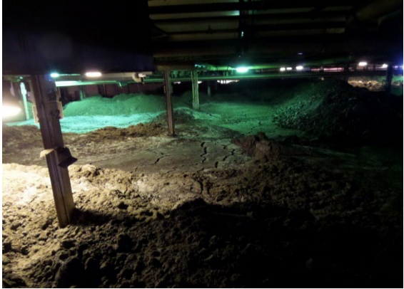
Figure 73: HTL. OKP. Observed washed-out area of the Pile from columns B9 to B12 and columns C9 to C12. 3:41 pm.
