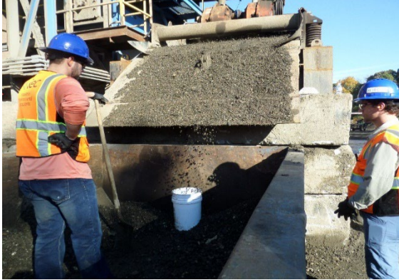
Figure 19: HTL. Adjacent Old Keebler Plant. Observed sampling of new FVS lights into 5-gallon container at from new FVS process. 10:16 am.
