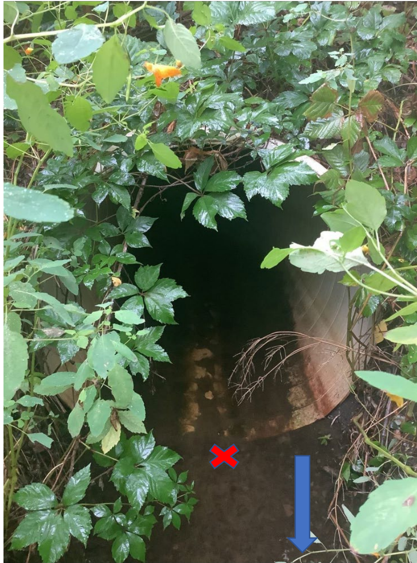
Cedar: A white PVC outfall located on the south side of the Cedar View Nursing Home. Flow direction indicated by a blue arrow. Sample point indicated by a red “X”.
