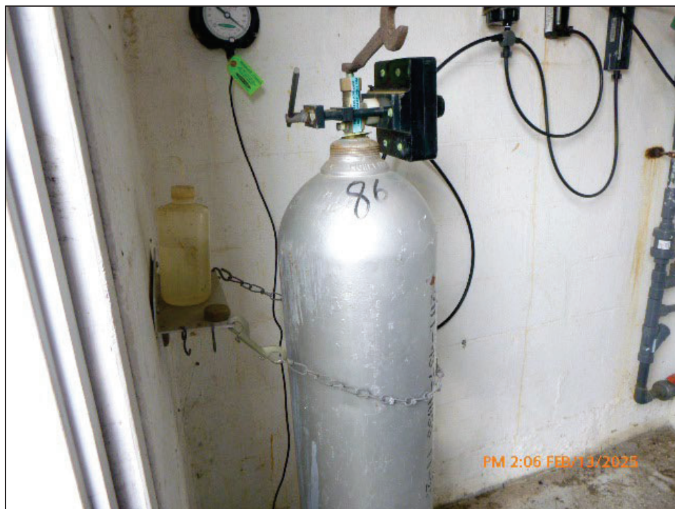
Photograph 26. 2/13/2025 2:06 pm P1010281.JPG Description: Plant #2. Partially-full chlorine gas cylinder.
