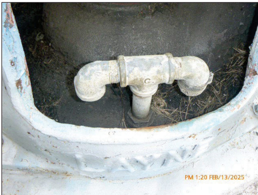
Photograph 16. 2/13/2025 1:20 pm P1010251.JPG Description: Plant #1. Well #3 vent with missing screen.
