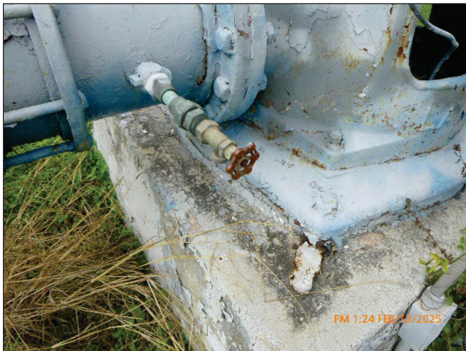
Photograph 15. 2/13/2025 1:24 pm P1010252.JPG Description: Plant #1. Well #3 with raw water threaded sample tap.
