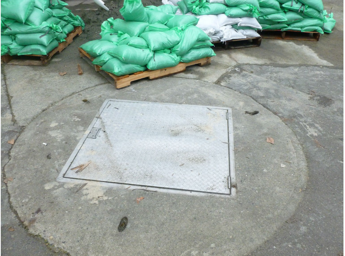
Photo 5 / P1010202 – Lift Station, Southwest Side of Site
