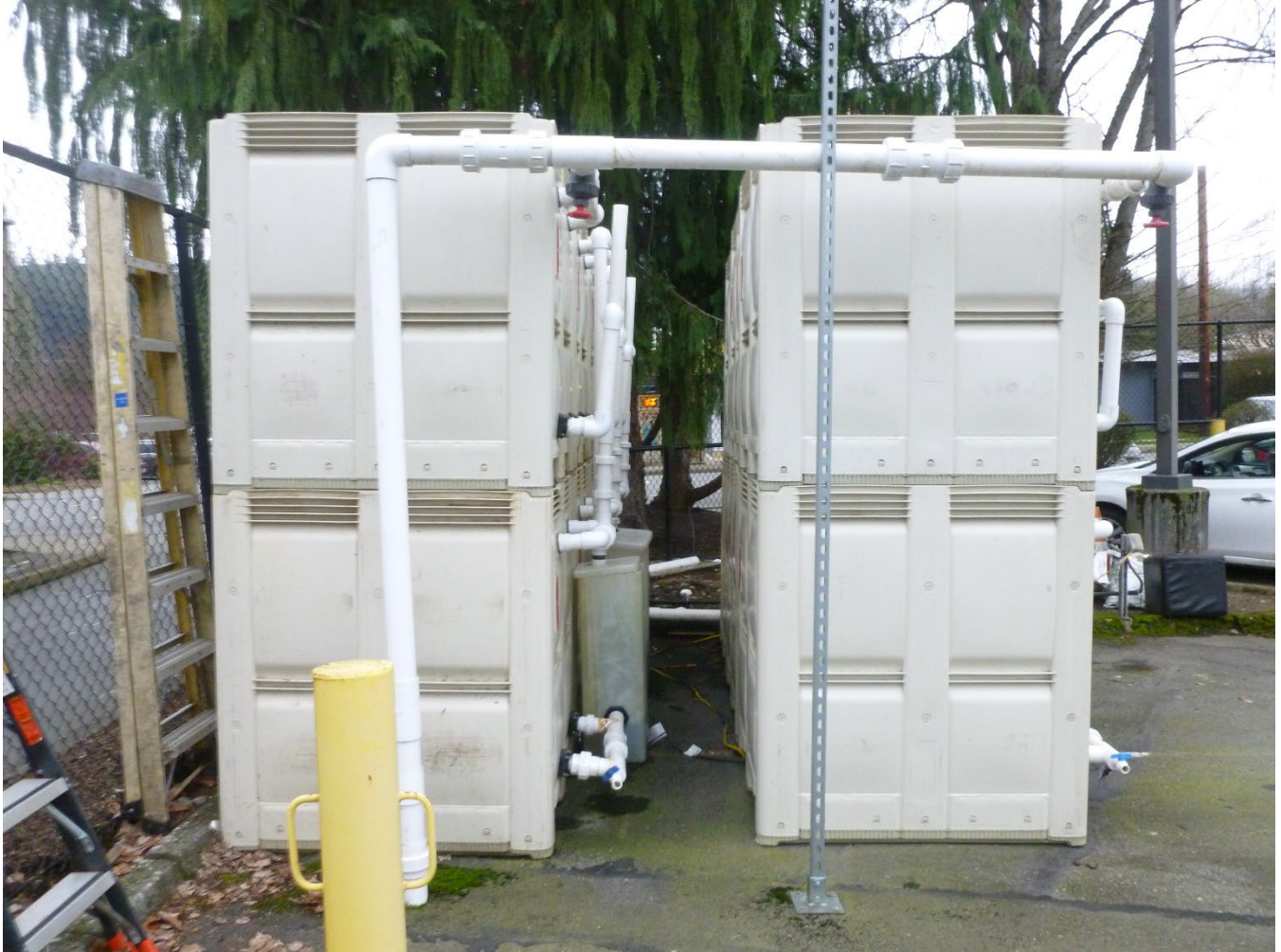
Photo 9 / P1010206 – Filtration System, west end
