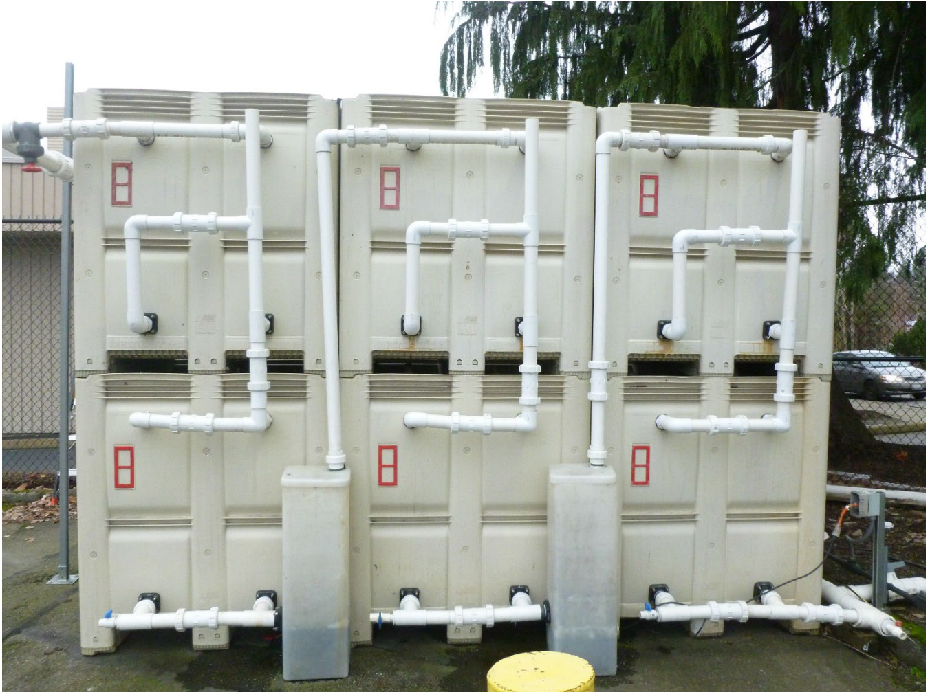
Photo 10 / P1010207 – Filtration System, south side
