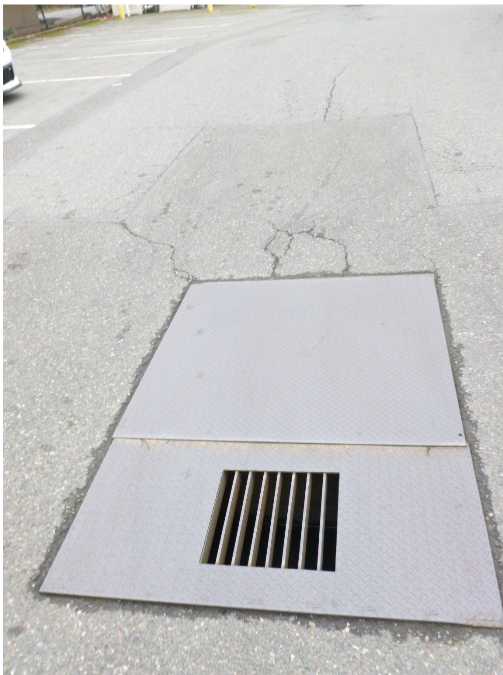
Photo 8 / P1010205 – Oil/Water Separator
