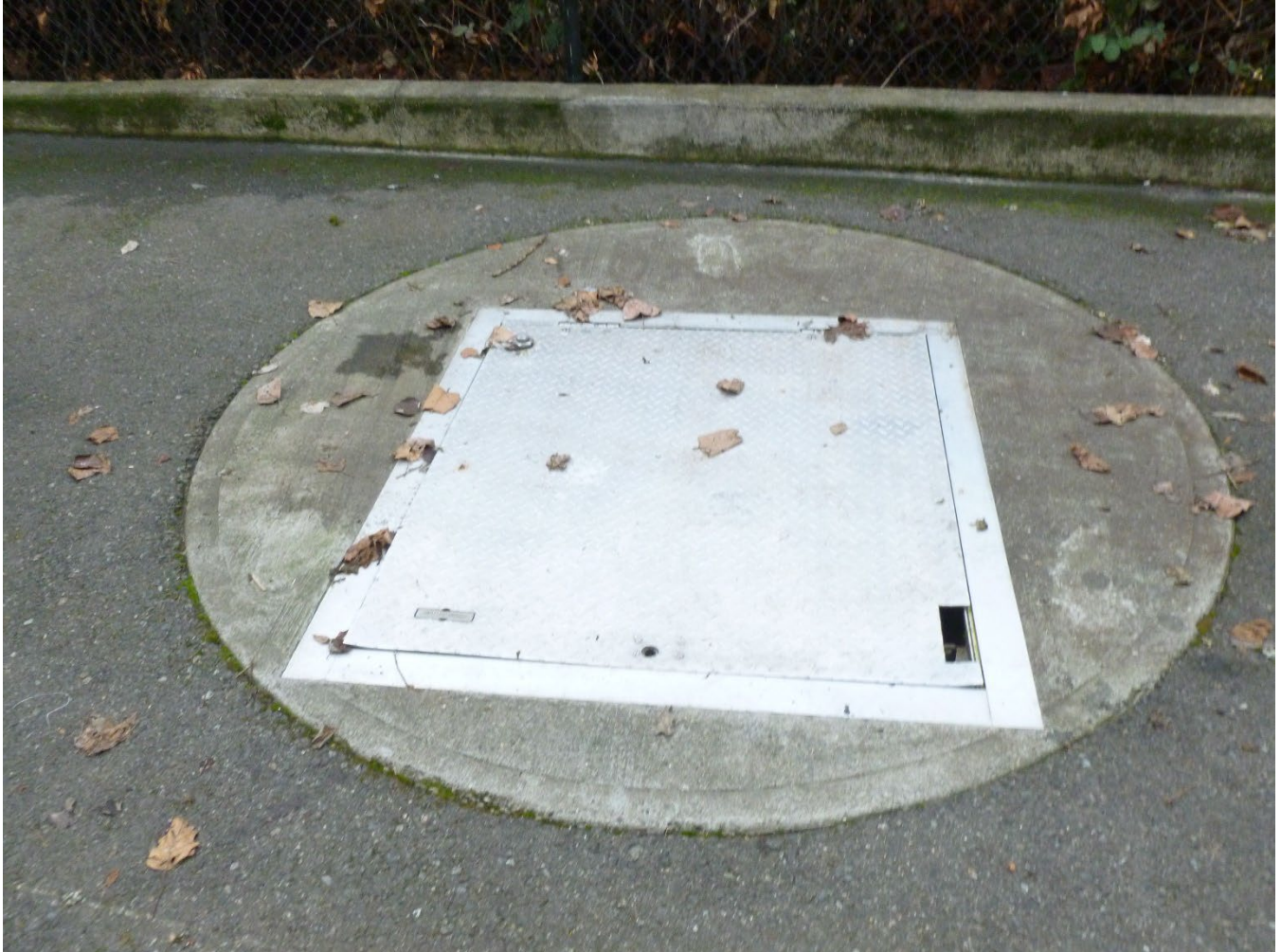
Photo 6 / P1010203 – Lift Station, facing west
