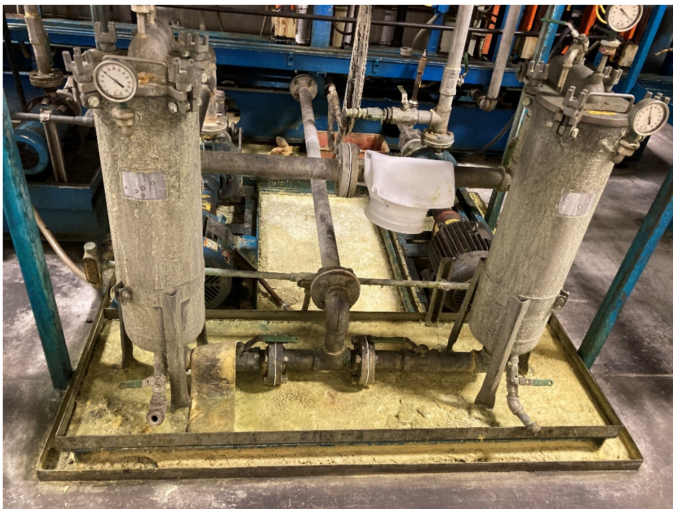
Photo #1 – Yellow dried debris under the washing filtration system.
