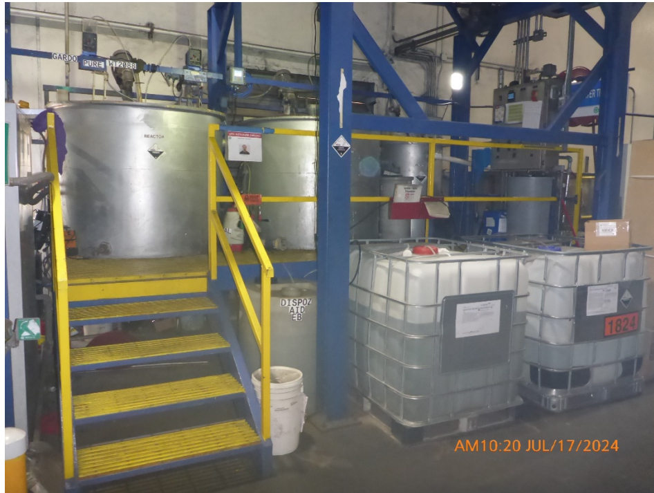
Photograph 3: Current wastewater pretreatment area inside the building.
