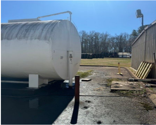
Photo-41 Oily Debris on the West Side
