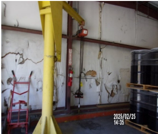
Photo-19 Insulation in Disrepair (Permitted Storage Area)
