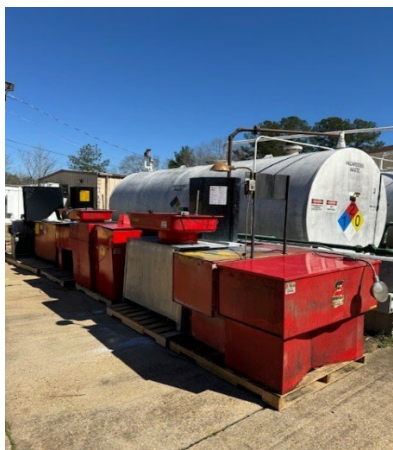
Photo-31 Used Parts Washer Station
