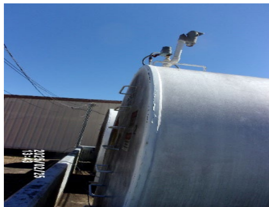
Photo-24 Tank #1 Coating Peeling
