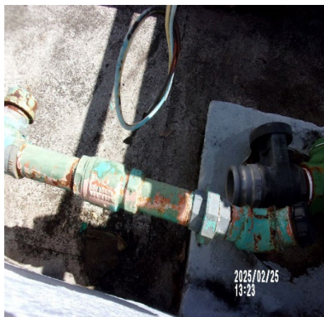
Photo-26 paint peeling and signs of rust
