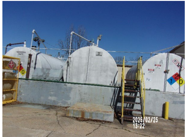
Photo-22 Hazardous Waste Tank Farm
