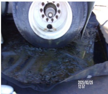
Photo-3 Oily Debris in Secondary Containment
