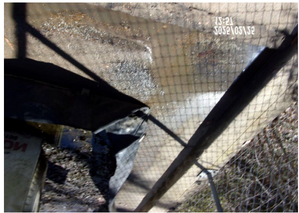
Photo-4 Sec. Containment in Disrepair
