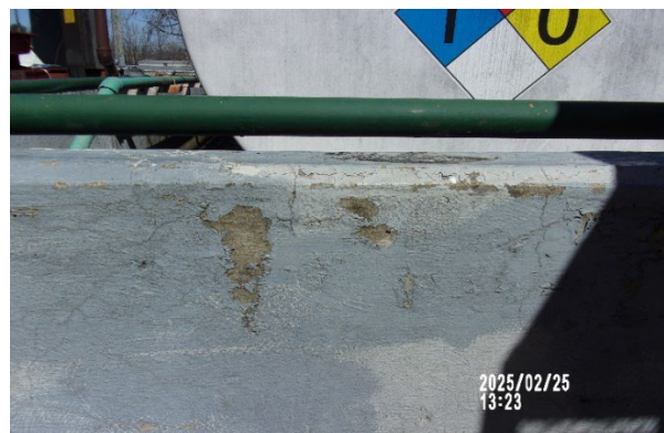
Photo-30 Cracked Secondary Containment
