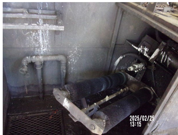
Photo-33 Drum Washer/Wet Dumpster
