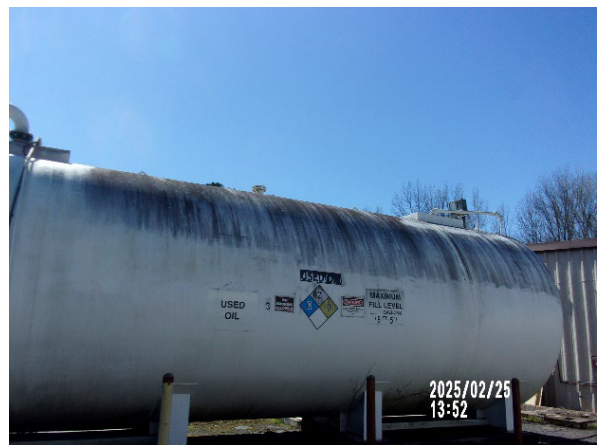
Photo-38 20,000-gallon Used Oil Tank
