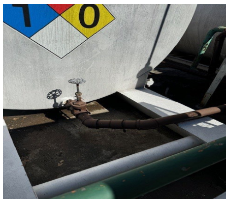
Photo-27 Signs of Rust on the Tank Valve
