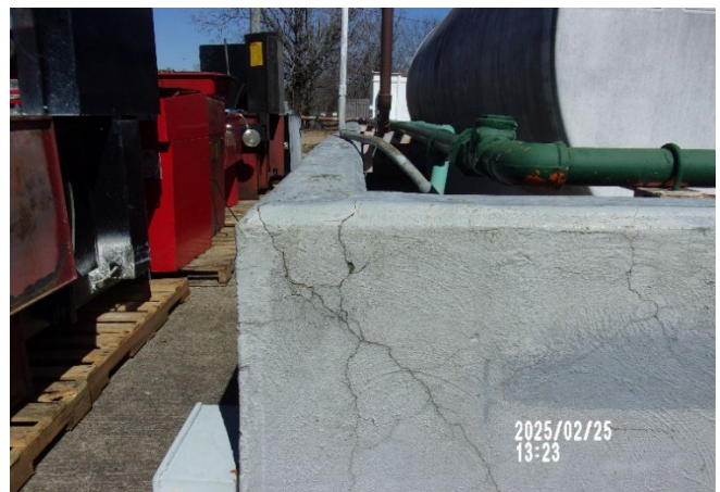
Photo-29 Cracked Secondary Containment
