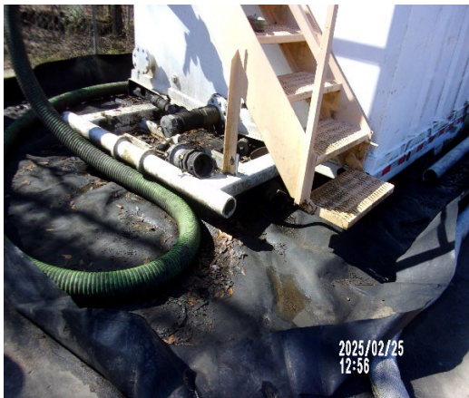
Photo-2 Secondary Containment in Disrepair
