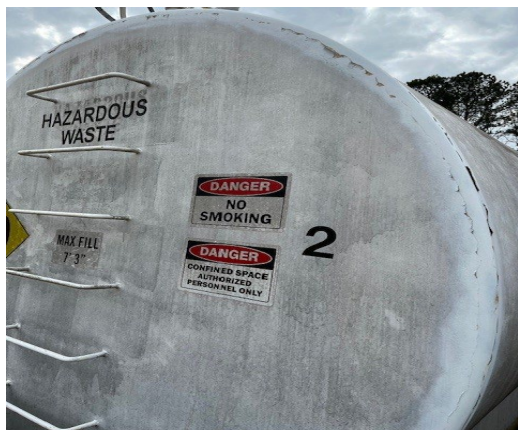
Photo-25 Tank #1 Coating Peeling
