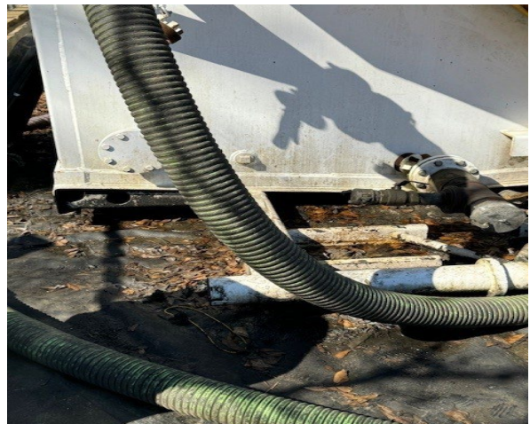
Photo-5 Debris in Secondary Containment
