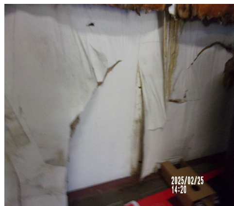
Photo-18 Insulation in disrepair (Permitted Storage Area)
