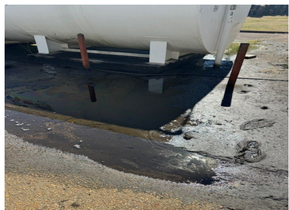
Photo-40 Stormwater Puddle with Oily Sheen
