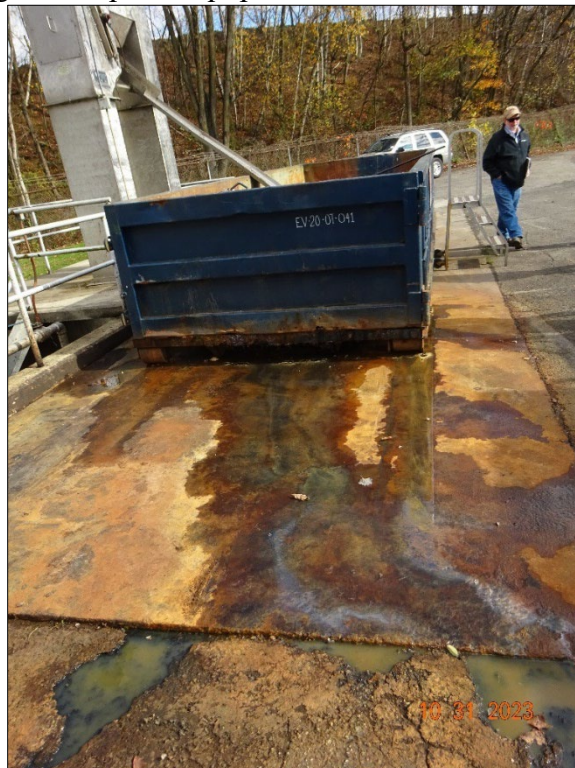
Photograph 4. DSC04748.JPG Description: Dumpster for grit and bar screen tailings.
