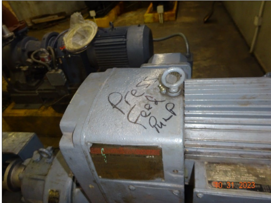
Photograph 19. DSC04848.JPG Description: Feed pump to the sludge press.
