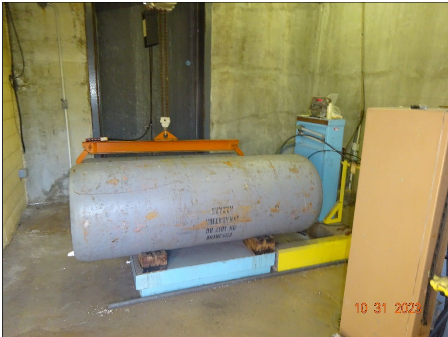
Photograph 22. DSC04815.JPG Description: 1 ton chlorine gas storage tank.
