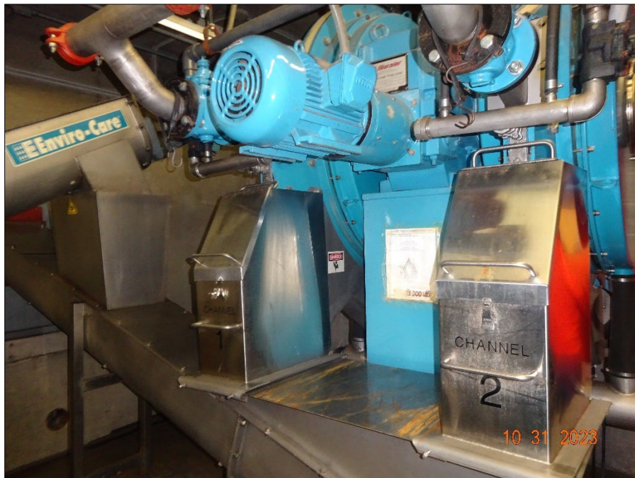
Photograph 18. DSC04828.JPG Description: Sludge press, currently offline.
