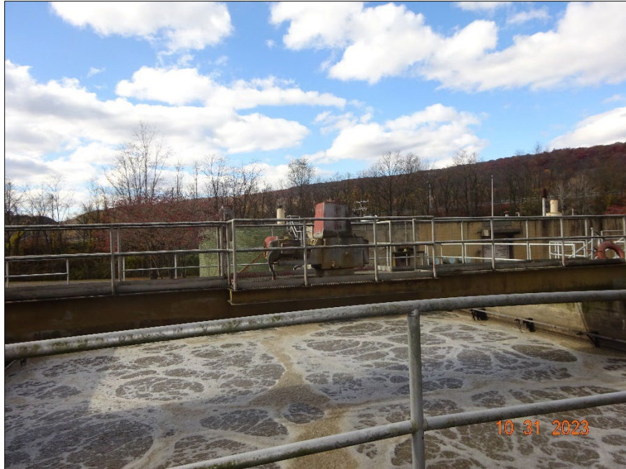
Photograph 13. DSC04781.JPG Description: Aeration Basin 1, online and operational.
