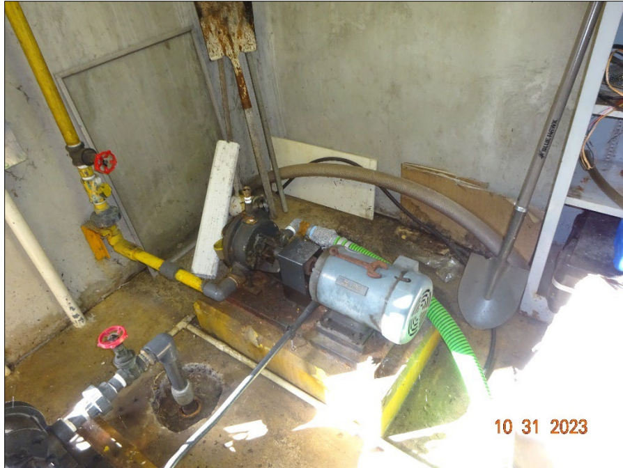
Photograph 25. DSC04804.JPG Description: Effluent sample withdraw pump.
