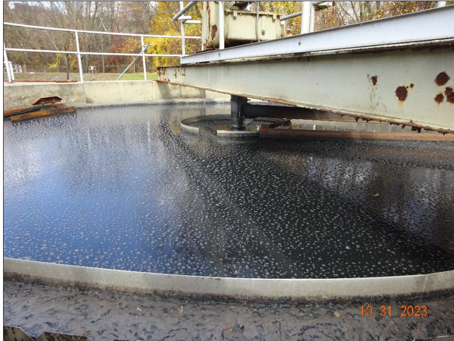
Photograph 17. DSC04774.JPG Description: Sludge Thickener, currently offline.
