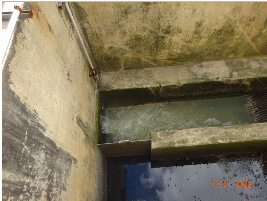
Photograph 2. DSC04743.JPG Description: Influent channel sampling point and bar screen.
