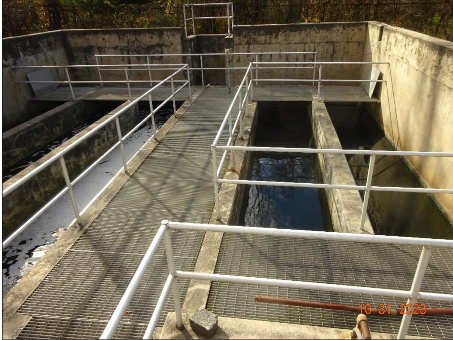
Photograph 21. DSC04802.JPG Description: Chlorine Contact Basin.
