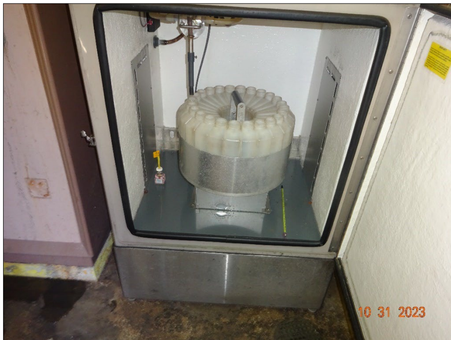
Photograph 28. DSC04807.JPG Description: Effluent Composite Sampler.
