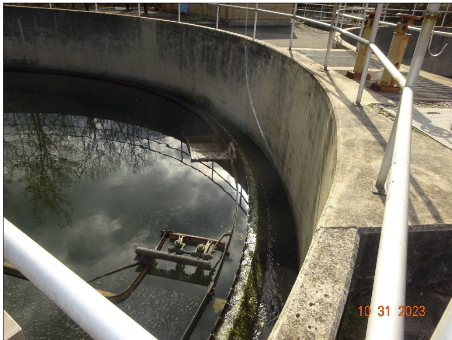
Photograph 20. DSC04789.JPG Description: Secondary Clarifier 1, online and operational.
