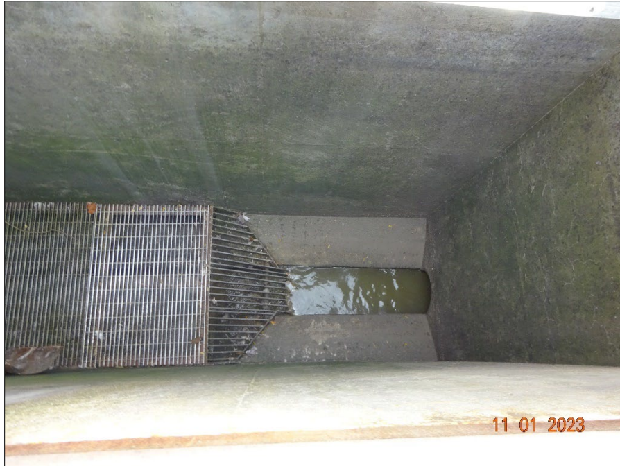
Photograph 35. DSC04874.JPG Description: Pump Station 1 Bar screen.
