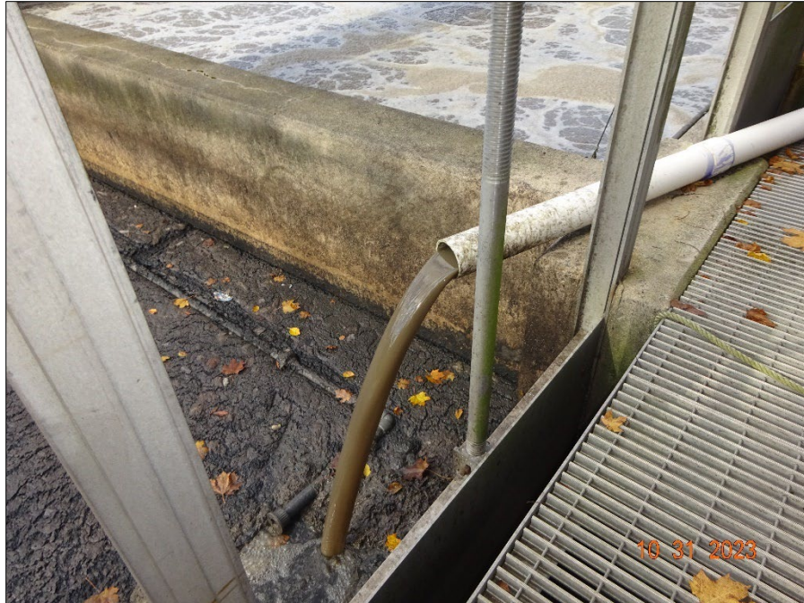
Photograph 15. DSC04782.JPG Description: WAS line draining into Aeration Basin 2.
