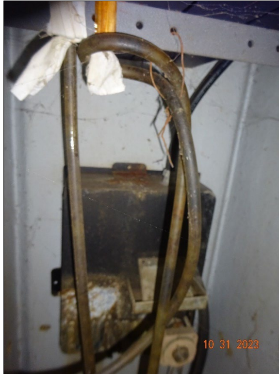
Photograph 27. DSC04811.JPG Description: Fouled effluent composite sample line.
