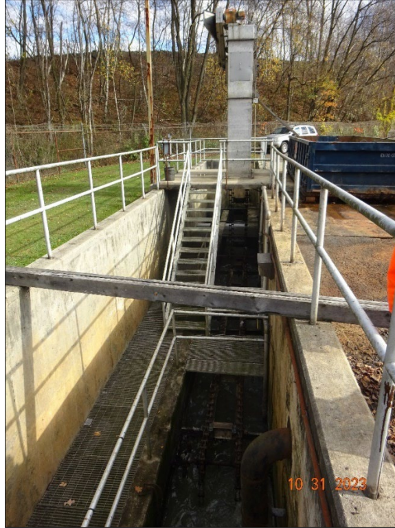
Photograph 3. DSC04752.JPG Description: Grit handling and disposal equipment.
