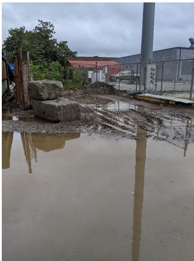
Figure 86: PXL_20211006_152333693.jpg – Plugged up Stormwater drain
