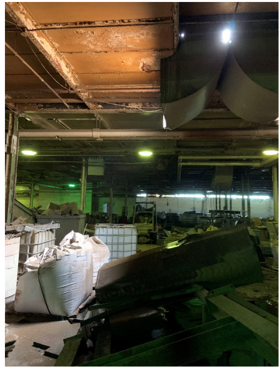
Figure 38: IMG_3107.jpg– Keebler Building showing holes in roof
