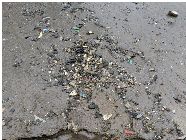
Figure 107: PXL_20211006_181815901.jpg – Settling Sludge from Stormwater Runoff in Outfall 3
