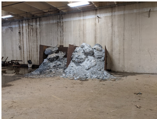
Figure 94: PXL_20211006_180547574.jpg – Partially melted aluminum in the Basement
