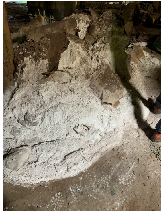
Figure 30: IMG_3099.jpg – Pile of quick lime in the Keebler building
