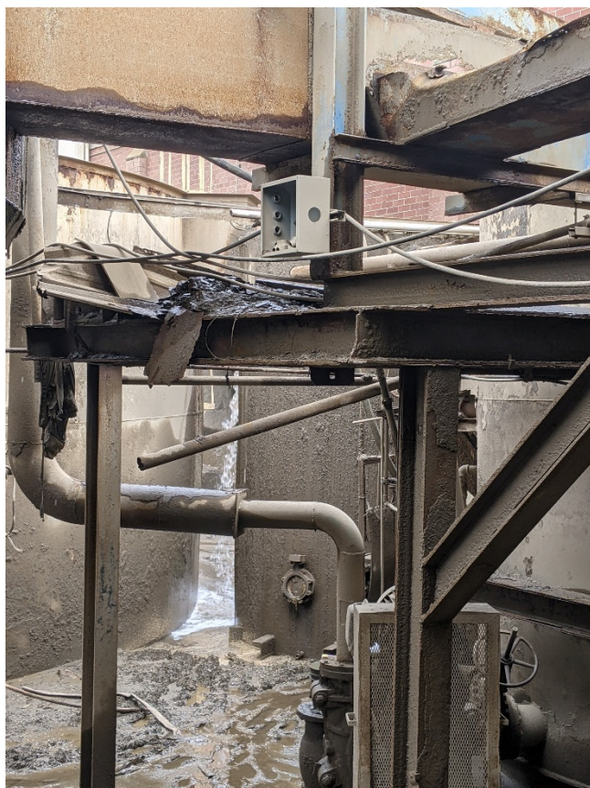
Figure 77: PXL_20211006_151059043.MP.jpg – Process water overflowing from Wastewater Treatment Area tanks
