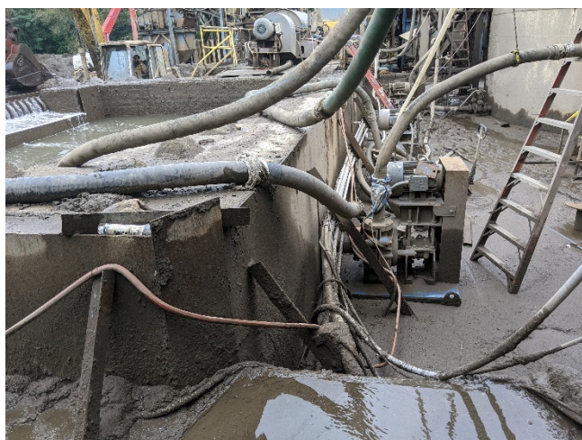
Figure 67: PXL_20211006_150035330.jpg – Wastewater treatment area
