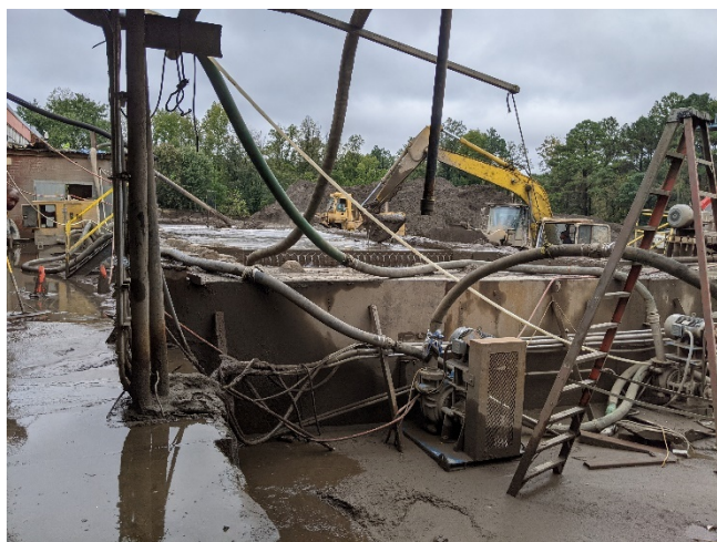
Figure 73: PXL_20211006_151020218.jpg – Wastewater Treatment Area
