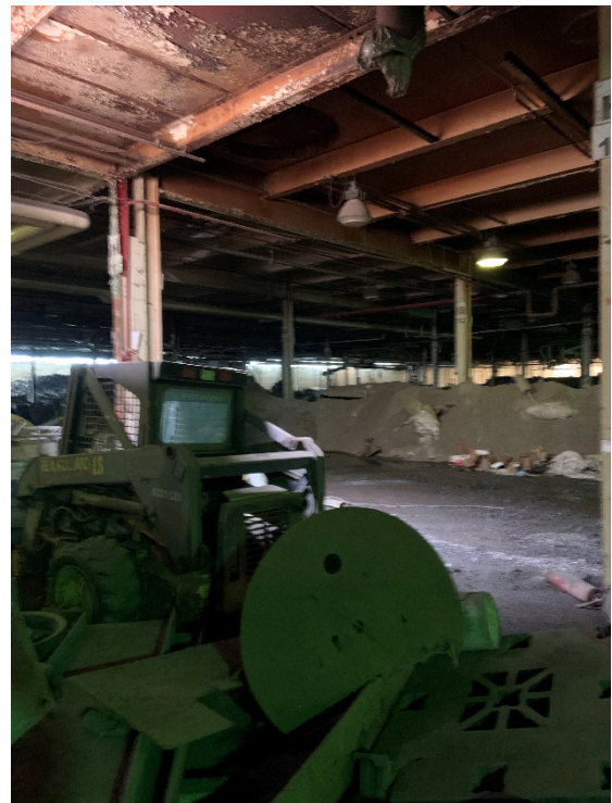
Figure 36: IMG_3105.jpg – Piles of solid waste stored in the Keebler Building
