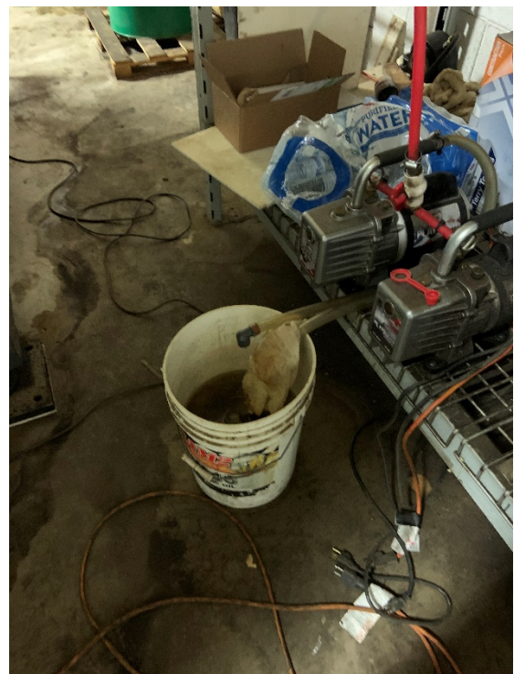
Figure 4: IMG_3073.jpg – Pump oil in a bucket in the Shipping Building
