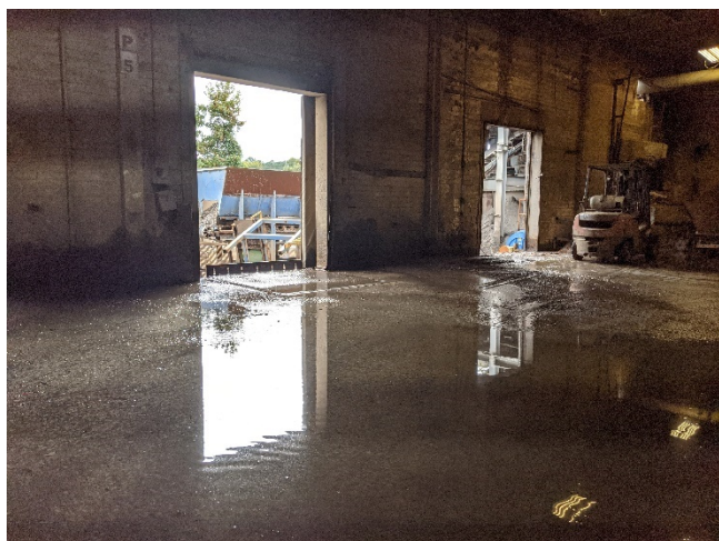
Figure 57: PXL_20211006_143449364.jpg – Process wastewater leaving the building
