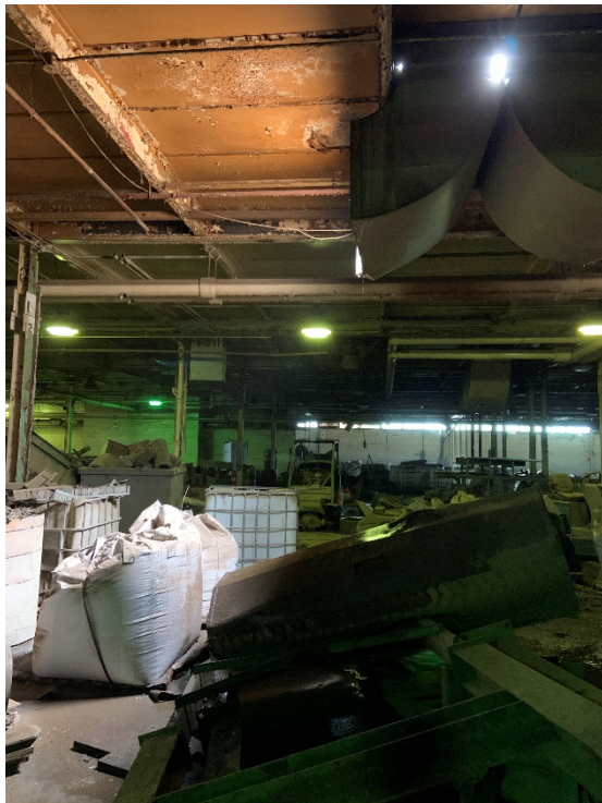
Figure 39: IMG_3108.jpg - Containers of unknown waste in the Keebler Building
