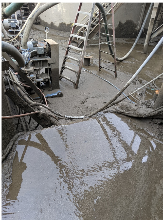
Figure 66: PXL_20211006_145946590.jpg – Process wastewater and sludge flowing from the process onto the ground in the wastewater treatment area
