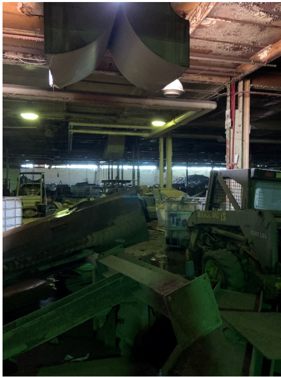
Figure 37: IMG_3106.jpg – Keebler Building showing holes in roof
