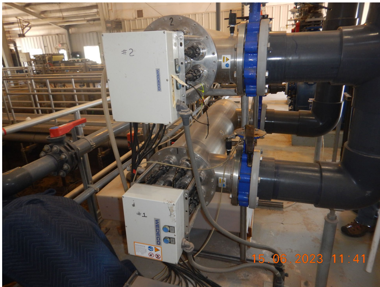
Picture of the two (2) bank Ultraviolet (UV) effluent disinfection configuration prior to discharge at Outfall 001 into the San Felipe Eastside Ditch (depicted in Aerial Image #1 above). (DSCN 2596). Photographed by D. Esparza.
