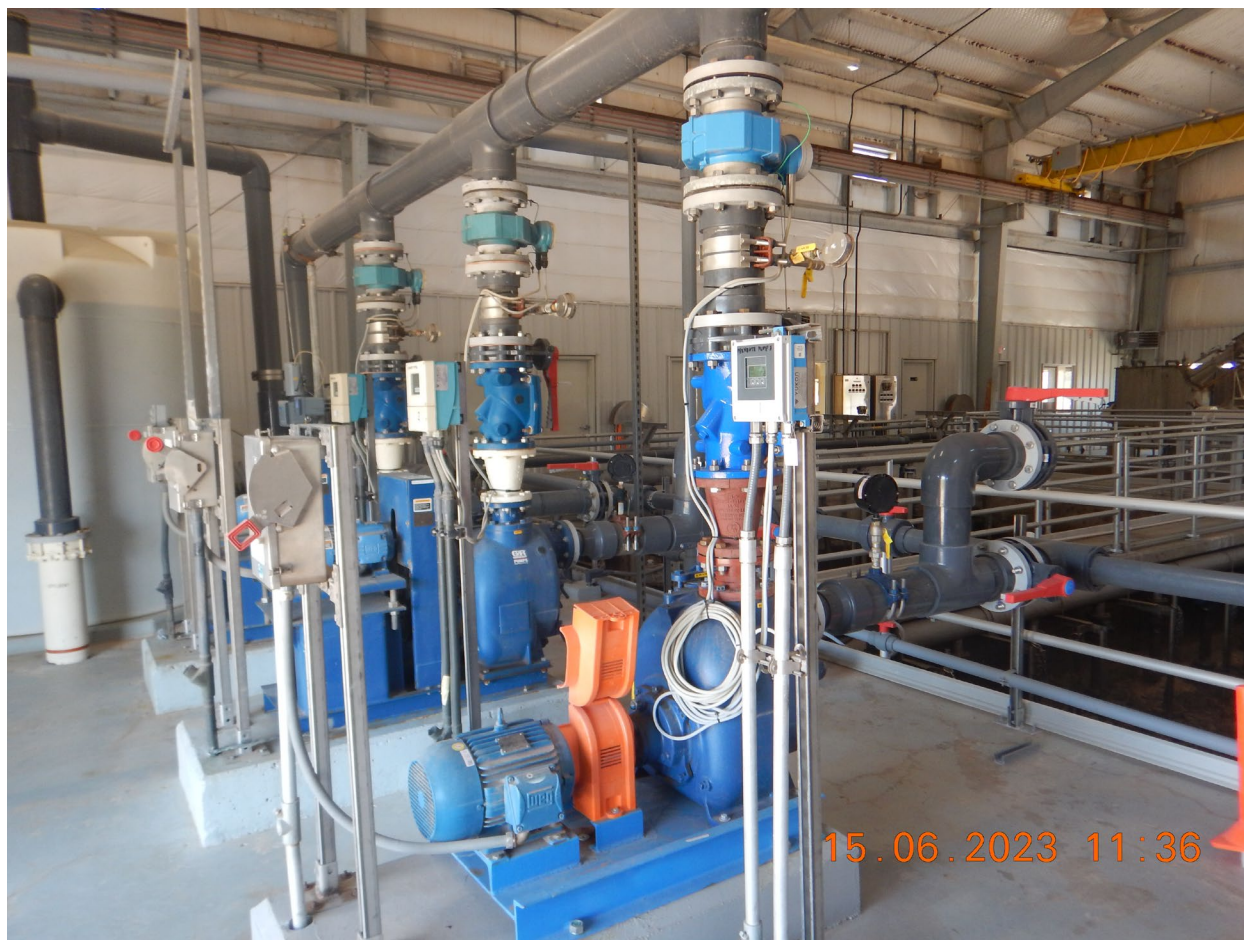
Picture of the three (3) MBR Permeate pumps located along the approximate southside of the treatment plant. (DSCN 2592). Photographed by D. Esparza.
