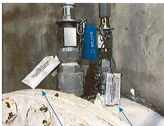
South – Caustic Injection Tag
