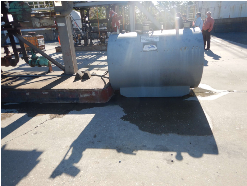
DSCN2464 View of small fuel tank labeled "E-5 Peninsula"
