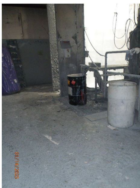
Picture 31 – Paint Area Filter Wall SAA
