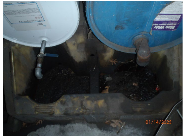
Picture 5 – Used Oil Drum Storage secondary containment
