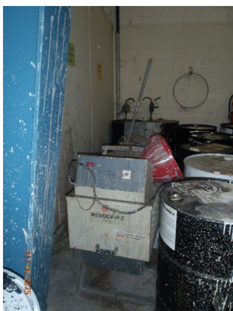
Picture 14 – Paint Area solvent recovery still pending repair
