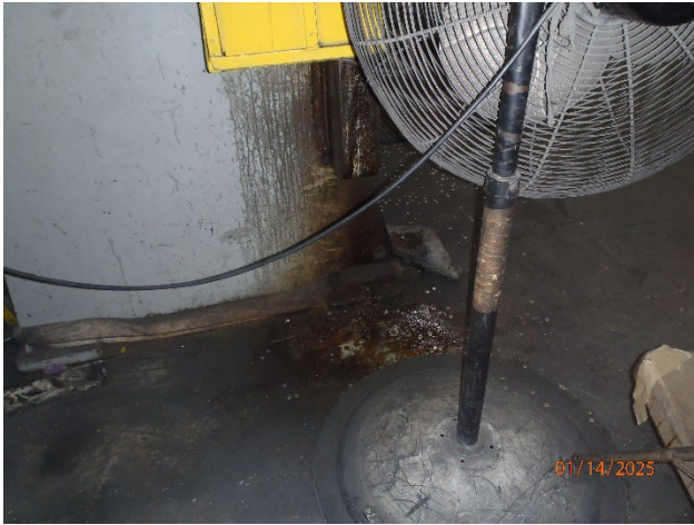
Picture 1 – Press brake machine oil release
