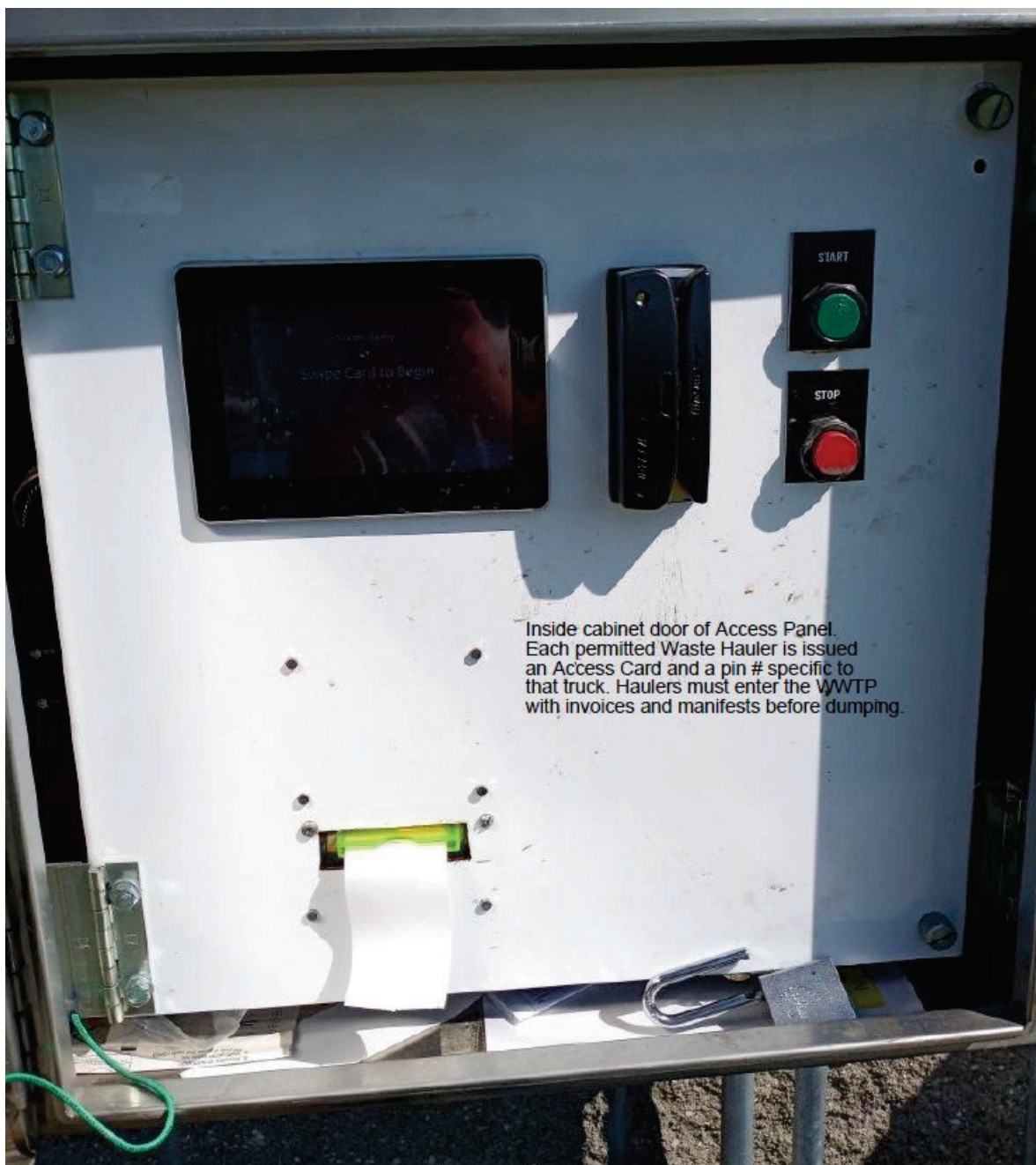
Figure 4 – Butte-Silver Bow Septage Receiving Station-Access Panel
