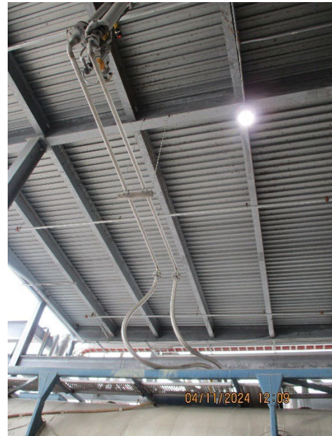
Photo 4: Top of hazardous waste tank and piping connections.
