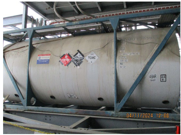
Photo 2: Hazardous waste tank in Solvent Feed Area.
