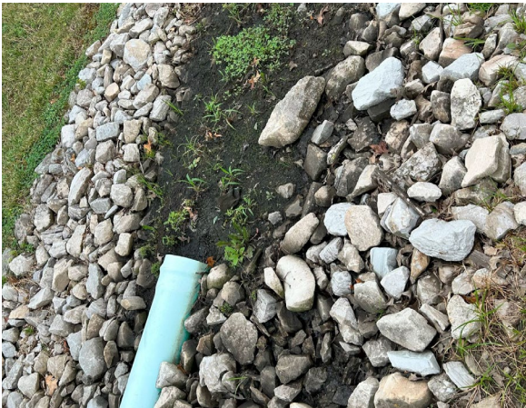
Photo-12 Used Oil draining into a drainage ditch
