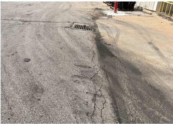
Photo-11 Pathway of Used Oil to a nearby storm drain
