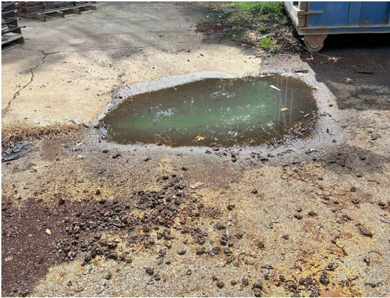
Photo-10 Used Oil puddling on a paved lot
