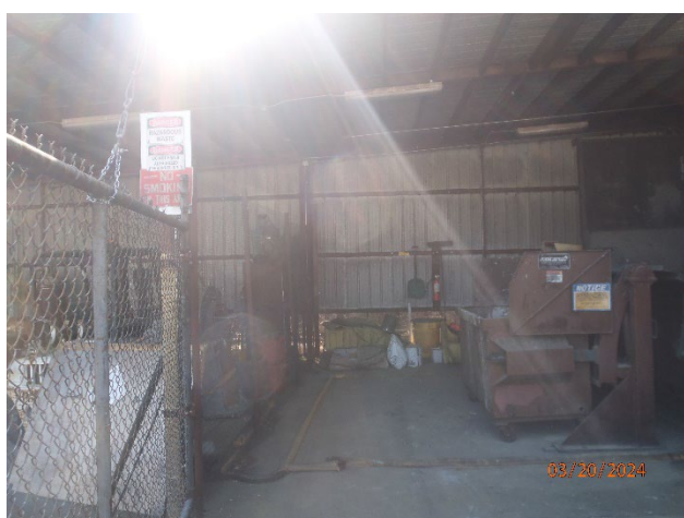
Picture 21 – Hazardous Waste Compactor
