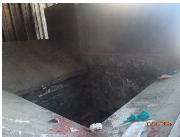
Picture 23 – Hazardous Waste Compactor opening
