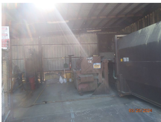
Picture 20 – Hazardous Waste Compactor
