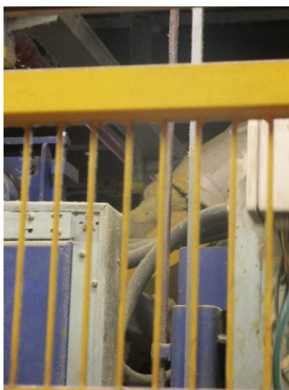
Figure 2. Photo taken by EPA during the inspection of August 15, 2023, showing accumulated PM on Unit 806
