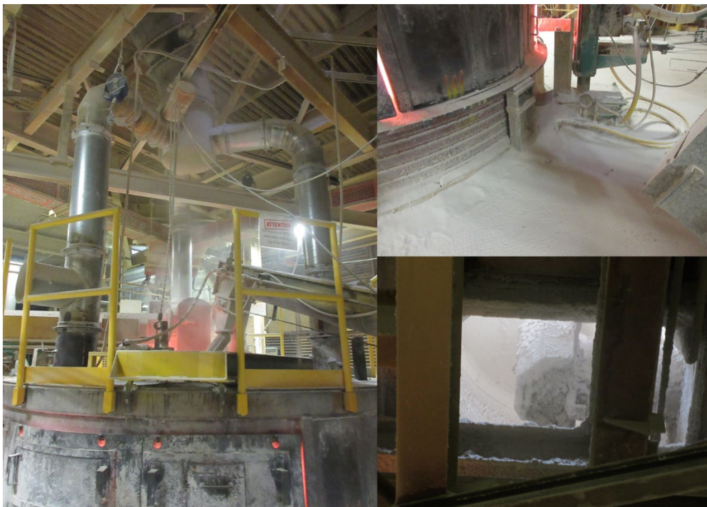
Figure 1. Photos taken by EPA during the inspection on August 15, 2023, showing a haze around melter 89 (left), PM accumulated on the melter 89 platform (top right), and PM accumulated in the roof vent above melter 89 (bottom right).
