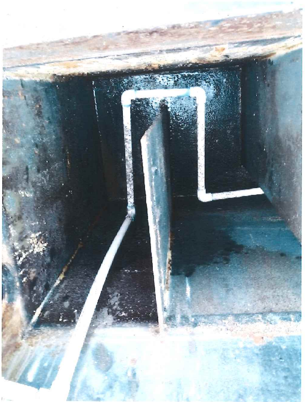
3-12-19 Kindco CCC Pump Back into Plant
