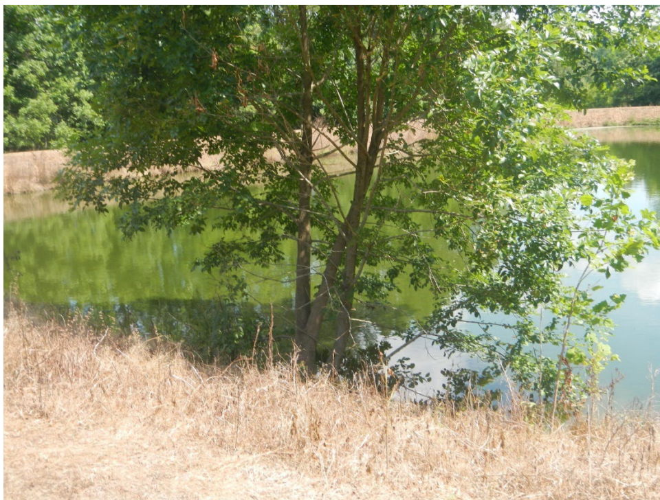
Figure 4. Tree growing on the inside wall of the wastewater lagoon berm.
