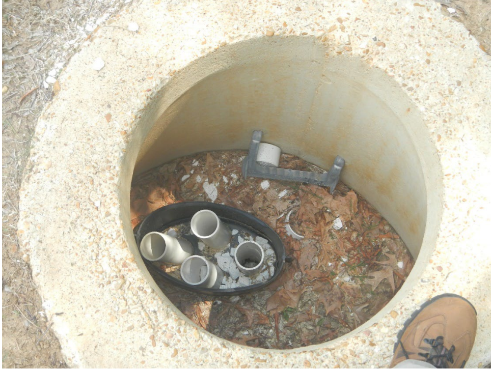
Figure 2. Chlorine contact chamber. Water has limited contact with chlorine tablets.
