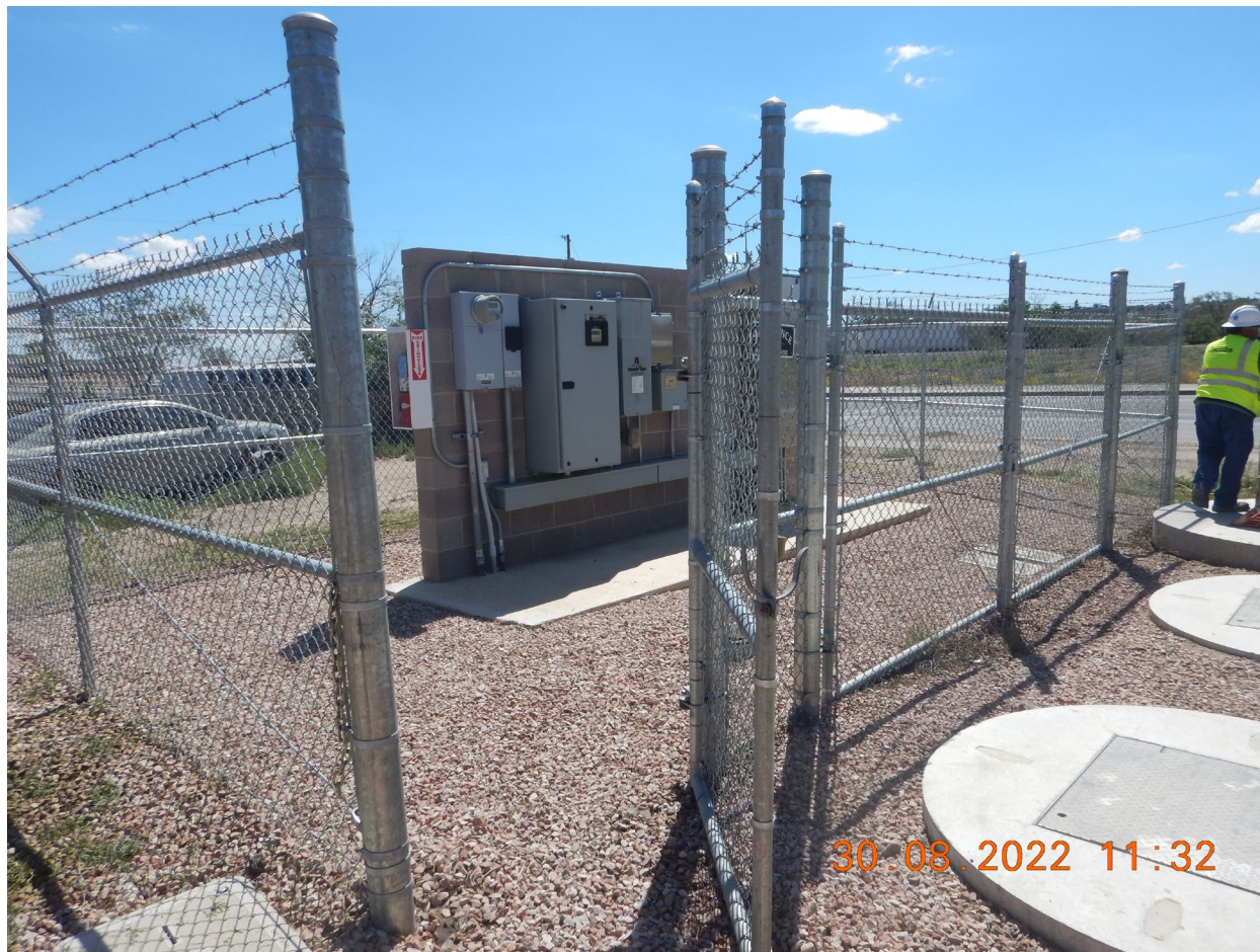
City of Gallup- Maxwell Lift Station. Fenced enclosure. Lacking signage, does have stub-out for back-up power and audible alarms (DSCN2307). Photographed by D. Esparza
