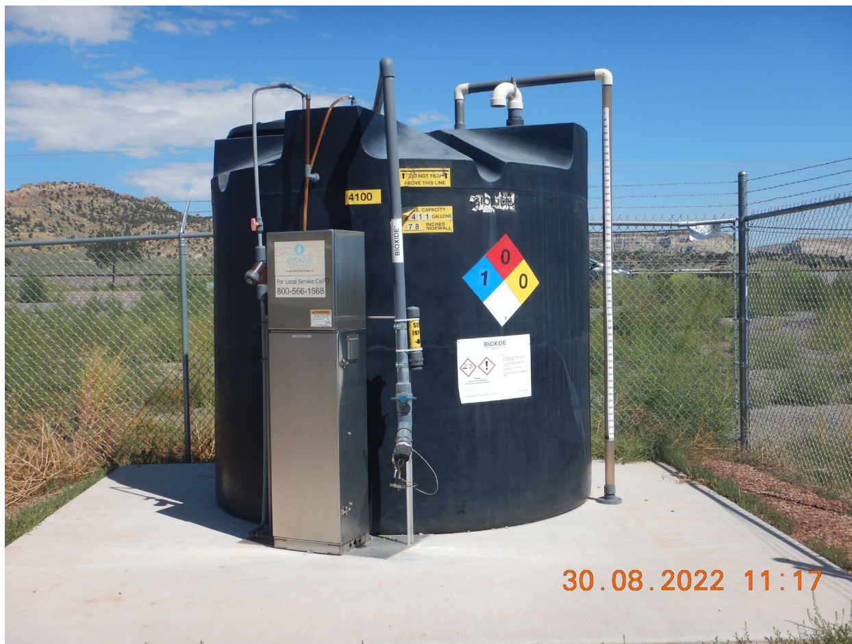
City of Gallup- Indian Hills Lift Station. Bioxide used in effort to lower Hydrogen Sulfide ( H_2S ) gas in lift station. (DSCN2303). Photographed by D. Esparza
