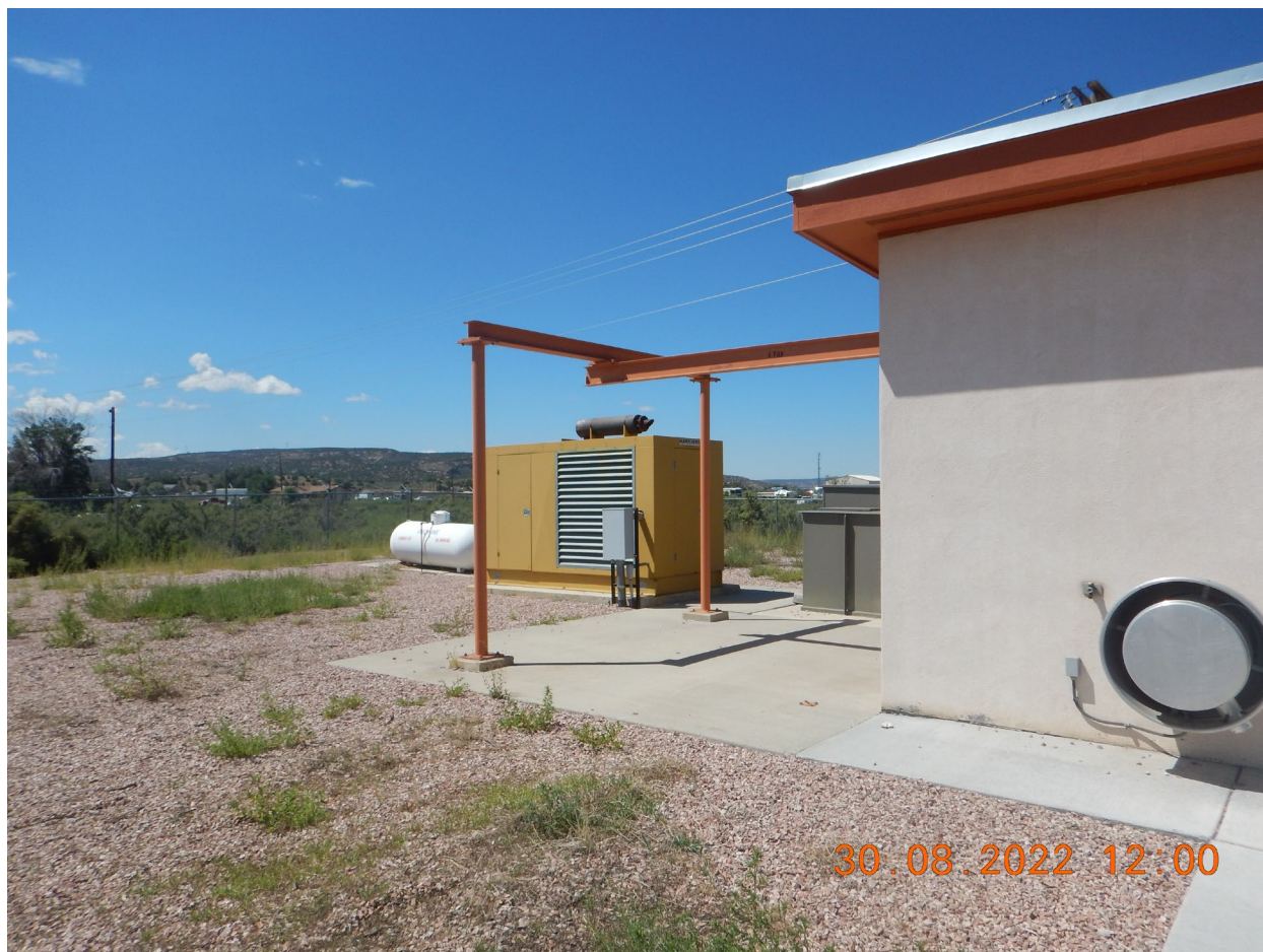
City of Gallup- Mentmore Lift Station. Enclosed CMU* (CMU- Concrete masonry unit (i.e., cinder block) building. On-site generator is exercised monthly. (DSCN2311). Photographed by D. Esparza
