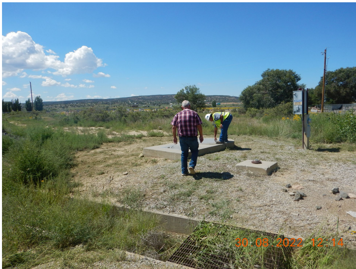
City of Gallup- Tomada Lift Station. Lacking fenced enclosure, signage, hatchway safety gate, back-up power and alarms (audible or flashing light) (DSCN2312). Photographed by D. Esparza
