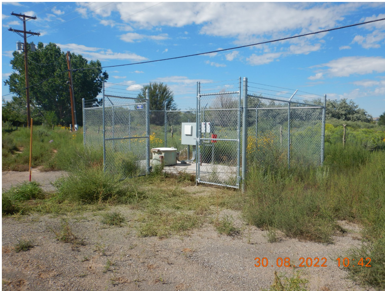
City of Gallup- Red Rock Lift Station. Fenced enclosure. Grinder pumps were installed circa June 2019. Lacking signage, back-up power and alarms (audible or flashing lights) (DSCN2300). Photographed by D. Esparza
