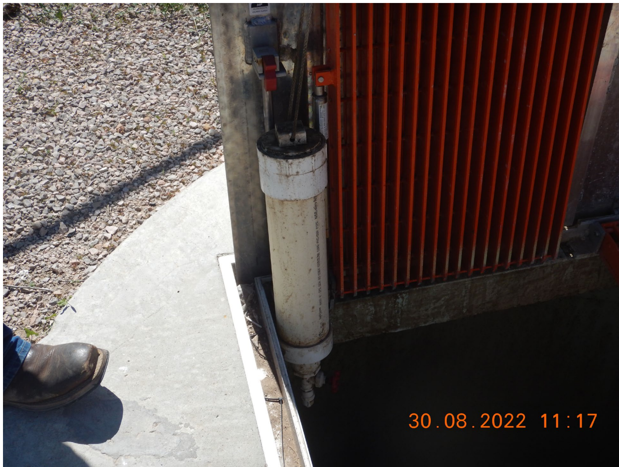
City of Gallup- Indian Hills Lift Station. Deodorizer installed below LS safety gate. (DSCN2302). Photographed by D. Esparza
