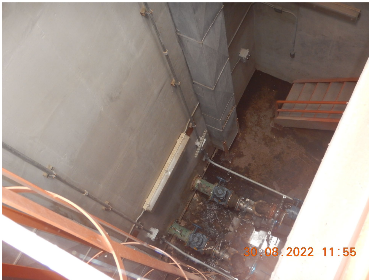
City of Gallup- Mentmore Lift Station. Pumps inside Mentmore LS. Pumps are serviced monthly (DSCN2309). Photographed by D. Esparza
