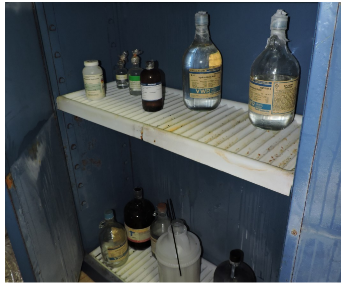
Picture 182 - UPR PHYSICS DEPARTMENT- At the Physics Labs, there were two (1) 4-L bottle hydrochloric acid, next to bottles of ammonium hydroxide, and potassium hydroxide (corrosive) not stored in a compatible manner and not used since year 2004.
