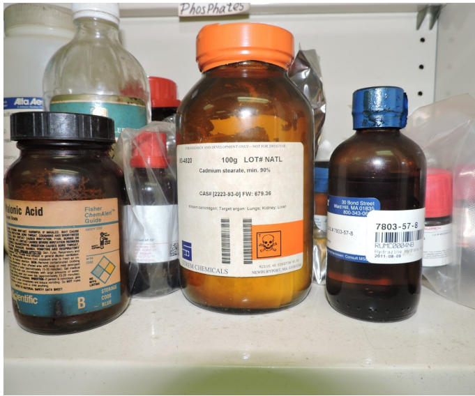
Picture 177 - UPR PHYSICS DEPARTMENT- At the Physics Lab F-458, there was cadmium stearate (toxic) next to malonic acid (corrosive) among many other chemical reagents stored together in an incompatible manner where they can be inadvertently mixed or where a spill or leak can cause danger or explosion.
