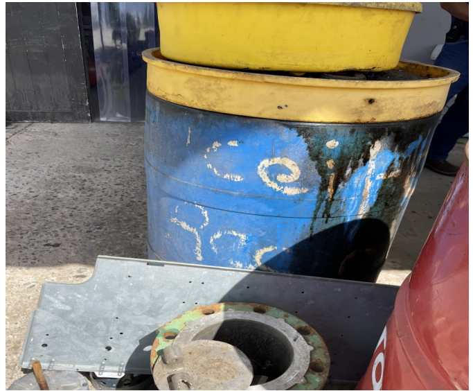
Picture 102 - UPR BUILDINGS & LAND DEPARTMENT- At the Refrigeration Shop, there was one (1) 55-gallon blue drum with a yellow drainage tray on top with used oil generated from draining compressors not marked with the words, "Used Oil"
