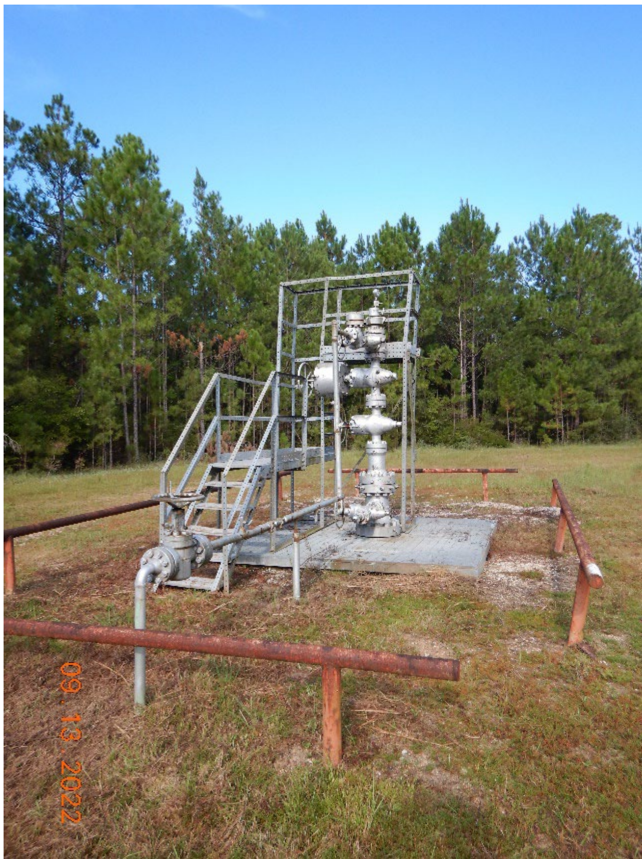
Photograph 5: Looking east, site overview, including well head, pressure gauges, valves, and access stairs.
