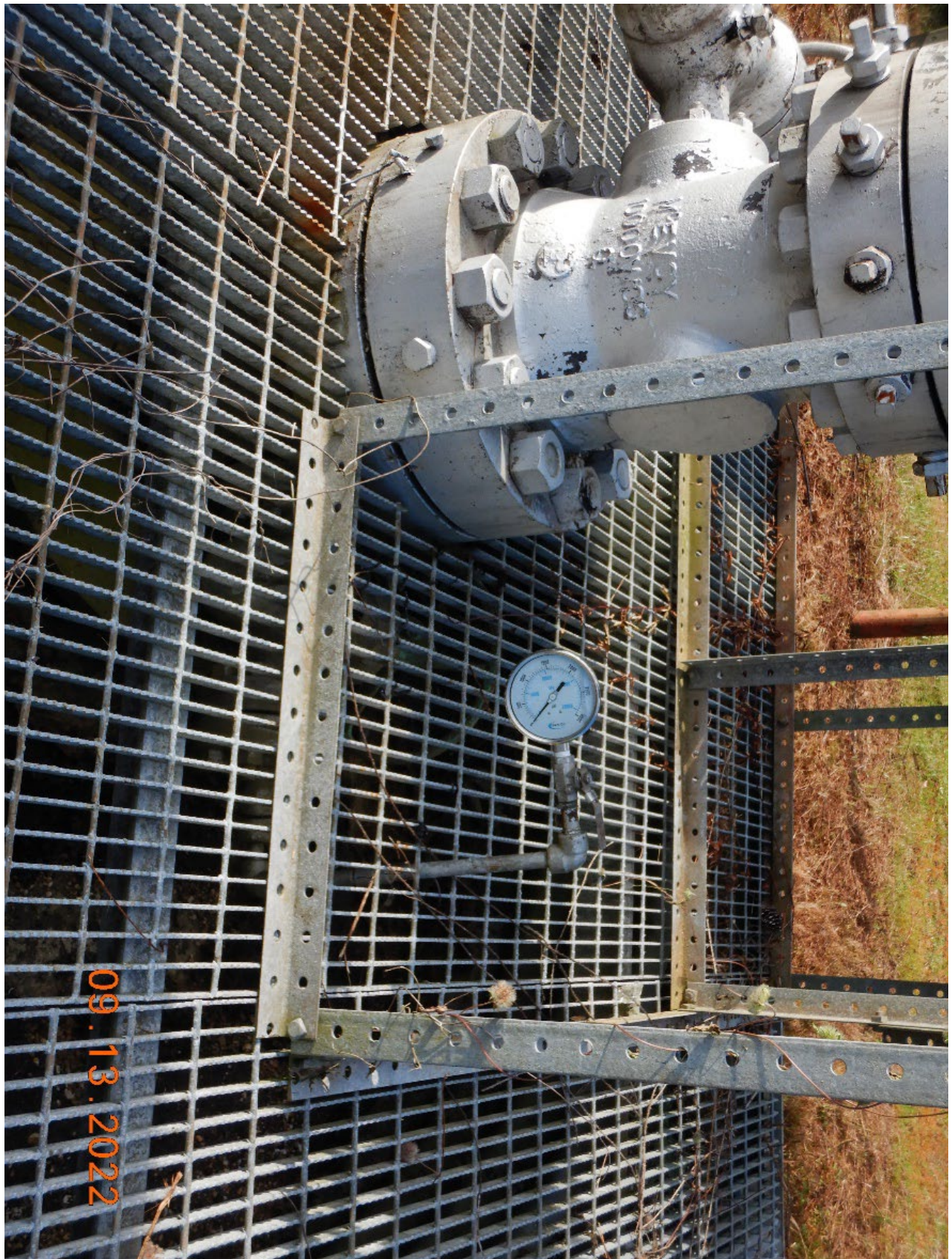
Photograph 2: Looking south, closeup view of surface casing pressure gauge reading 0 psi.
