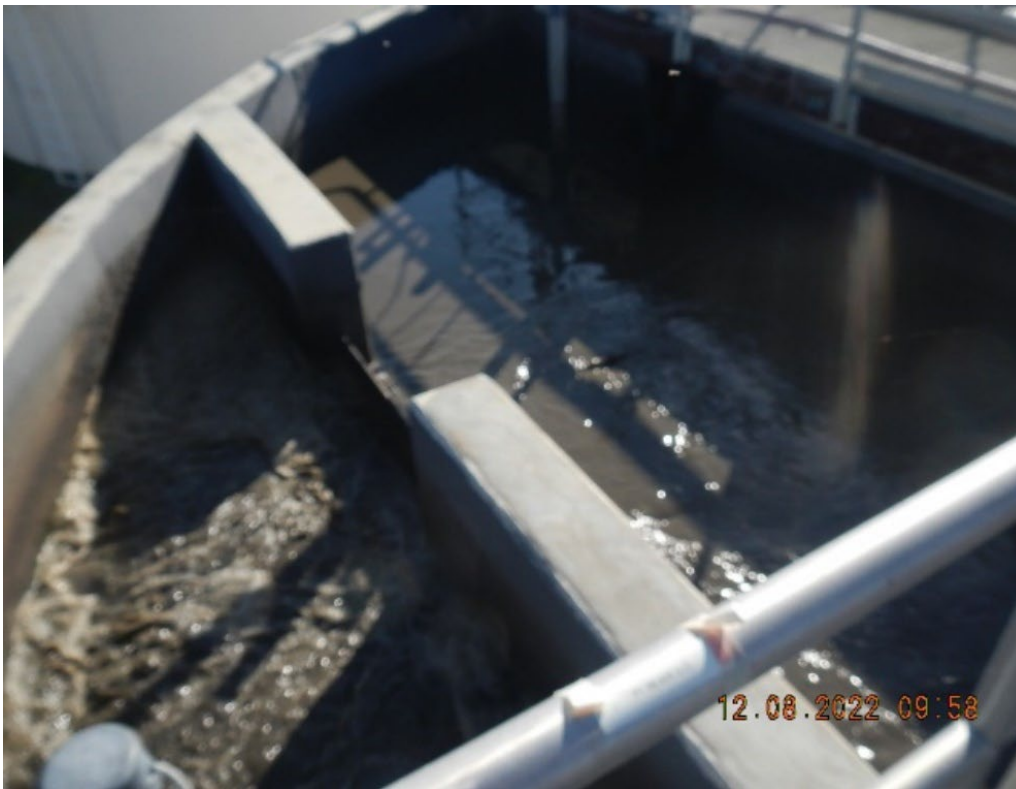
Photo 5. IFAS post anoxic zone and re-aeration zone.
