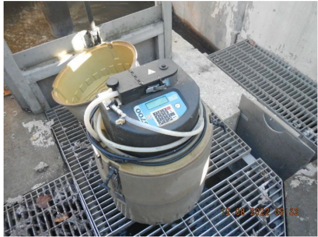
Photo 2: Portable ISCO composite sampler located at the Headworks.
