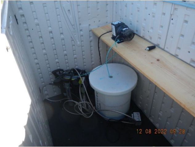
Photo 1. MUNOX® system storage tank and supply pump.
