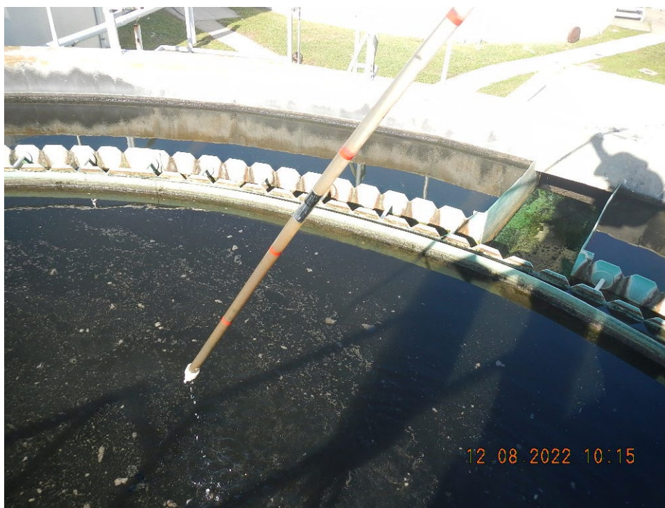
Photo 6. Sludge judge measuring the sludge blanket depth at approximately 2 feet off the bottom of the clarifier.
