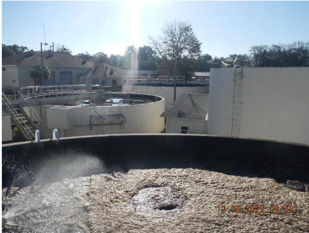
Photo 4. IFAS re-aeration zone.
