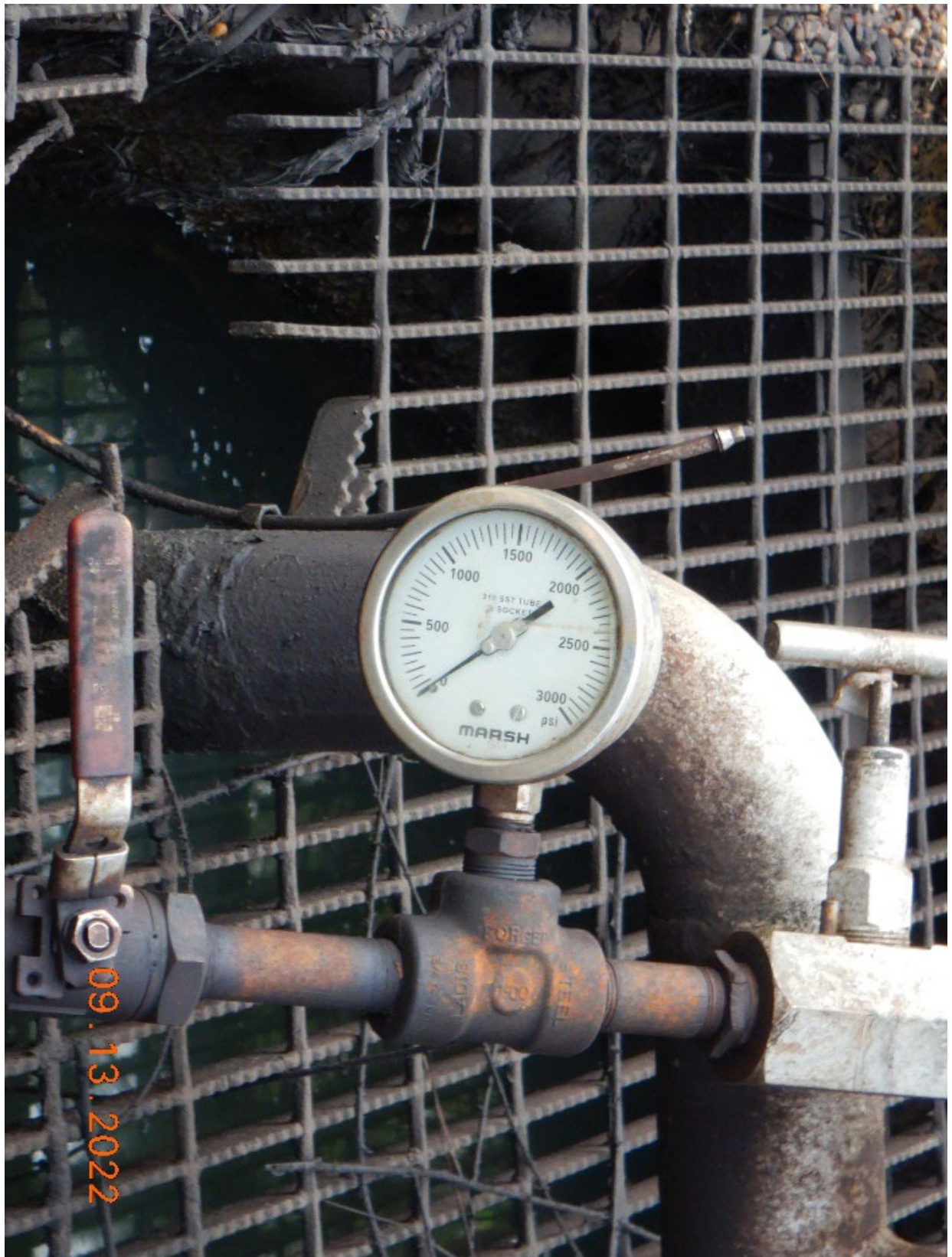
Photograph 3: Looking south, closeup view of casing pressure relief gauge reading 0 psi.
