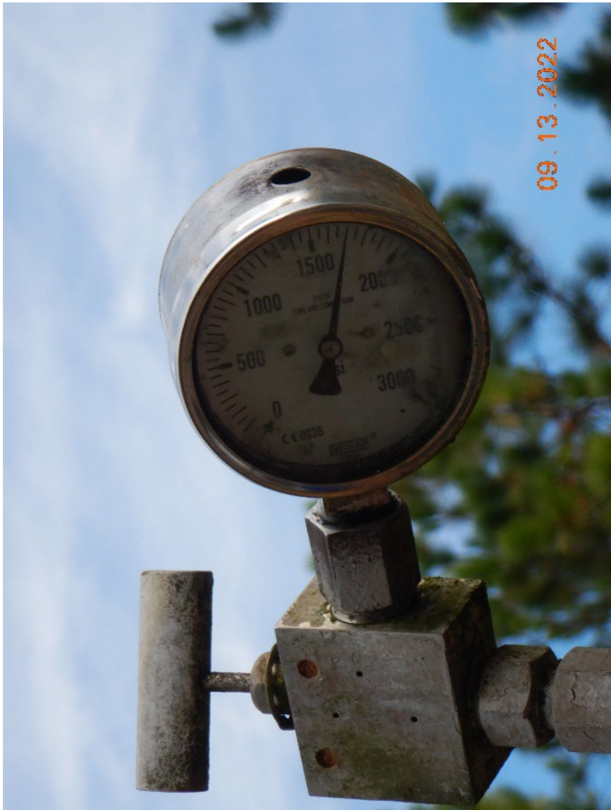
Photograph 4: Looking north, closeup view of internal pressure gauge reading 1,700 psi.
