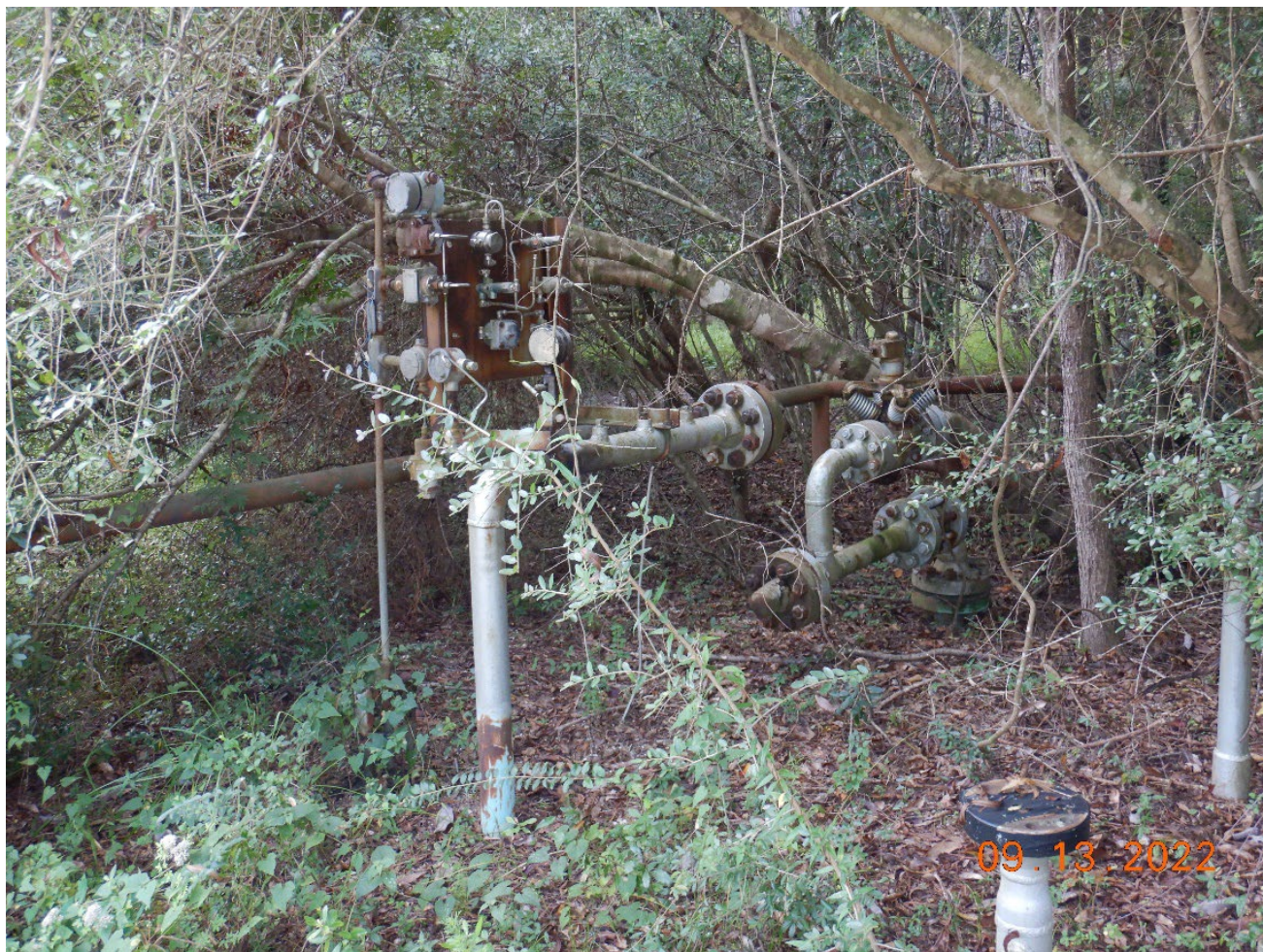
Photograph 5: View, looking south, of formerly-used casing pressure relief system. These lines are no longer connected to the well, and are sealed.
