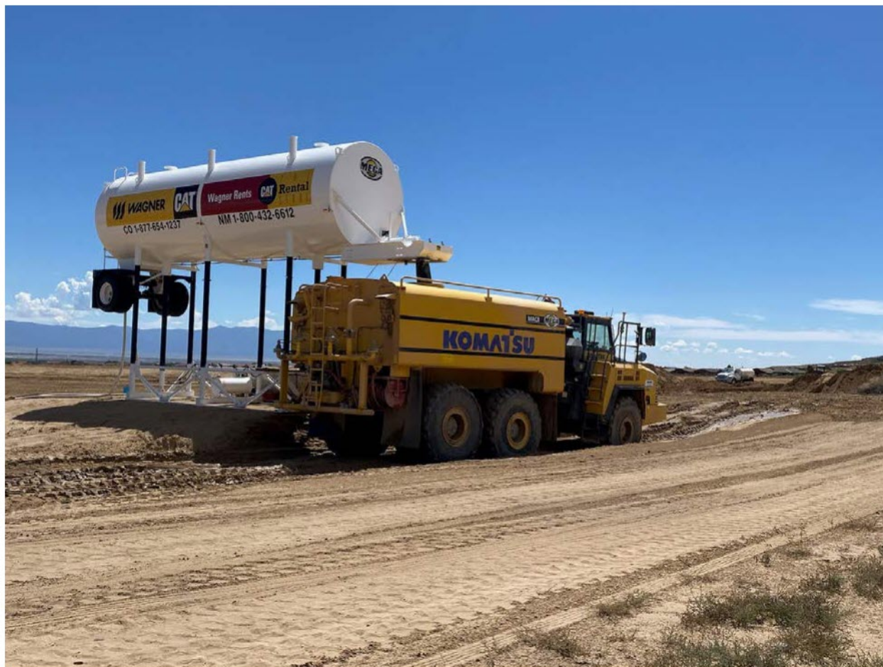
Project Antelope Phase II onsite water storage tank filling a water truck. Photograph provided by Greater Kudu/Facebook.
