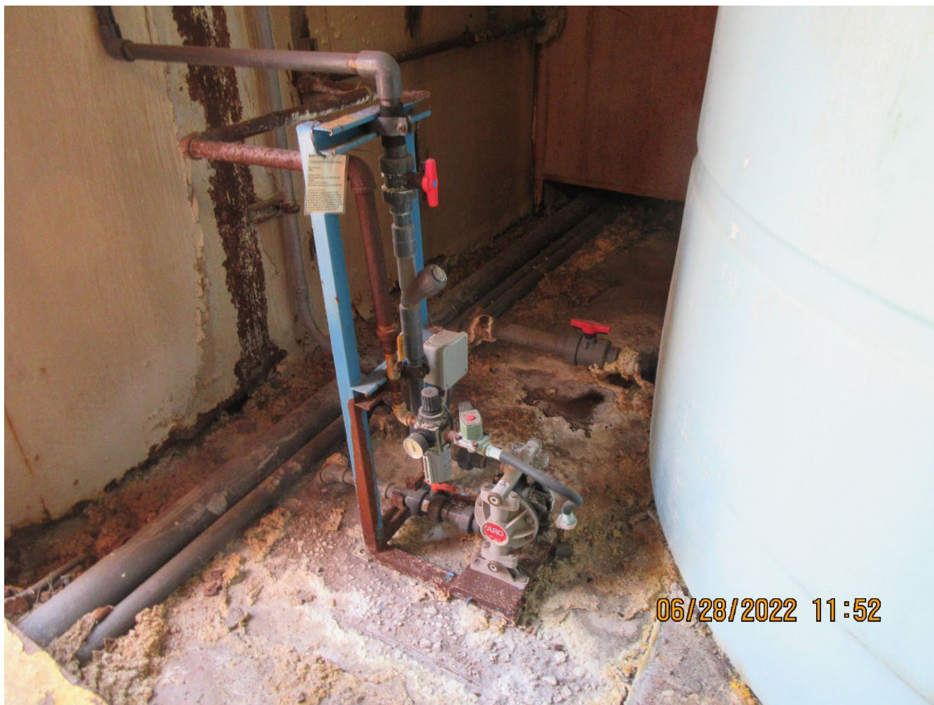
Photo 11 – Pump and metering device for overflow
