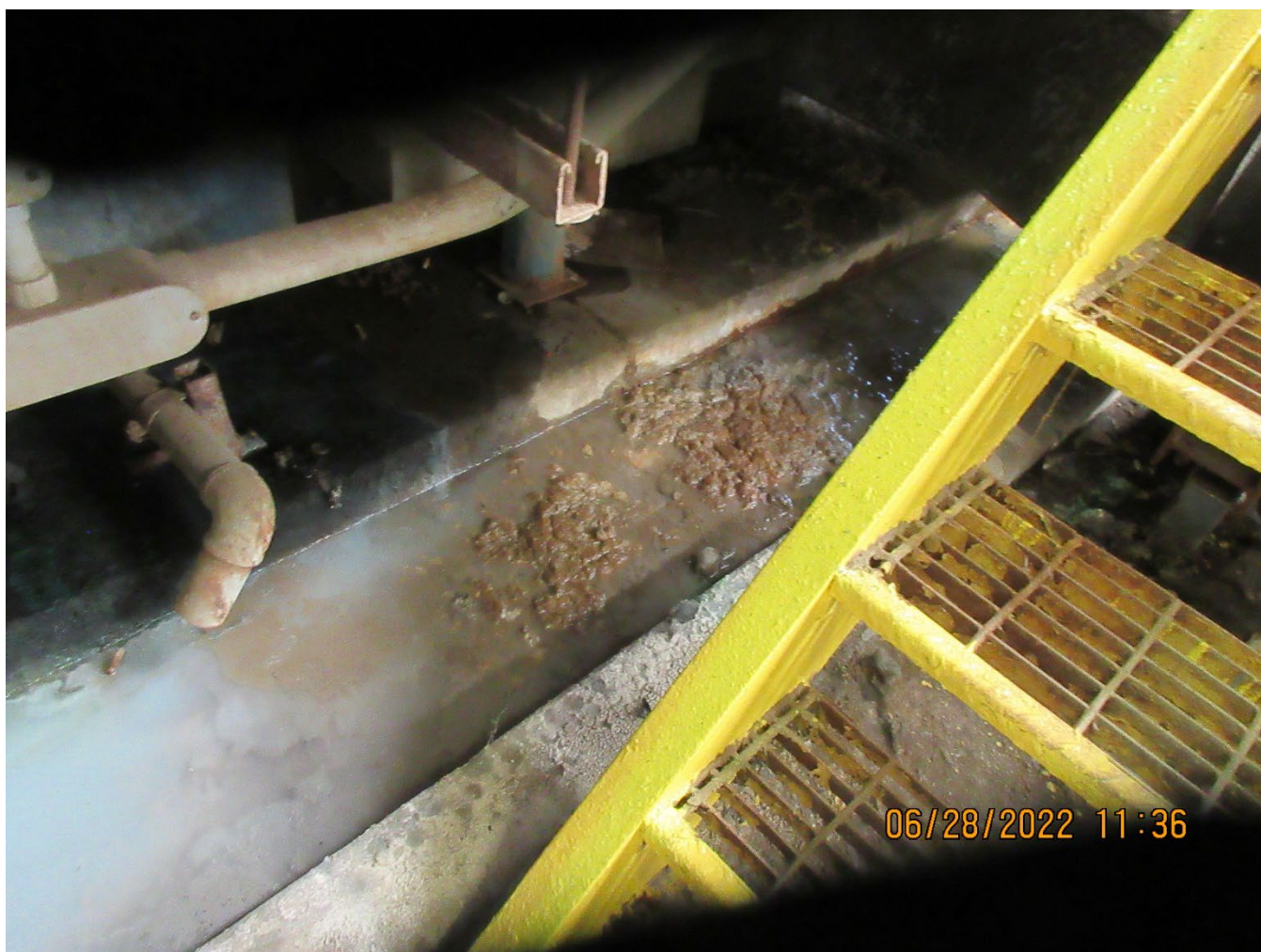
Photo 8 – Sludge in trough on north side of Rack Line 3
