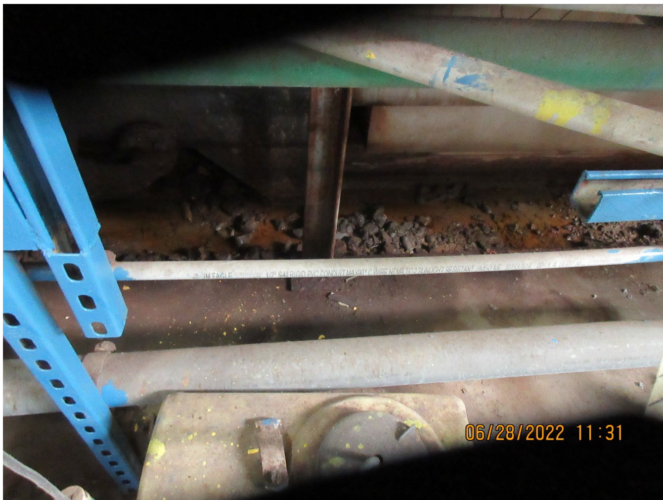
Photo 6 – Sludge in trough on north side of hoist line
