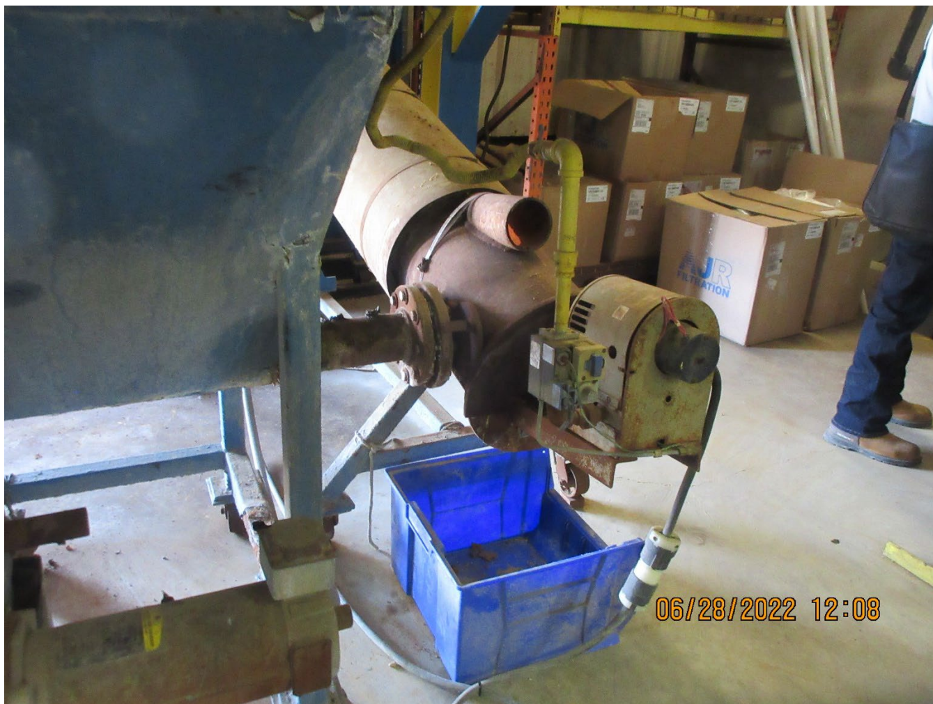
Photo 16 – F006 sludge gas-fired sludge dryer
