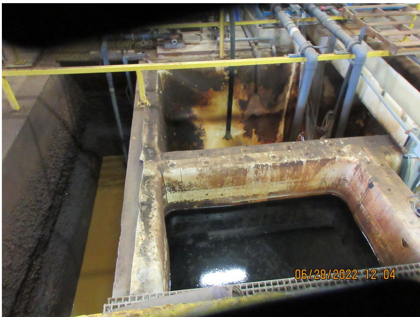
Photo 13 – Inground concrete wastewater treatment tanks
