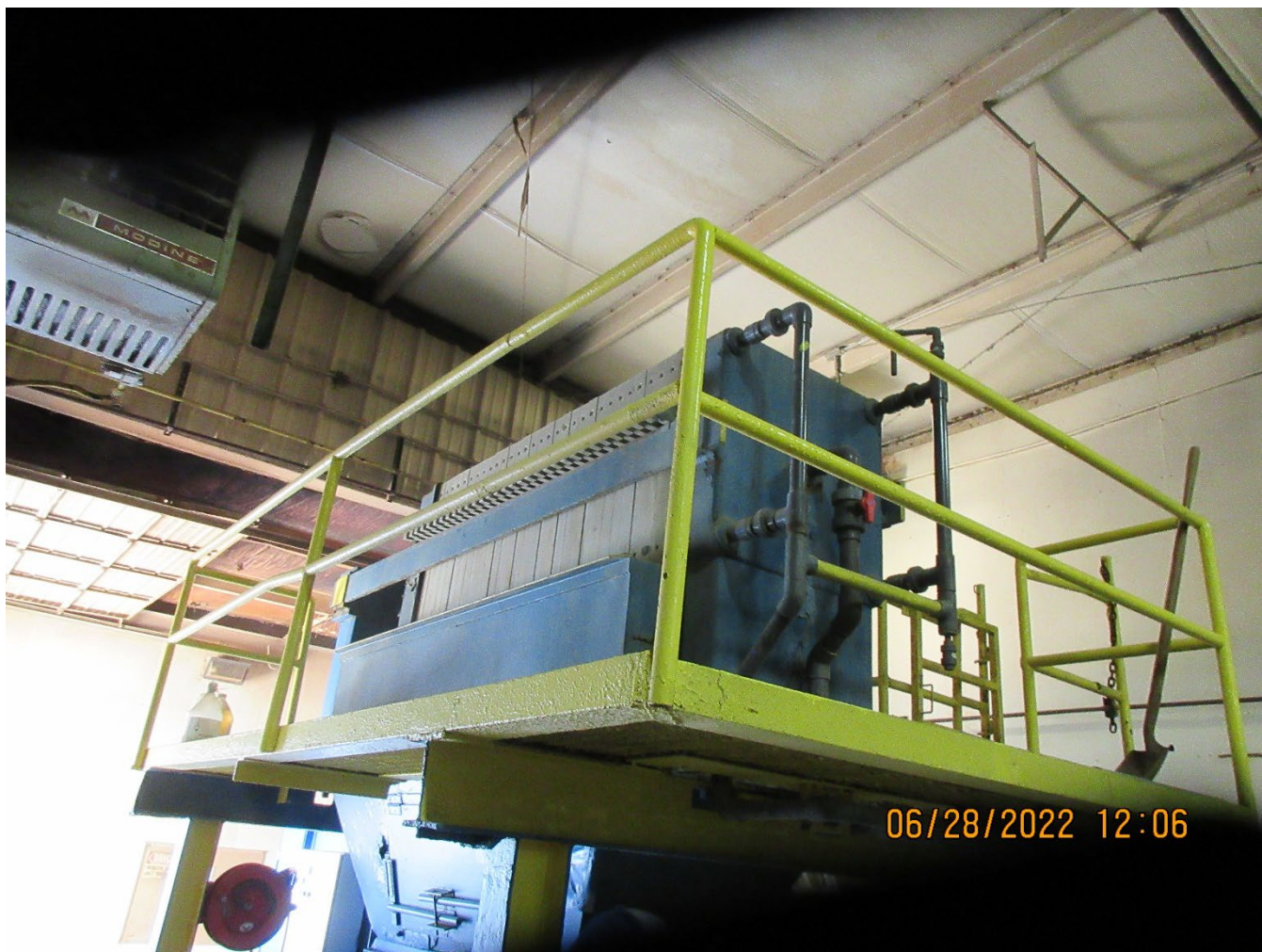
Photo 15 – F006 sludge filter press in wastewater treatment facility
