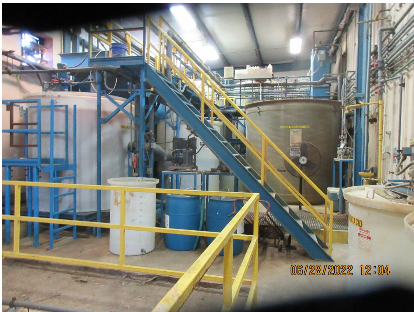
Photo 14 – Above ground poly and fiberglass wastewater treatment tanks
