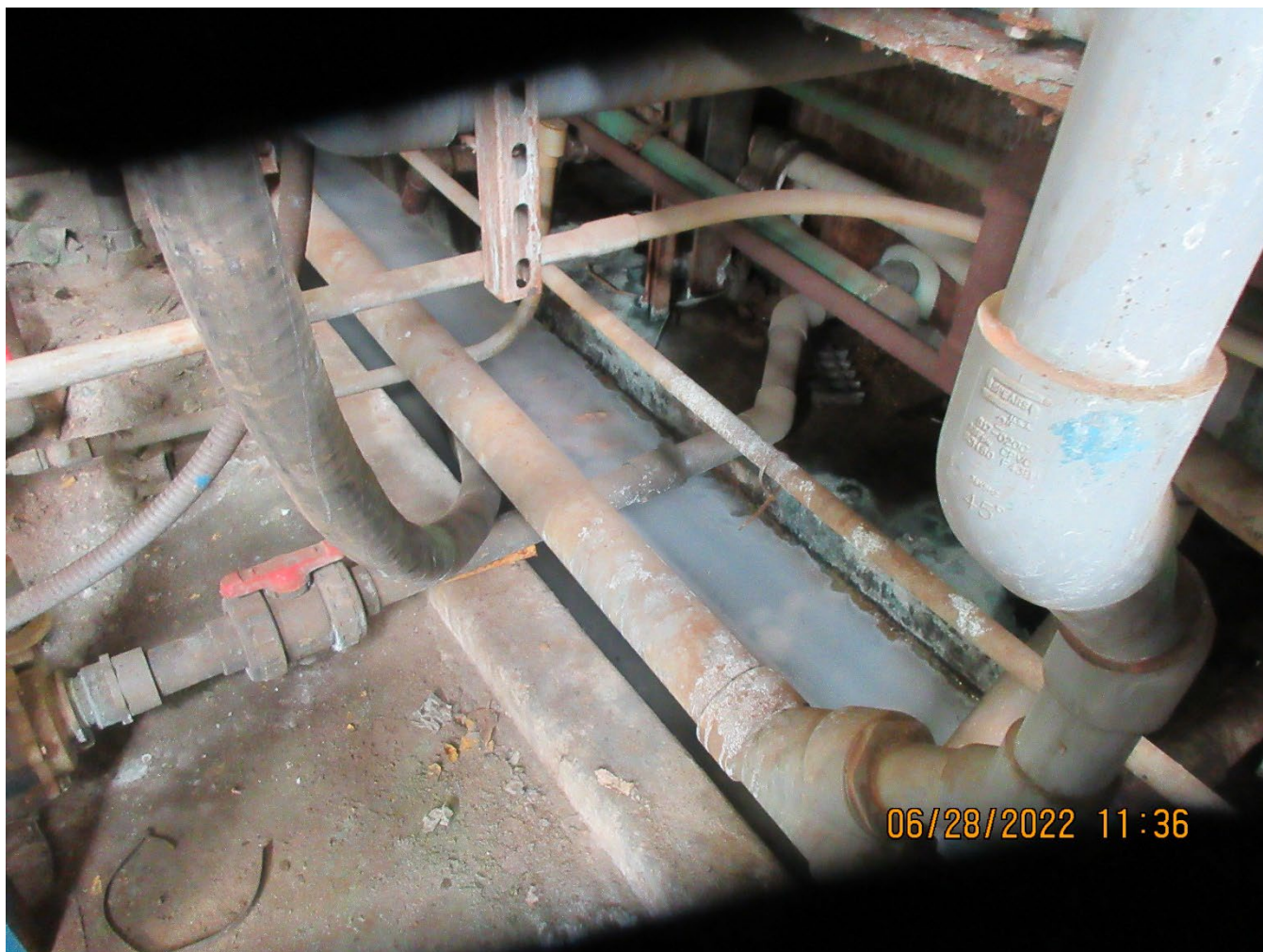
Photo 9 – Sludge in trough on north side of Rack Line 3
