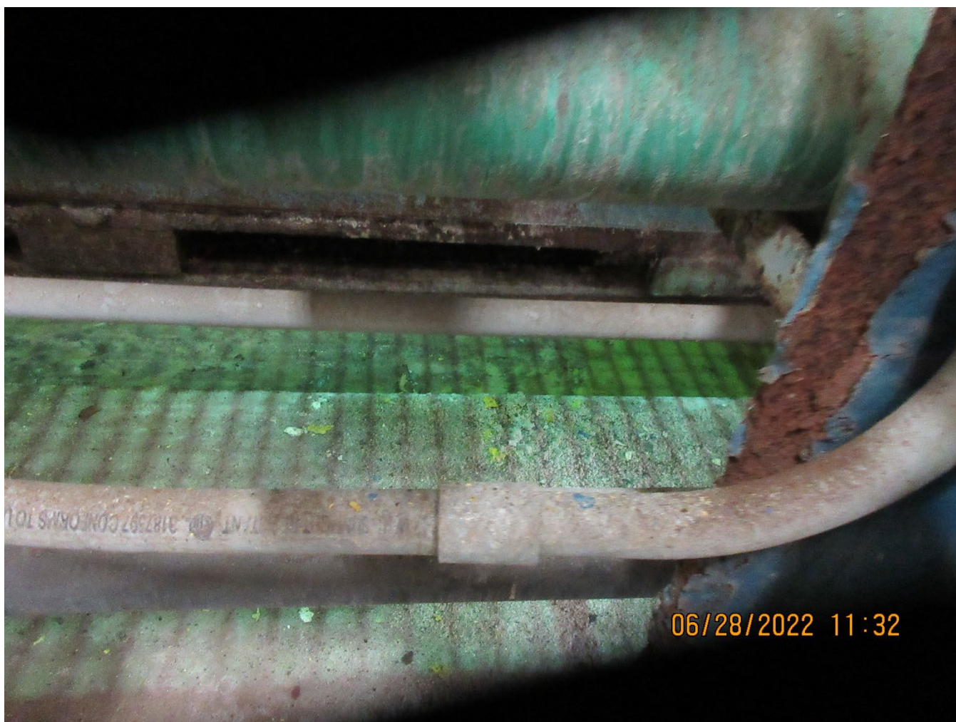
Photo 7 – Liquid and Sludge in trough on north side of hoist line
