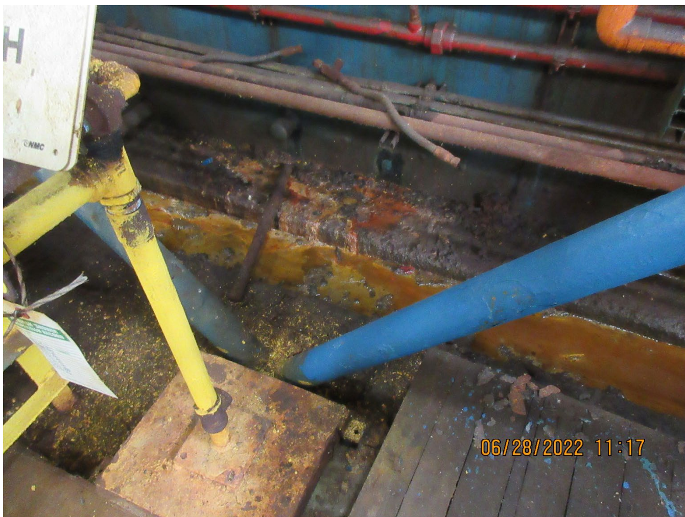
Photo 2 – Sludge in trough on north side of barrel line
