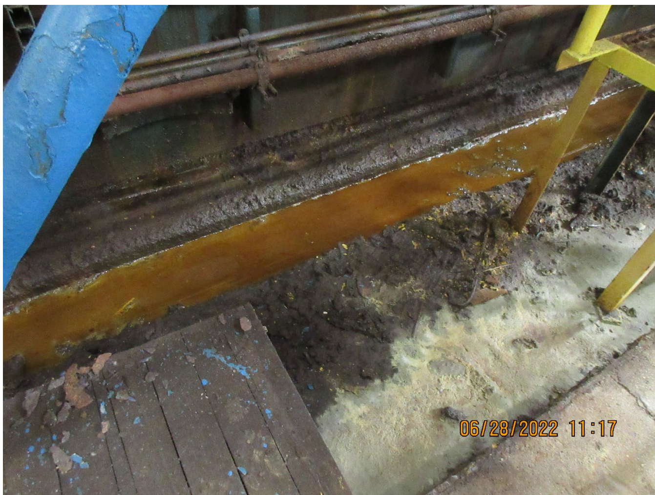
Photo 3 – Sludge in trough on north side of barrell line
