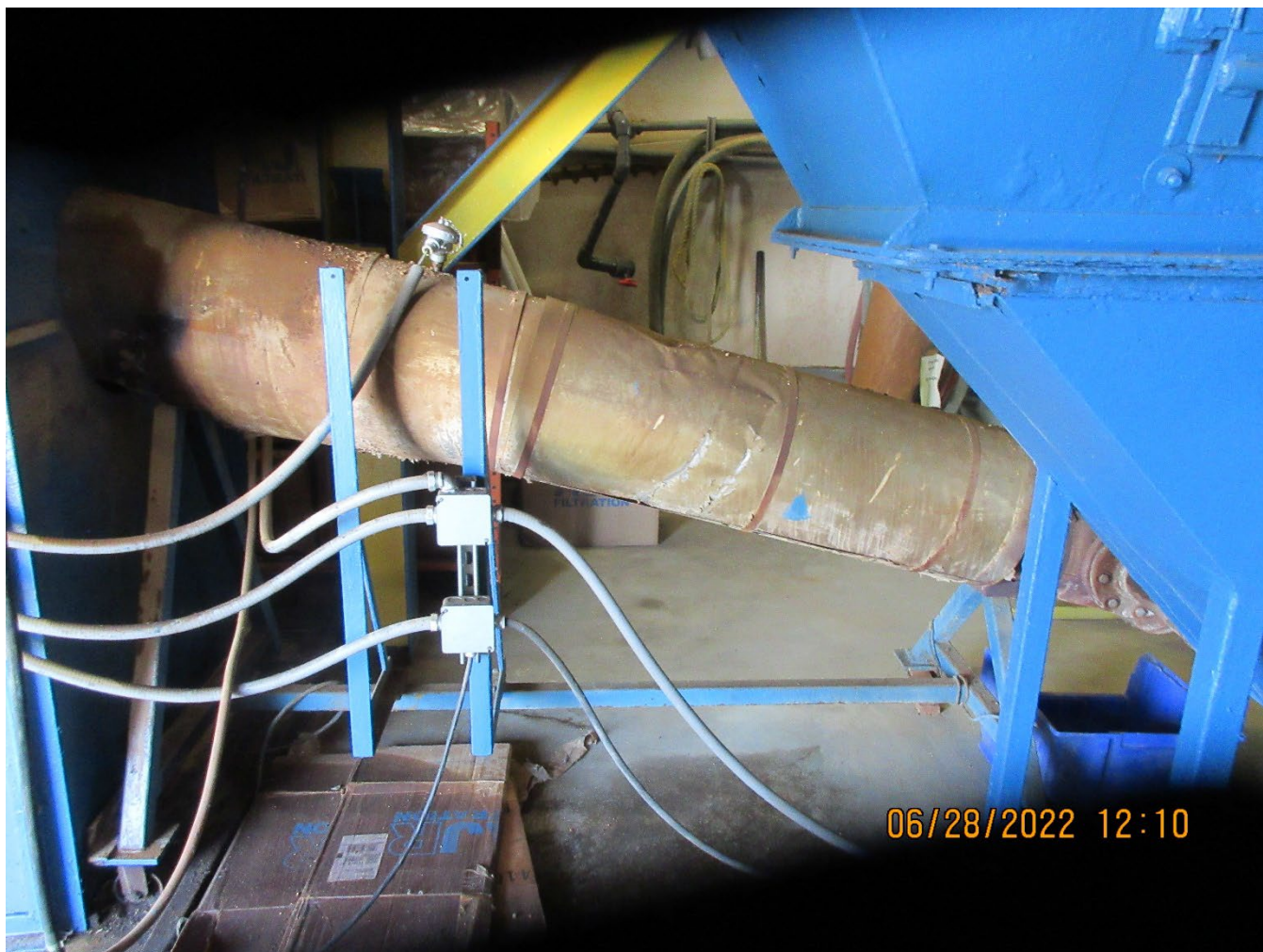
Photo 17 – F006 sludge gas-fired sludge dryer
