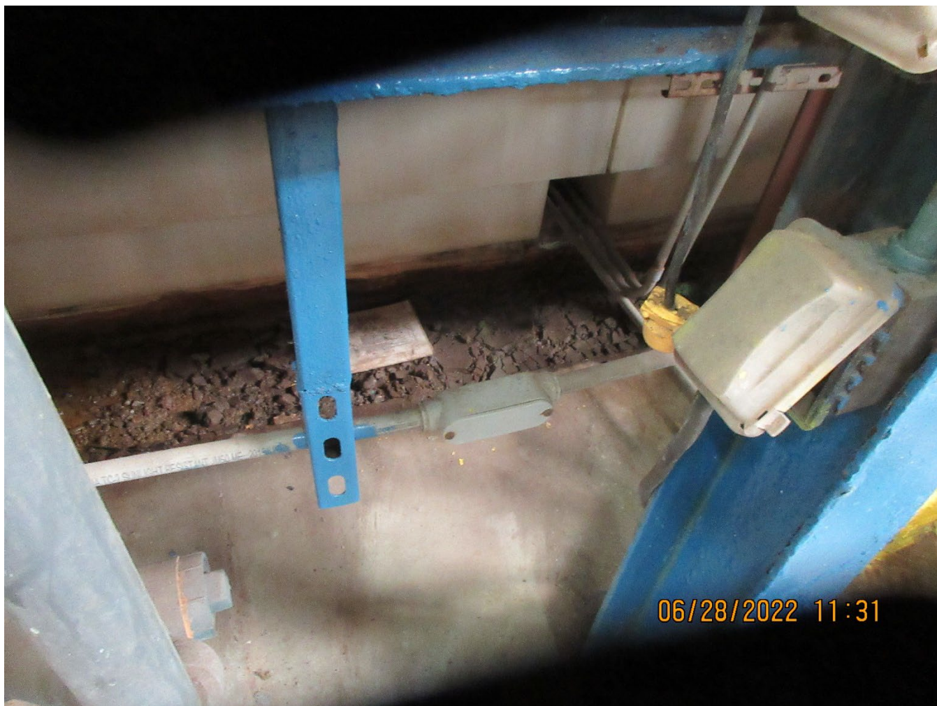
Photo 5 – Sludge in trough on north side of hoist or rack line
