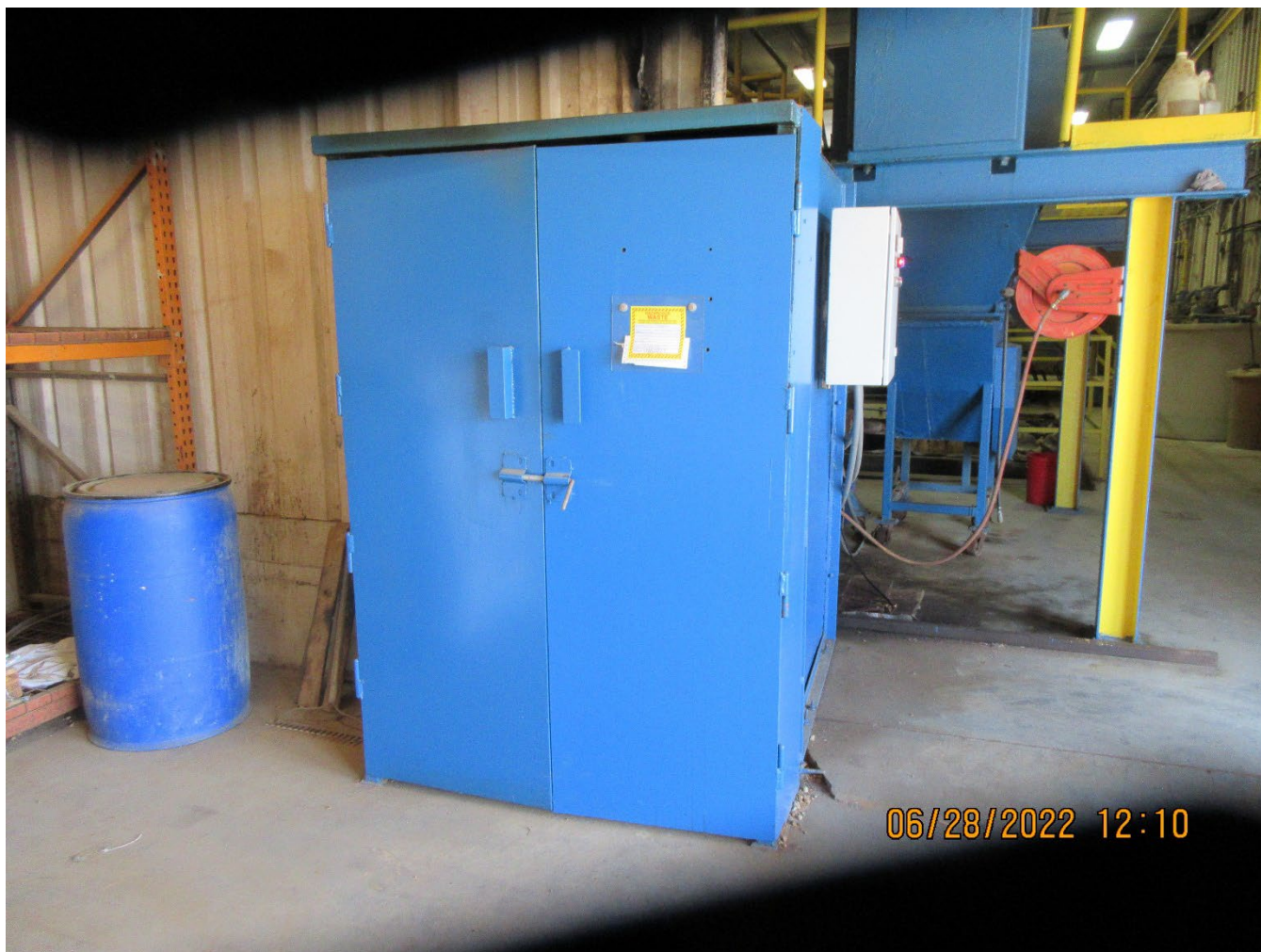
Photo 18 – F006 sludge collection cabinet from gas-fired sludge dryer
