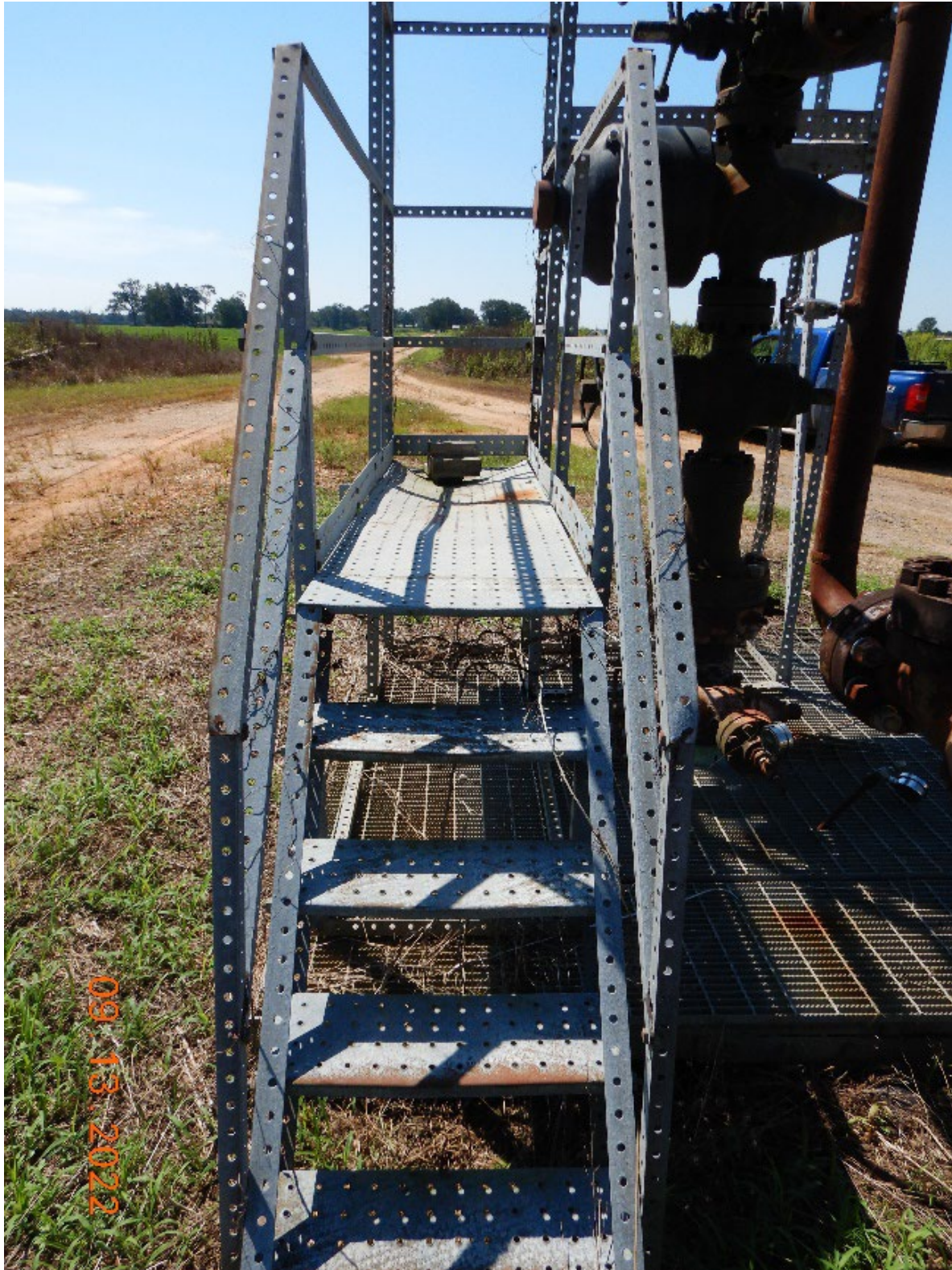
Photograph 6: Looking south, access stairway with sagging platform.
