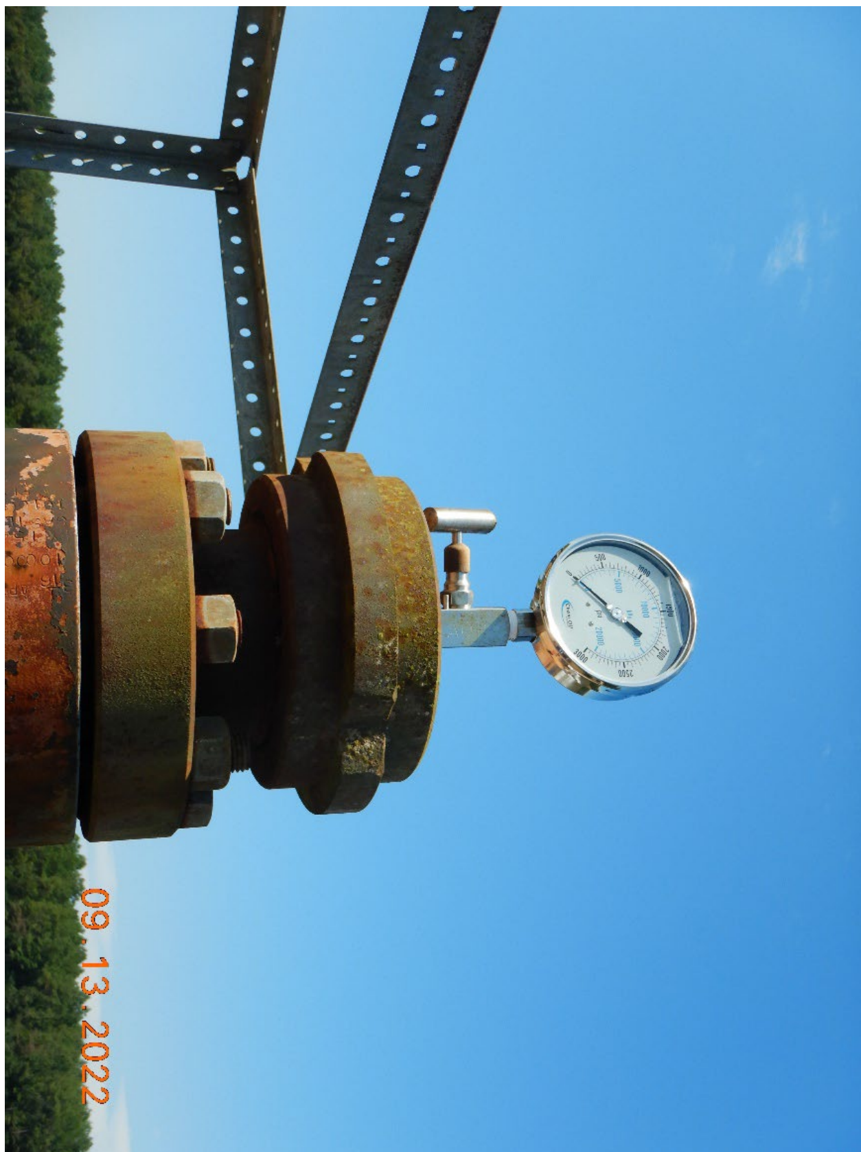
Photograph 5: Looking west, closeup view of internal pressure gauge reading 0 psi.
