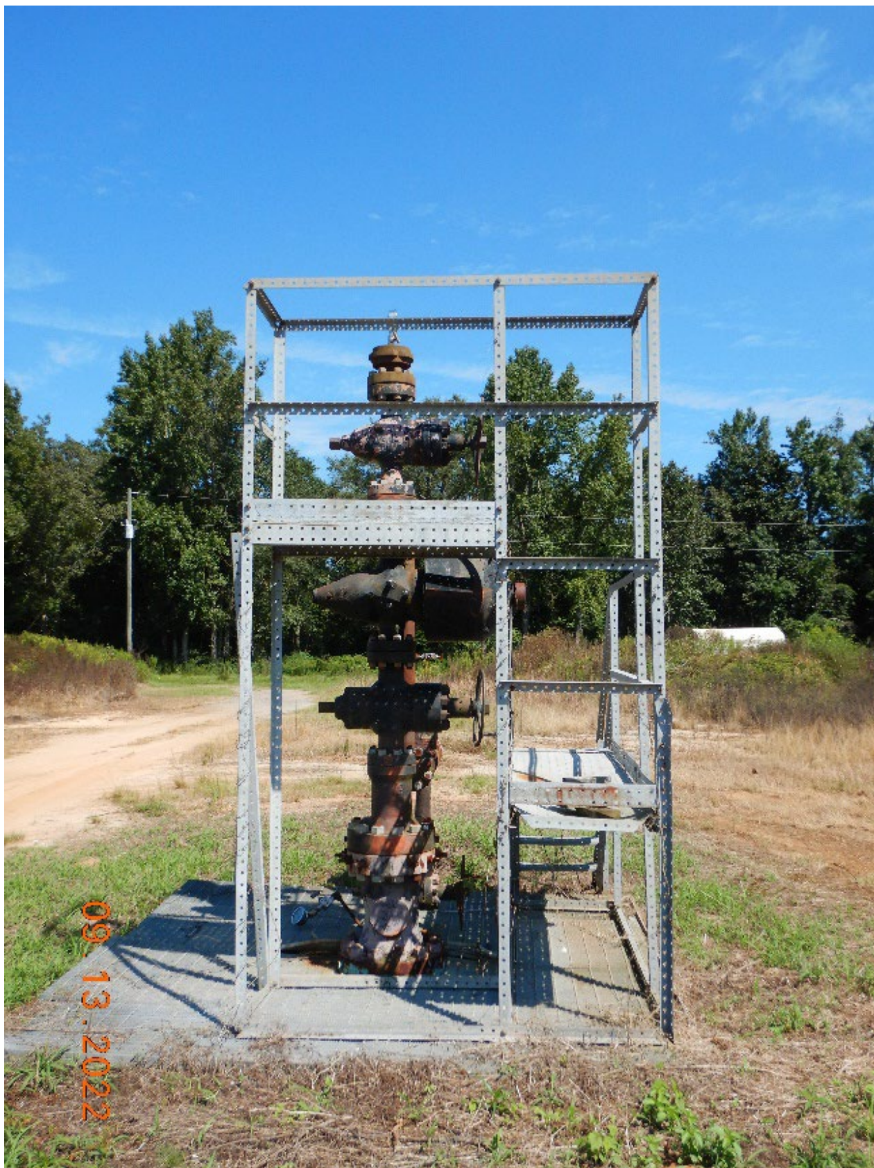
Photograph 2: Looking north, site overview showing well head, pressure gauges, valves, and access stairway.
