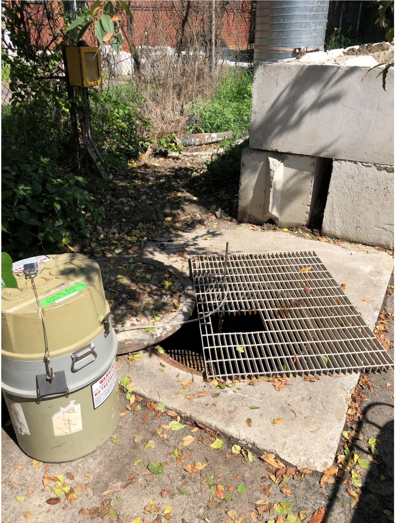
Photo #1: View of the pretreatment discharge location for Outfall DSN 001L.
