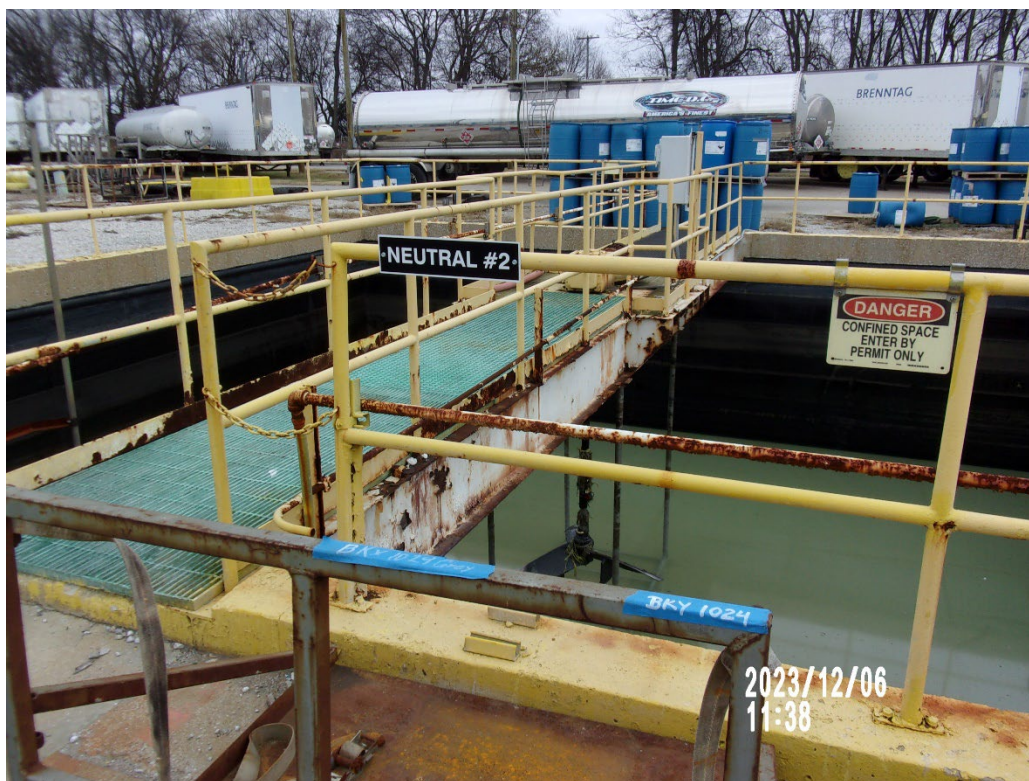
Photograph 19: Wastewater treatment area Neutralization Tank #2.
