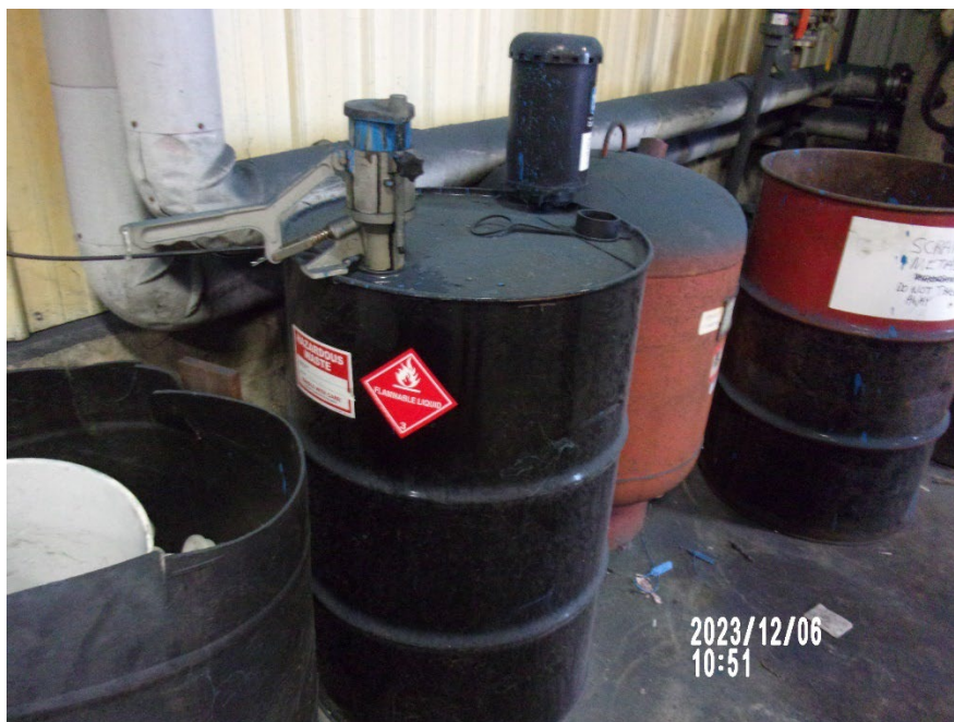
Photograph 12: Corrected container with new hazard indicator marking.
