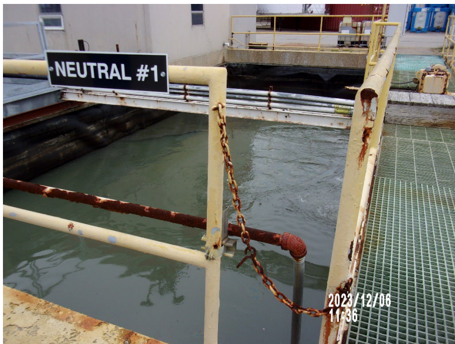
Photograph 18: Wastewater treatment area neutralization tank #1.
