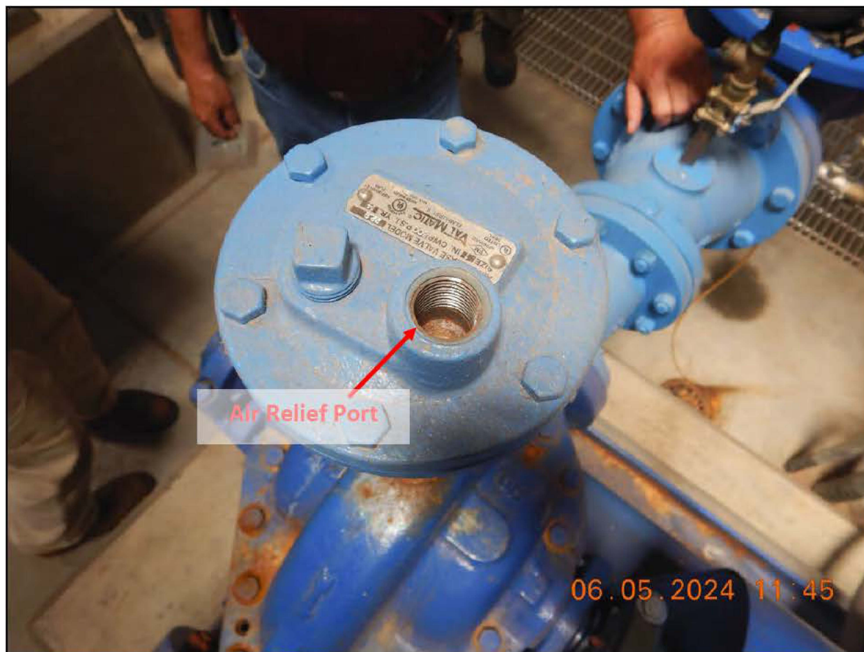
Photograph 29. 6/5/2024 11:45 AM DSCN0838.JPG South Perkins Road Pump Station View of an air relief port that was missing a downturned exhaust line.
