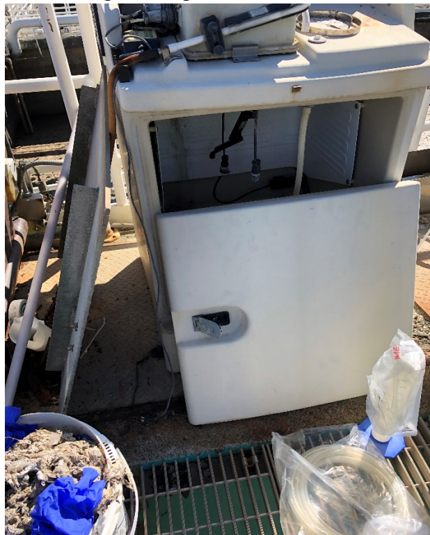
Photo #2. The facility's influent automatic composite sampler is out-of-service. As a result, composite samples are collected as grab samples.
