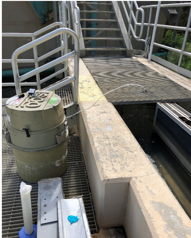
Photo #12. EPA automatic effluent composite sampler was set-up ahead of the UV System.
