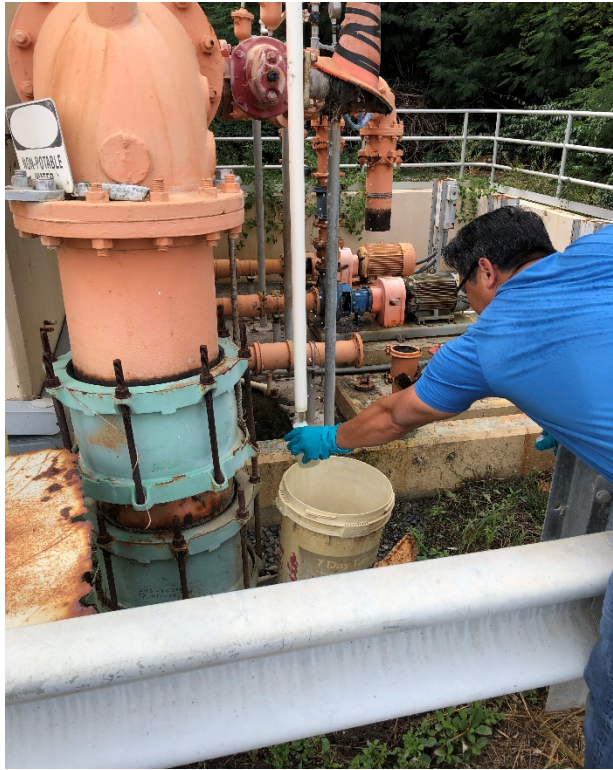
Photo #11. Compliance grab samples are collected from the effluent grab sampling point.
