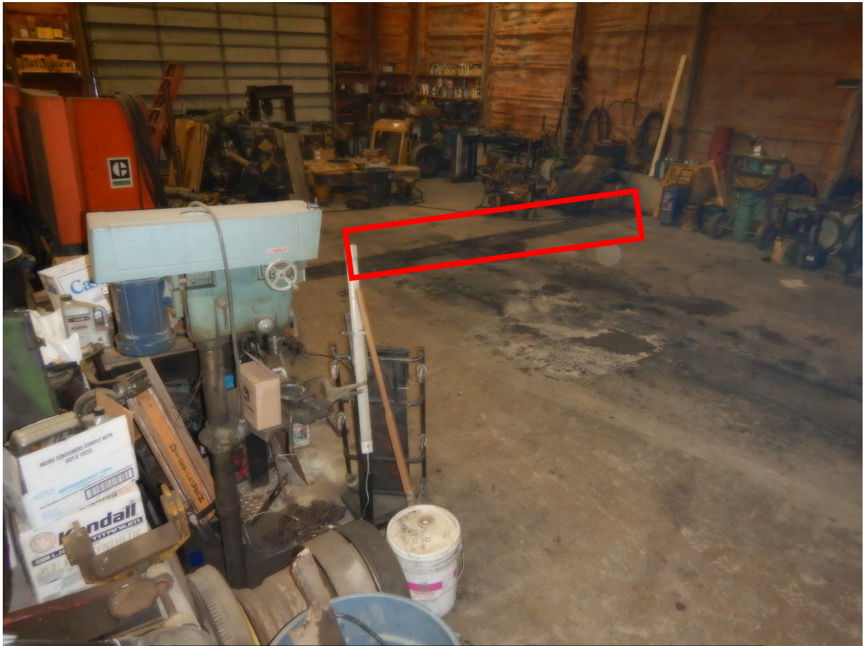
DSCN 4069 Trench drain (red box) in maintenance garage – drain was plugged at time of inspection.
