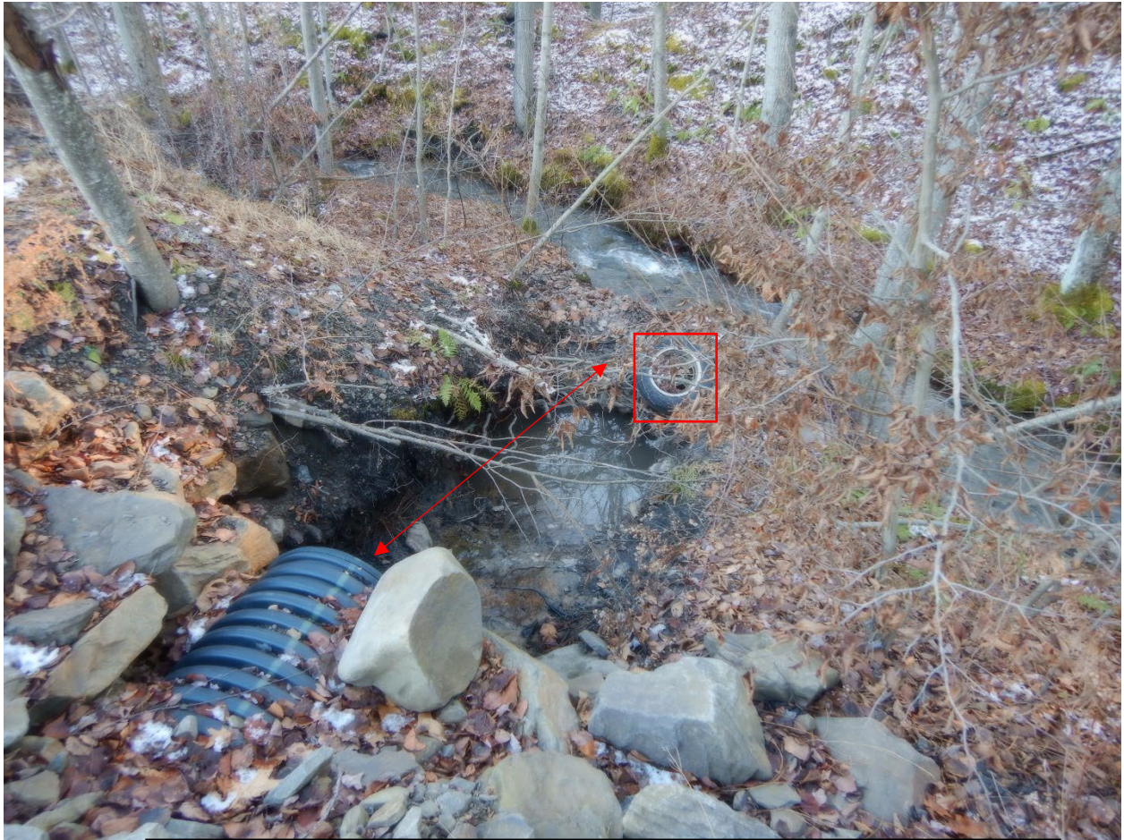
DSCN4059 Meredith Creek – About 40 ft south, across from the entrance to facility yard (Note tire displaced (red box) into stream and erosion on banks upstream westwards surrounding pipe (red arrow))
