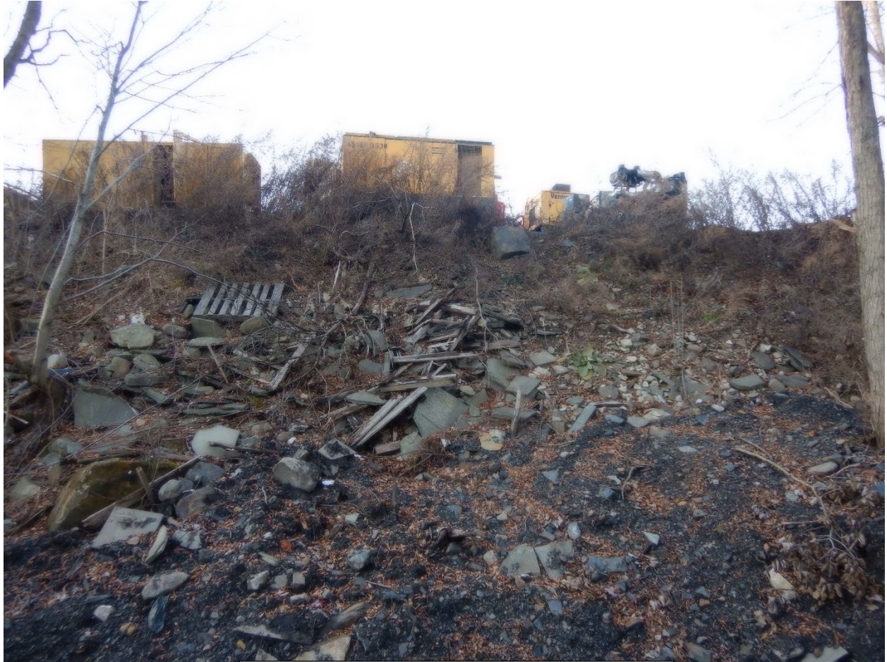
DSCN4063 Edge of east boundary of facility approximately 50ft west of Main street and 20ft north of driveway – Note debris scattering downslope.
